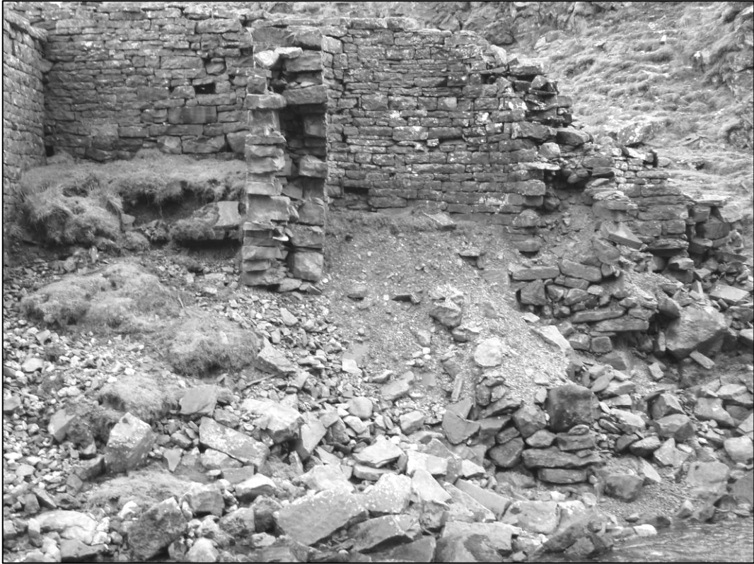
Plate 11: Eroding wall between bins B86/4 and B86/5, Sir George Level Bouse teams, looking E, December 2009 (photo 1/718).
