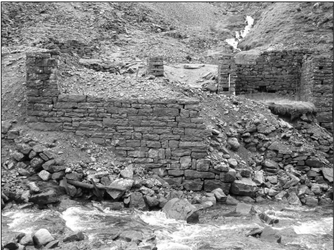
Plate 12: Revetment wall B85, Sir George Level bouse teams, looking E, December 2009 (photo 1/712).
