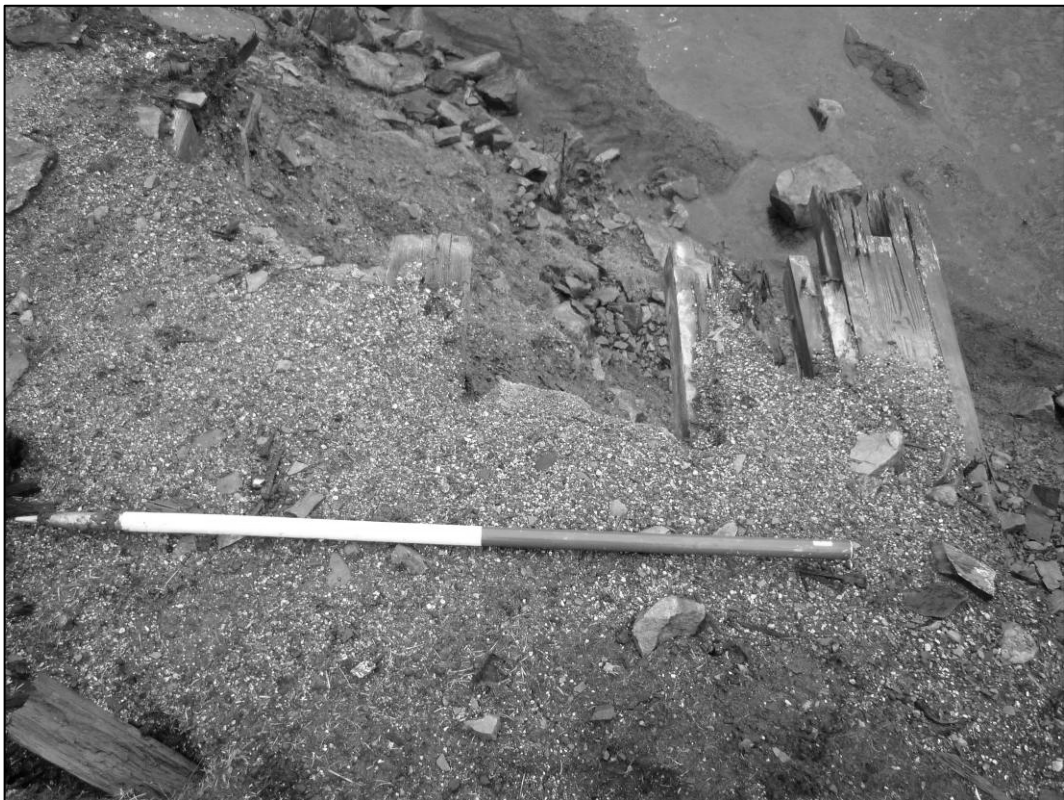
Plate 6: Eroding timber structure, Sir Francis Mine dressing floor, looking E, December 2009 (photo 2/785).
