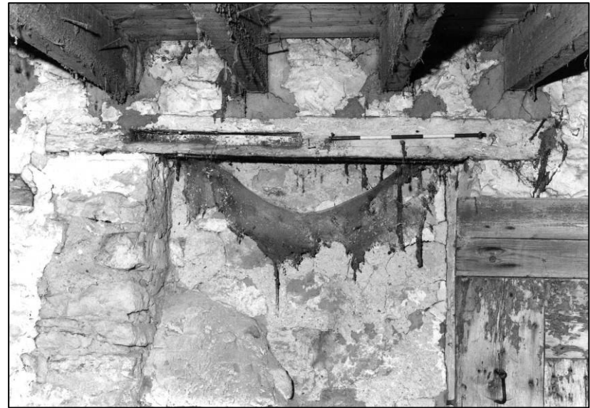
Plate 16: Granary: GF S cell, re-used timber to lintel of window, looking SW (photo 1/6).
