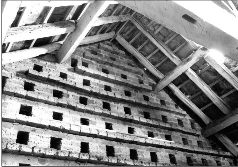
Plate 53: Granary: 2F pigeon loft, upper part of N wall, looking NE (photo 4/6).
