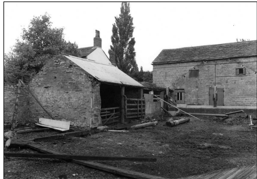
Plate 92: Workshop and recent shed to SW of barn, after demolition of adjoining shed, looking W (photo 9/4).
