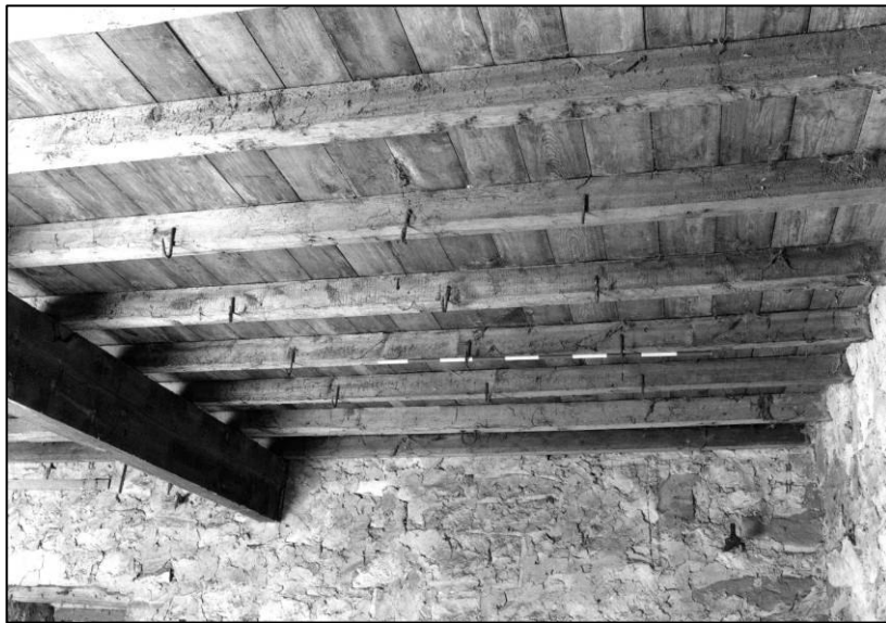
Plate 39: Granary: N bay of 1F N cell, ceiling hooks to joists, looking NW (photo 3/4).
