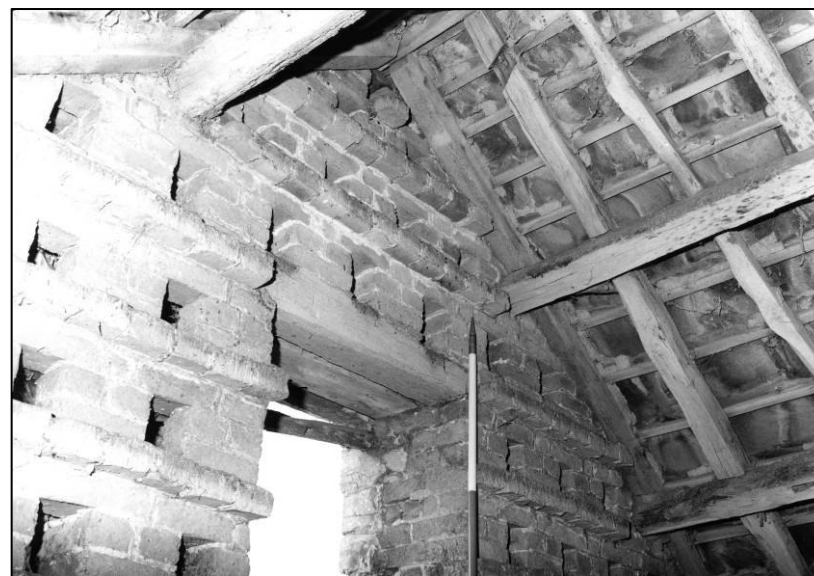
Plate 48: Granary: 2F pigeon loft, upper part of S wall, looking W (photo 4/11).
