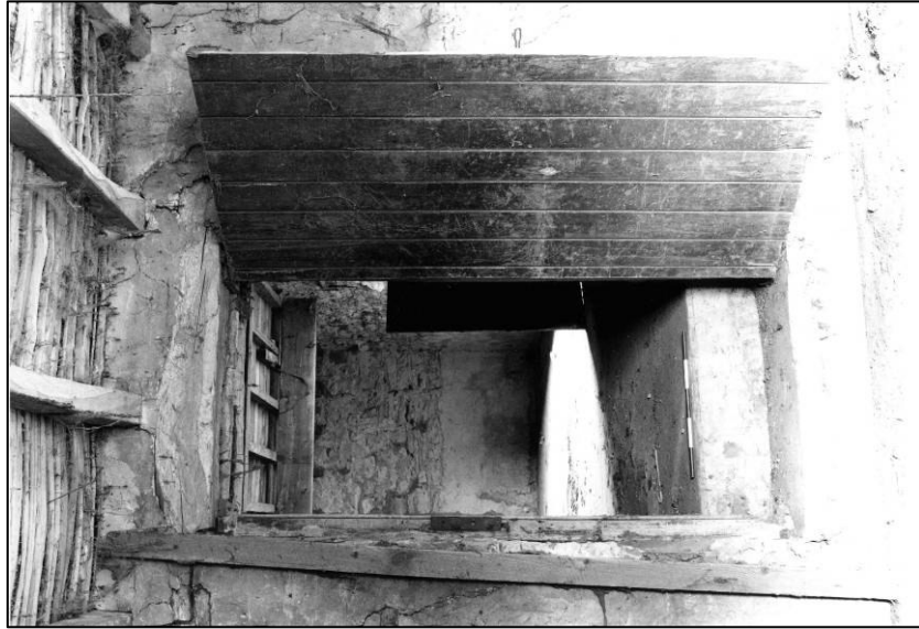
Plate 33: Granary: 1F S cell, doorway to N cell, looking NE (photo 2/17) (top to left).
