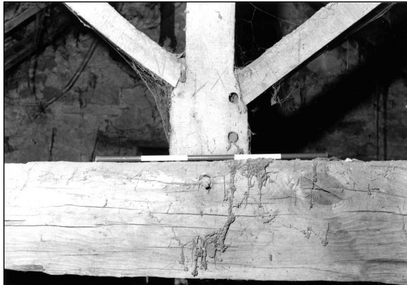
Plate 59: Granary: 2F N cell, base of king post to S face of N truss, looking NE (photo 3/15).
