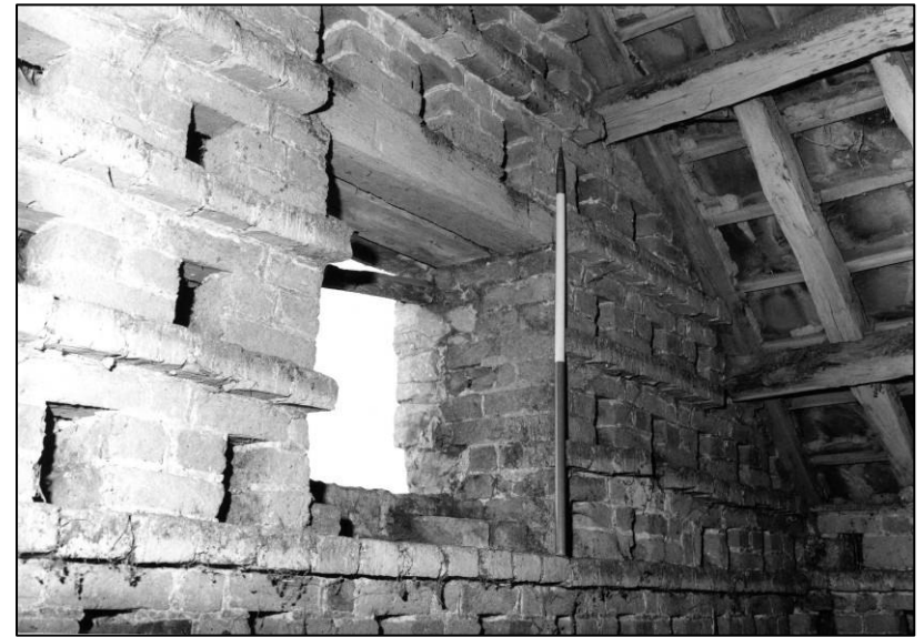
Plate 40: Granary: 2F pigeon loft, upper part of S wall, looking W (photo 4/12).
