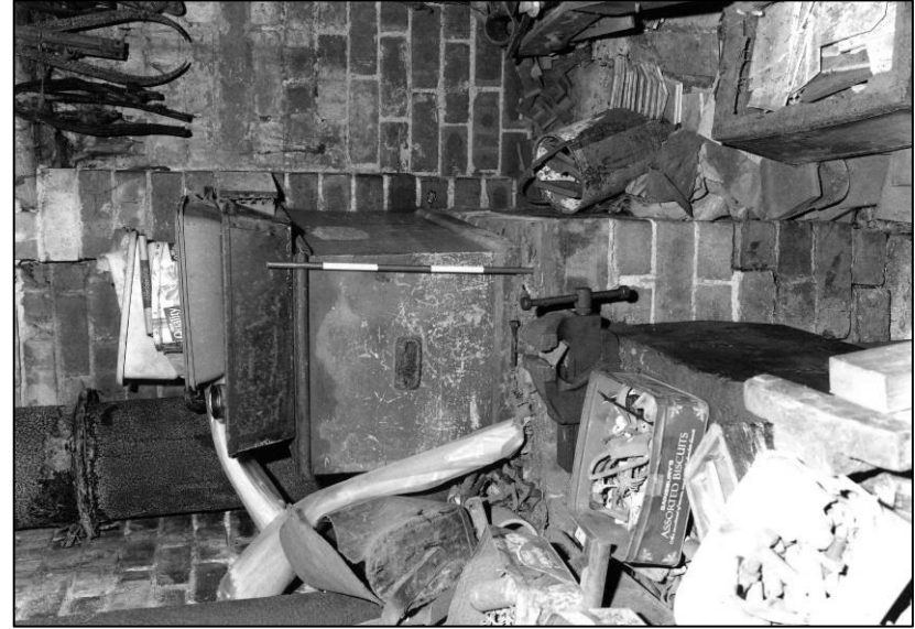
Plate 98: Workshop: interior of S cell and boiler, looking S (photo 5/13) (top to left).
