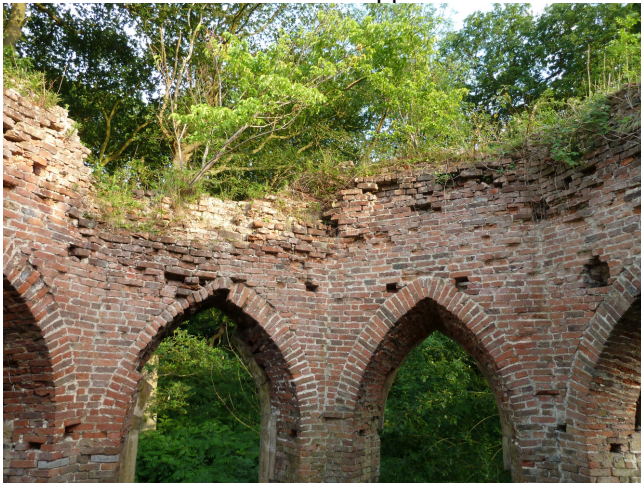
Plate 4 Occasional crevices suitable for bat entrances into potential bat roosts were also recorded in the upper levels of the building
