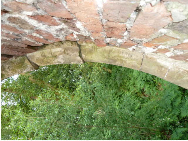
Plate 3 Occasional crevices suitable for bat entrances into potential bat roosts were also recorded between the stonework at the apex of some of the arches
