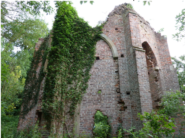
Plate 5 Dense ivy covered parts of the external elevations of the fireplace making the brickwork inaccessible for inspection
