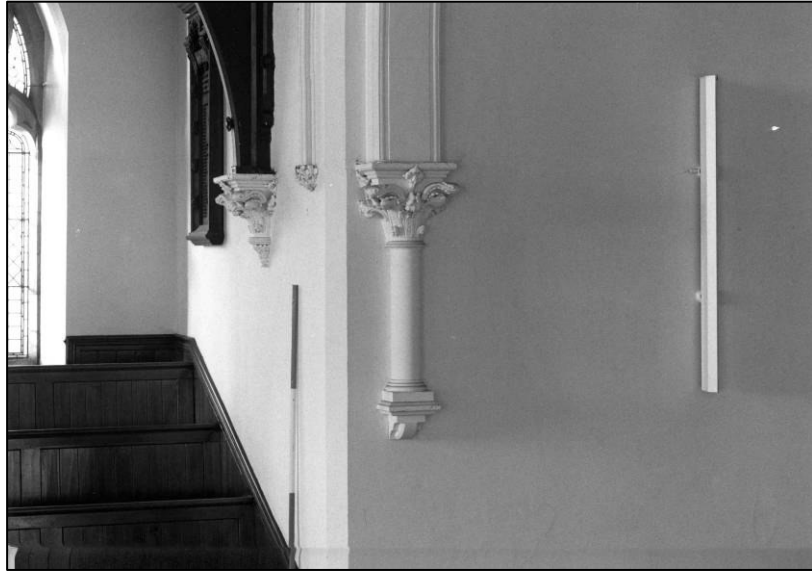
Plate 93: Church: 1F gallery, typical corbels to N end (W side), looking NW (photo 4/5).
