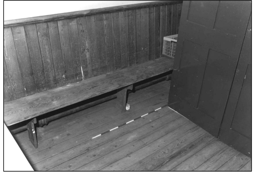
Plate 146: School: GF, typical side room off main hall (S side), looking SW (photo 12/17).
