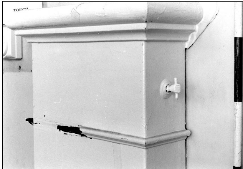
Plate 143: School: GF main hall, S side, hand control to heating, looking SE (photo 11/13).
