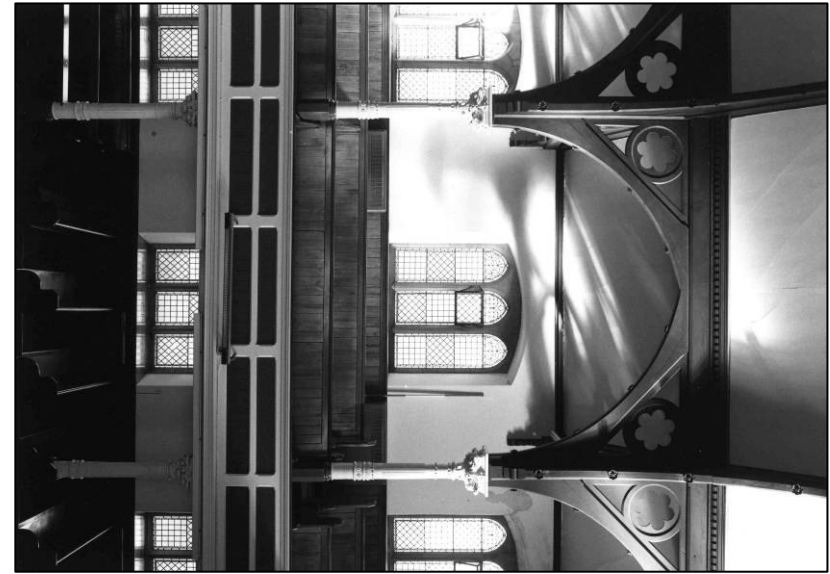
Plate 100: Church: 1F gallery, typical bay (W side), looking W (photo 4/16) (top to right).
