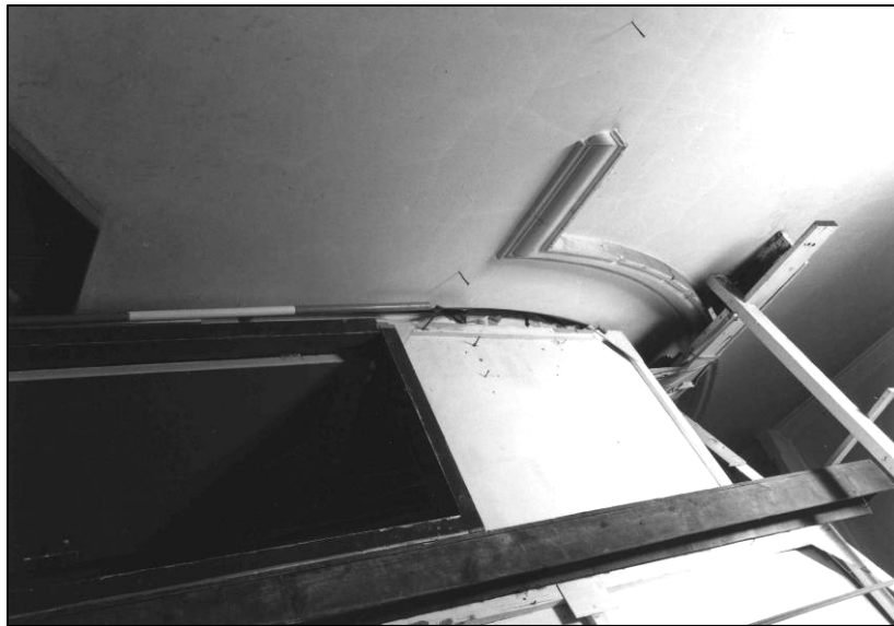
Plate 139: School: GF main hall, original proscenium arch to stage at W end, looking NW (photo 11/16) (top to right).
