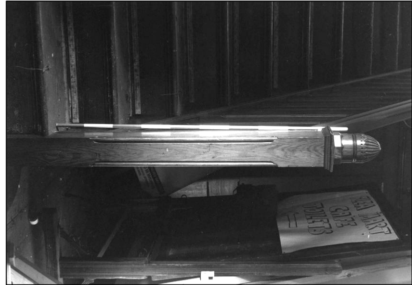
Plate 38: Church: GF entrance foyer, W stair newel post, looking W (photo 1/12) (top to right).
