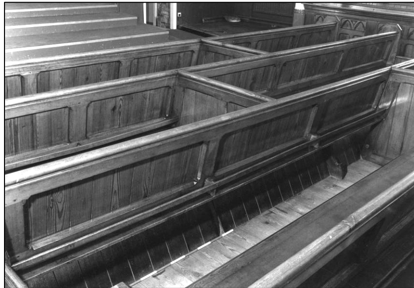
Plate 55: Church: GF, typical nave pews showing foot rests etc, looking NE (photo 2/12).
