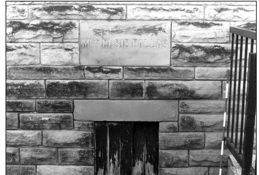
Plate 112: School: 'Fallas' foundation stone, S elevation of main hall, looking N (photo 13/9).
