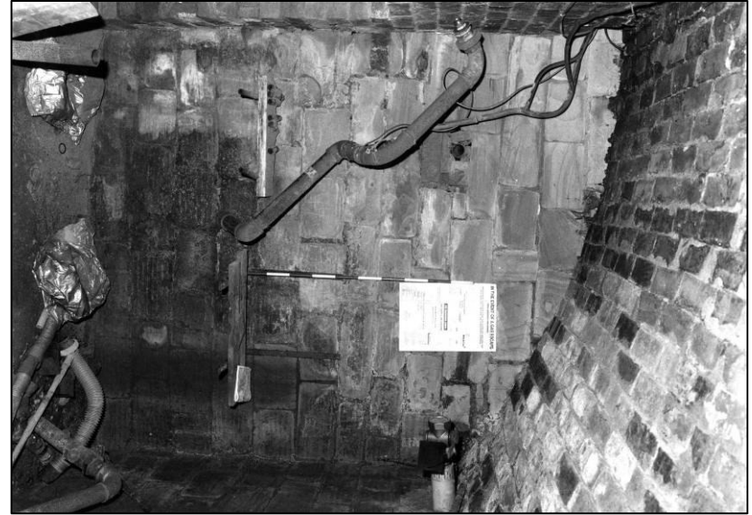
Plate 22: Church: heating basement beneath N end, looking S (photo 9/7) (top to right).
