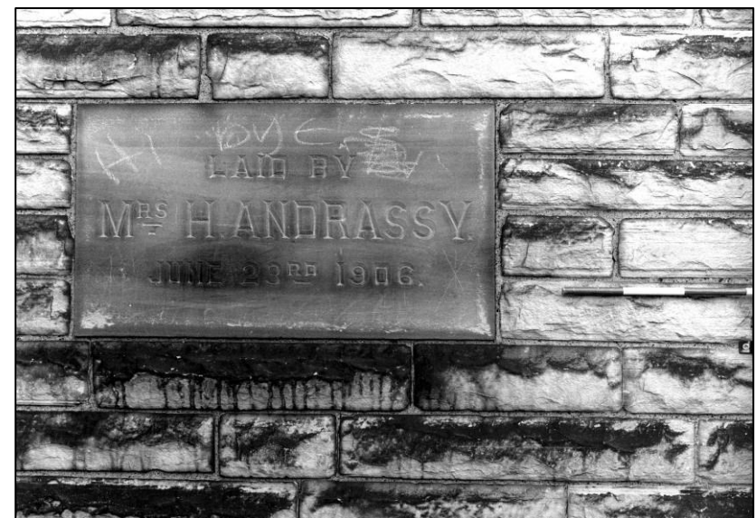
Plate 116: School: 'Andrassy' foundation stone, W elevation of band room, looking E (photo 13/14).
