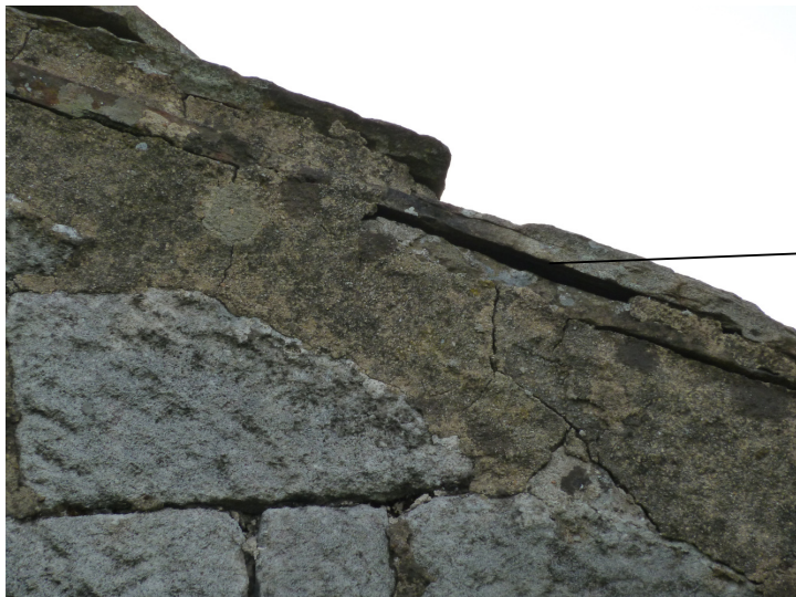
Plate 4 East elevation (north room): small hole for bat entry into a potential bat roost just below the roof
