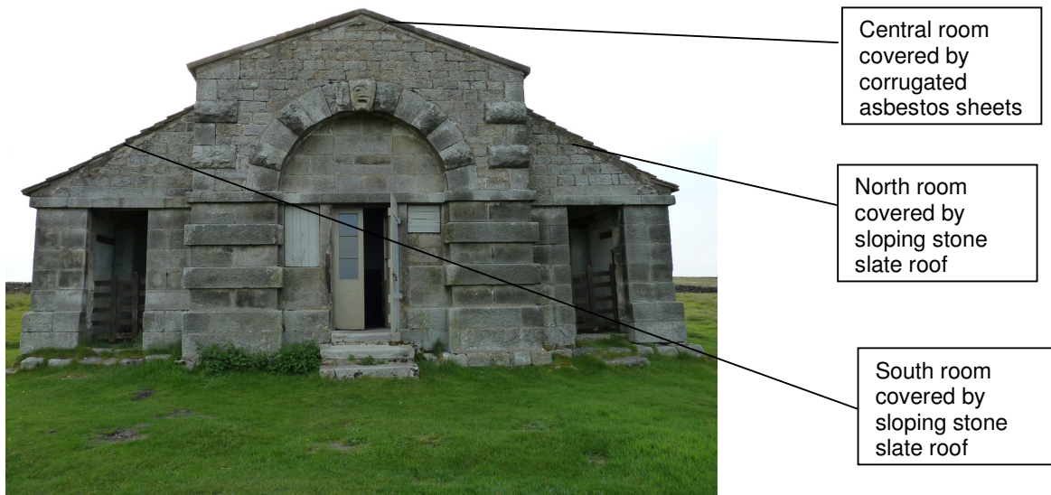
Plate 2 South elevation: gaps suitable for bat entry into potential roosts between overlapping stone slates
