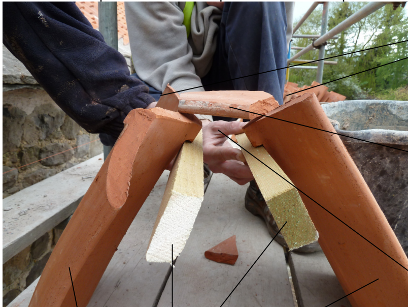
Plate 11 Example: the creation of potential bat roost spaces under ridge tiles (cross-section)
