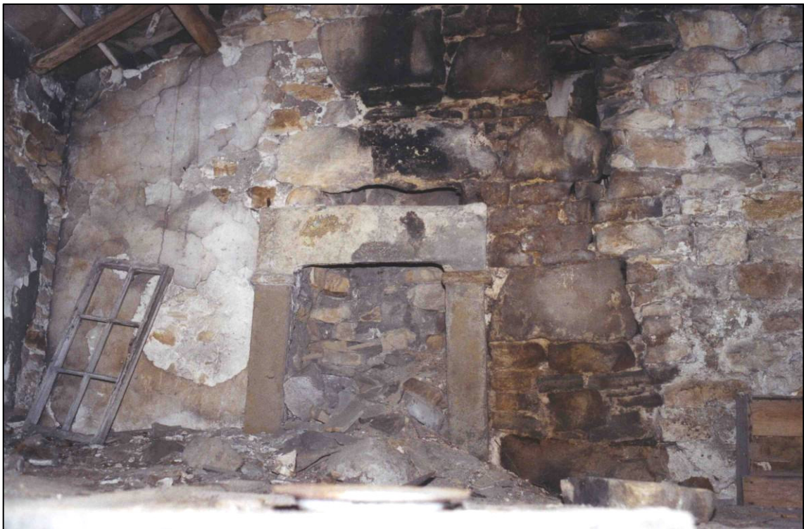
Plate 5: Fireplace in north end of central part of west range (first floor), looking S.
