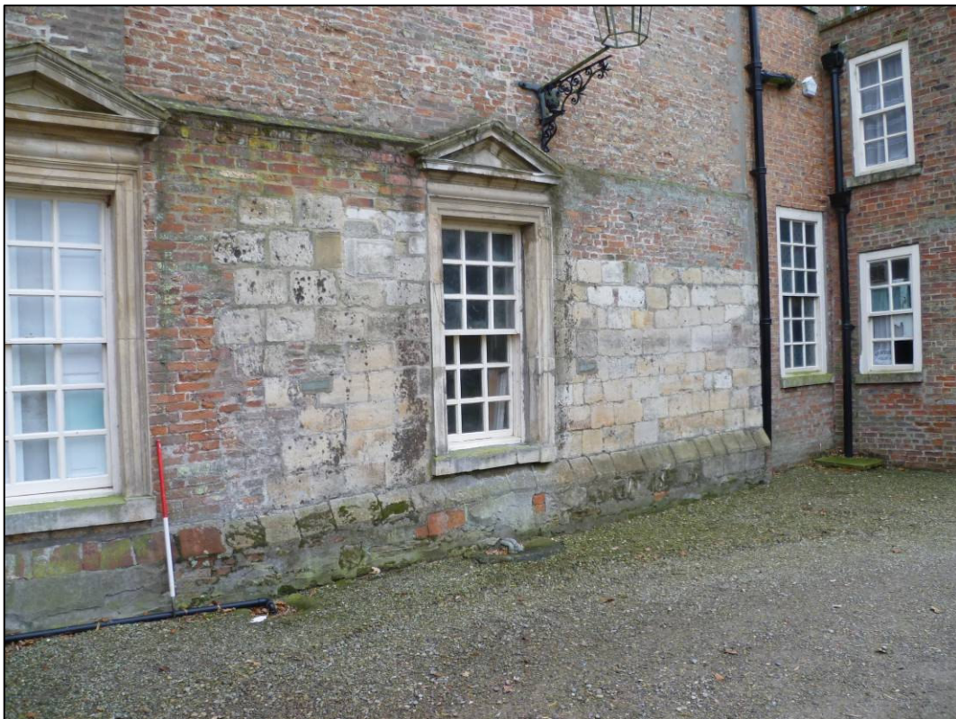
Plate 14: Base of north elevation of north tower of Burton Constable Hall, showing potentially early stonework.
