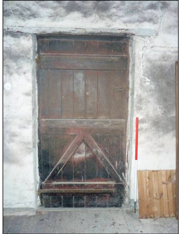
Plate 9: West doorway in first floor east cell, granary/cart shed range, looking W (photo 1/71).
