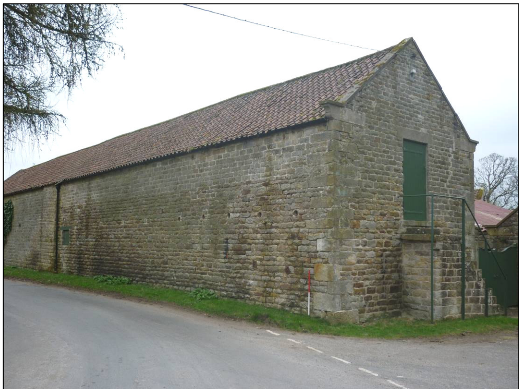
Plate 5: North elevation and west gable of granary and cart shed range, looking SE (photo1/18).
