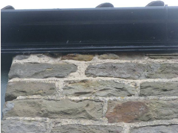
Plate 2 The Granary (south elevation) – bats recorded in the crevices between the fascia board and stone wall
