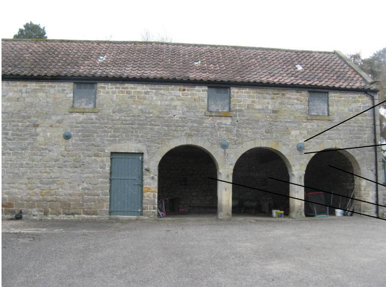
Plate 3 The Granary (south elevation) – bats recorded in, and emerging from the stone walls and under the arches
