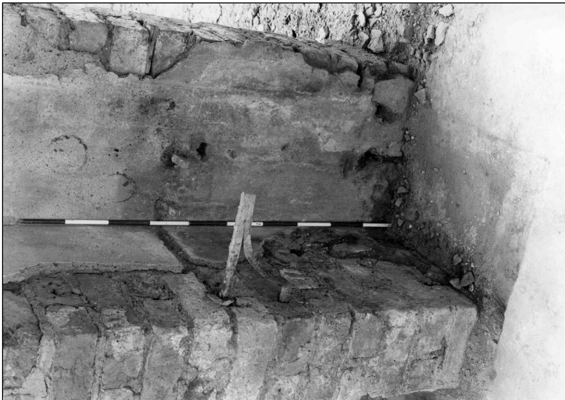
Plate 36: Brackets to west of fireplace, south wall of central room, looking SE (photo 2/18) (top to left).
