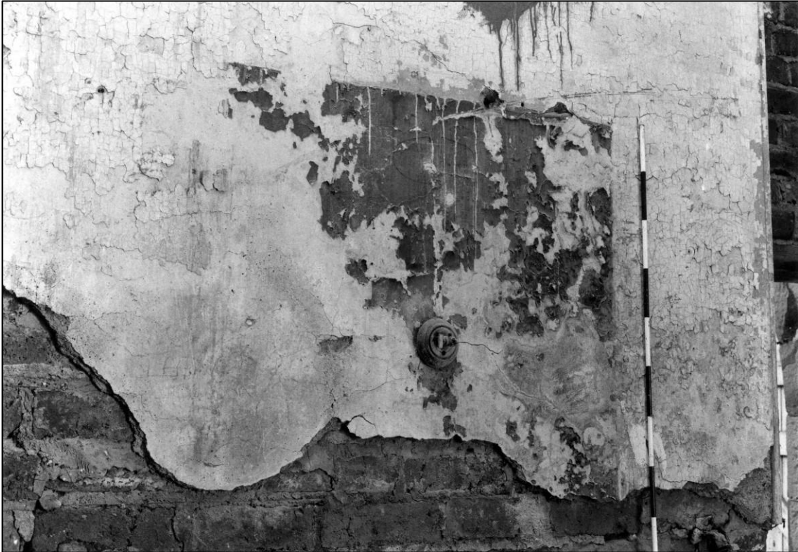
Plate 35: Gas mantle and paint on south wall of central room, looking S (photo 2/17).
