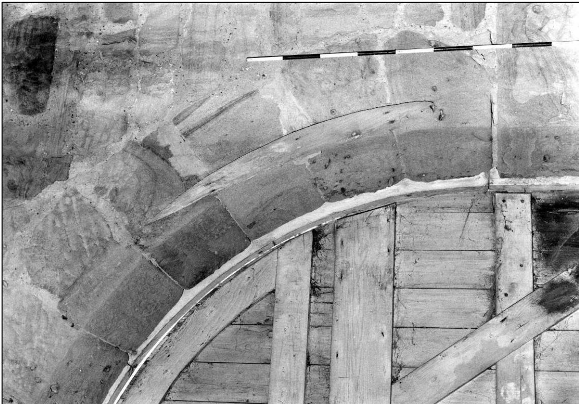
Plate 46: Former timber lining of south coach opening, west wall of south room, looking W (photo 1/15) (top to left).
