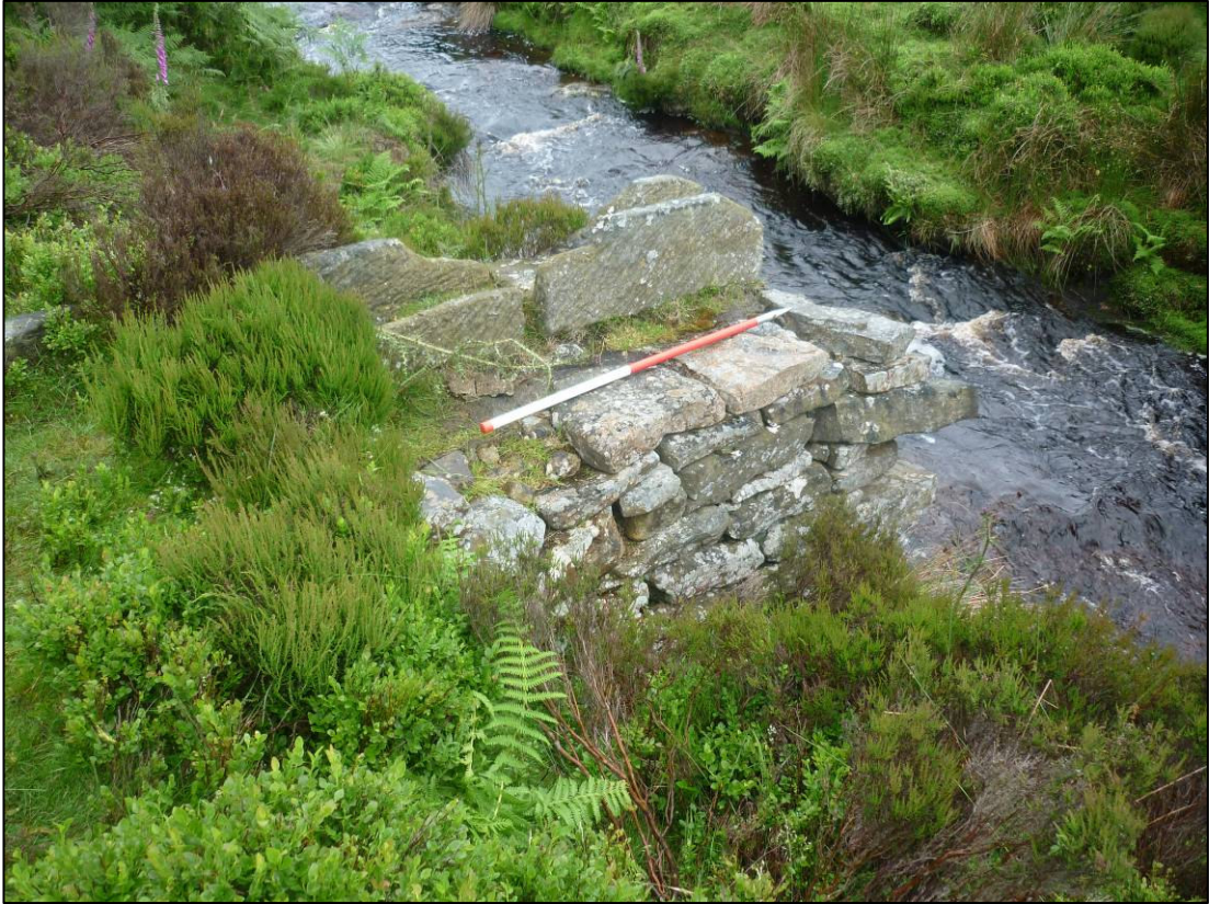
Plate 4: Collapsing west pier, looking NE (photo 1/650).
