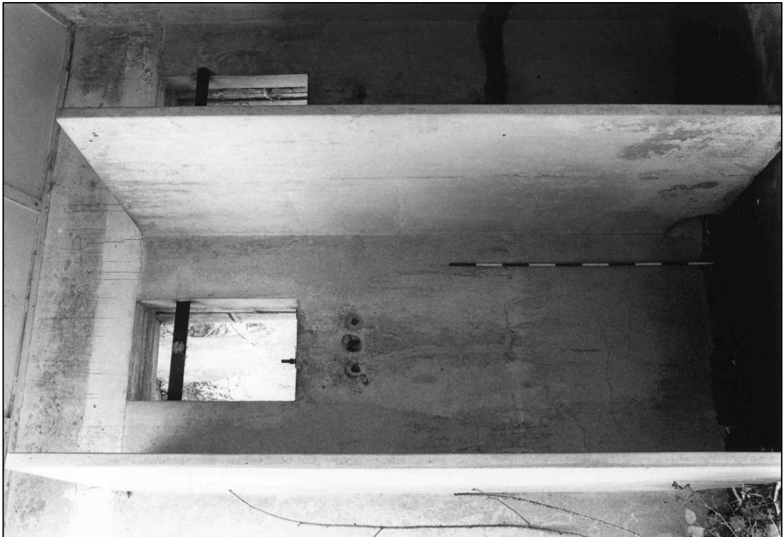
Plate 82: Building S5, typical appearance of showers, looking SW (photo 3/9) (top to left).
