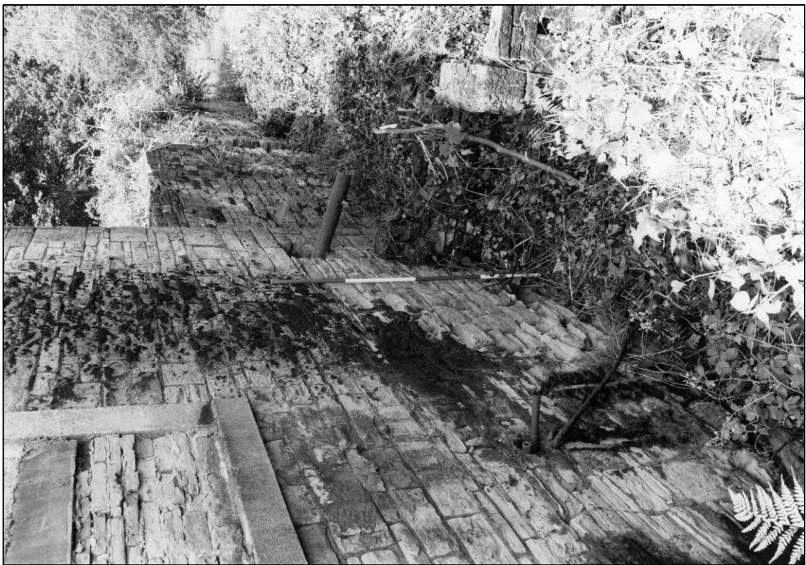
Plate 28: Building N2, base of east gable, looking NW (photo 6/4) (top to left).
