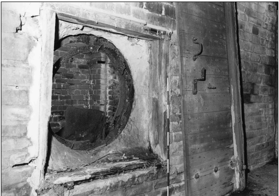
Plate 60: Building N4, opening in north wall of fan passage to Building N3, looking NE (photo 4/10).
