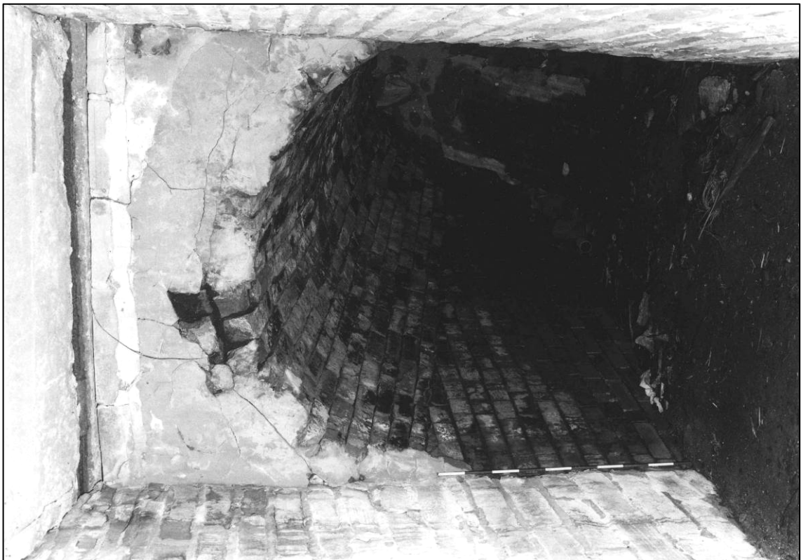
Plate 62: Building N4, entrance to fan drift, looking W (photo 4/5) (top to left).
