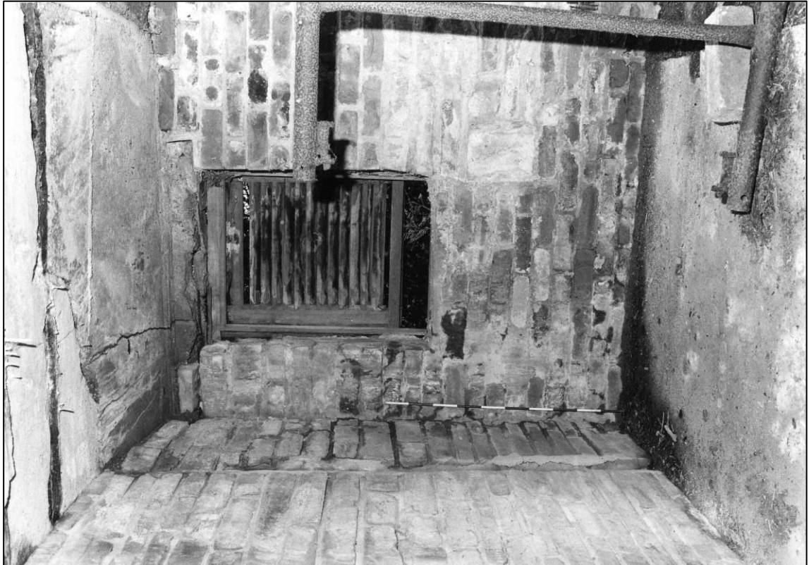
Plate 55: Building N4, interior of fan passage, east end, looking E (photo 4/15) (top to left)
