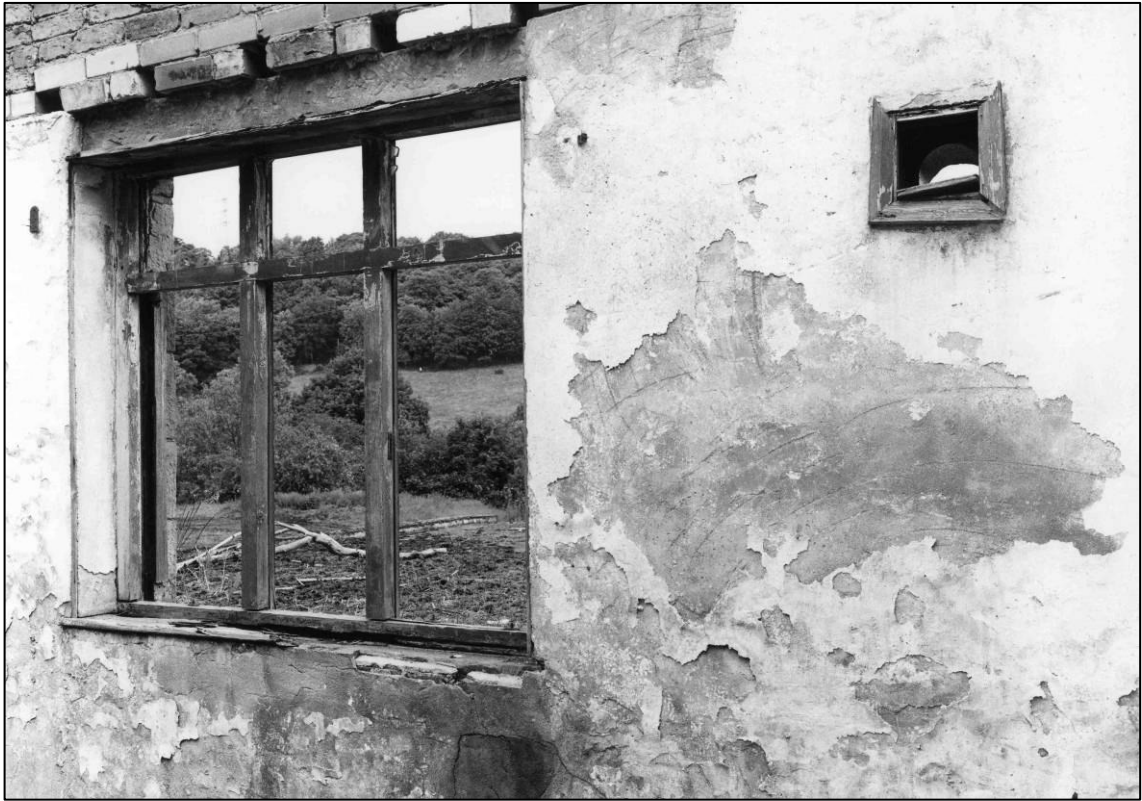
Plate 87: Building S1, first floor interior, north wall showing vent, looking N (photo 3/4).
