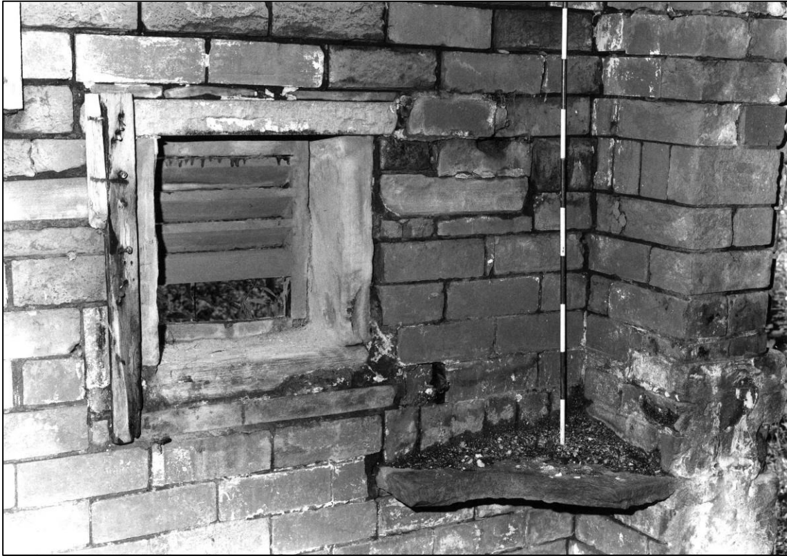
Plate 15: Building N1, central cell, vent and shelf to north wall, looking NE (photo 2/5).
