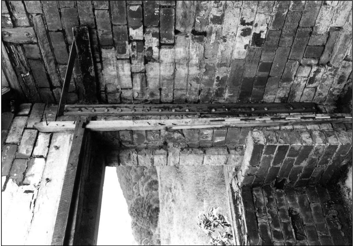
Plate 13: Building N1, interior west cell, former tallies to W wall, looking NW (photo 1/16) (top to left).
