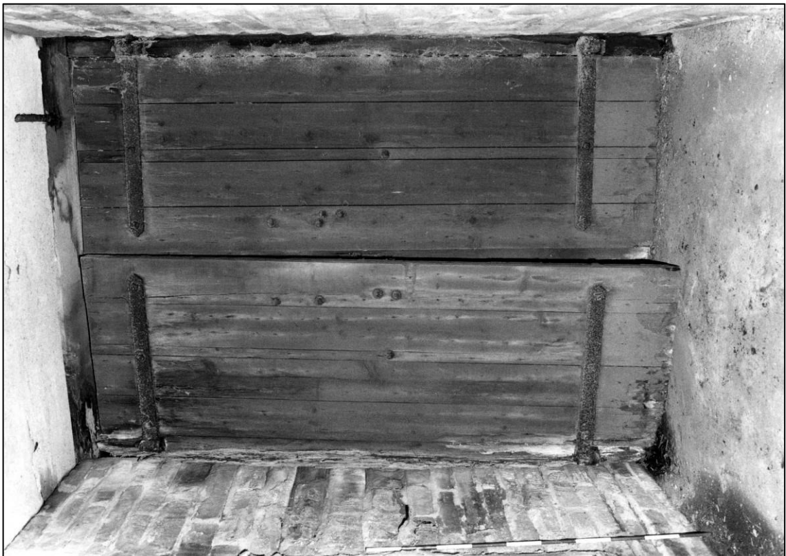
Plate 58: Building N4, fan passage, west door face, looking E (photo 4/11) (top to left).
