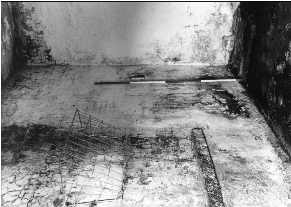
Plate 72: Building S2, south wall of south cell, looking SW (photo 4/17) (top to left).
