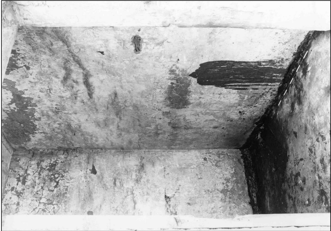
Plate 71: Building S2, typical interior of one of north cells, looking SW (photo 3/5) (top to left).
