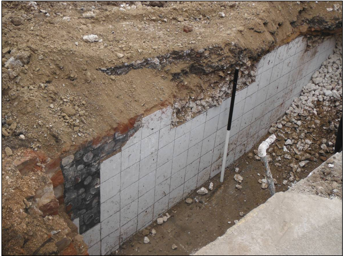
Plate 3: White tiled brick wall (116) of concrete-floored passage, in north side of south foundation trench, looking NE.
