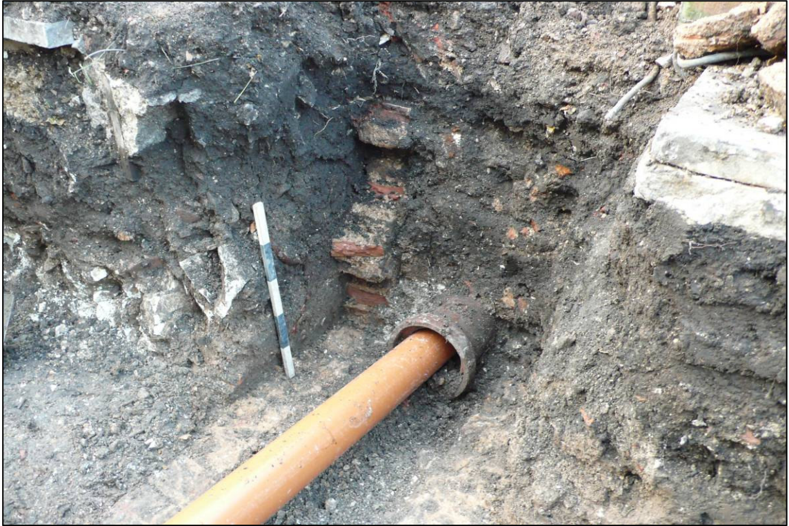
Plate 16: Sewer pipe (052) cut through centre of brick wall (051) leaving outer skins intact, looking SW.
