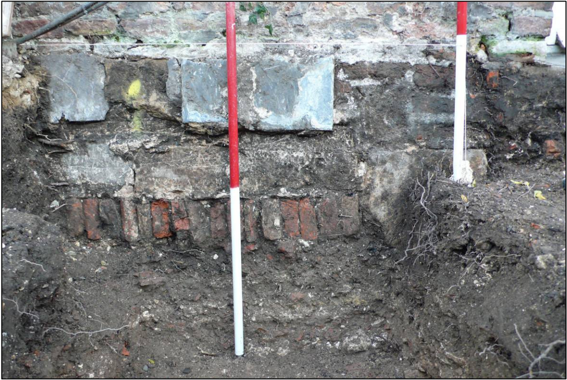
Plate 9: Foundations for gable of Lambert's c.1700 rear wing comprising dressed stone and brick on edge (023) on brown soil (033), looking E.
