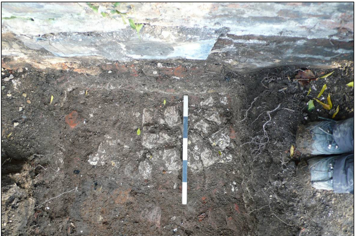
Plate 17: Chalk wall foundation (036) under gable of Lambert's c.1700 rear wing, from above.
