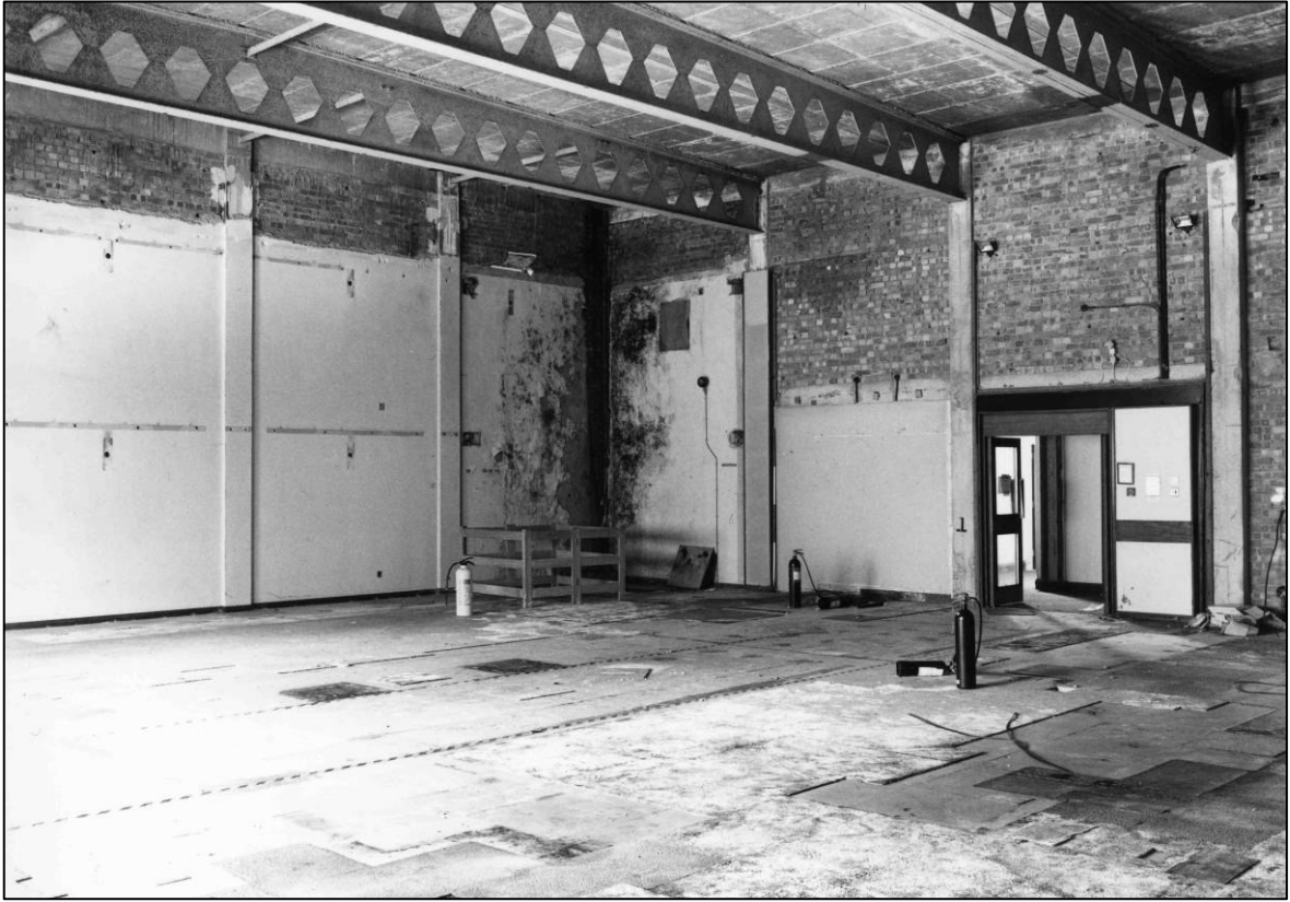
Plate 115: Interim Control Room (1F25), looking E (photo 3/4).
