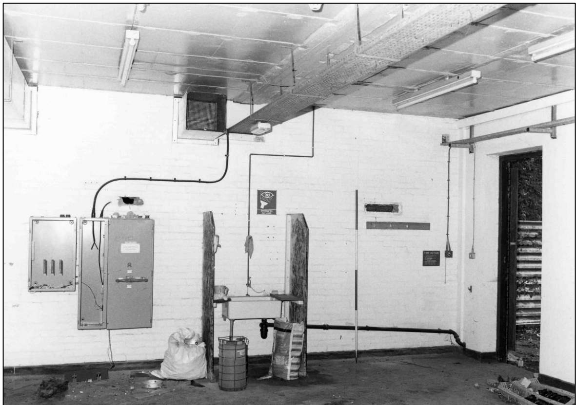
Plate 60: UPS Battery Room (GF17), looking SE (photo 9/9).
