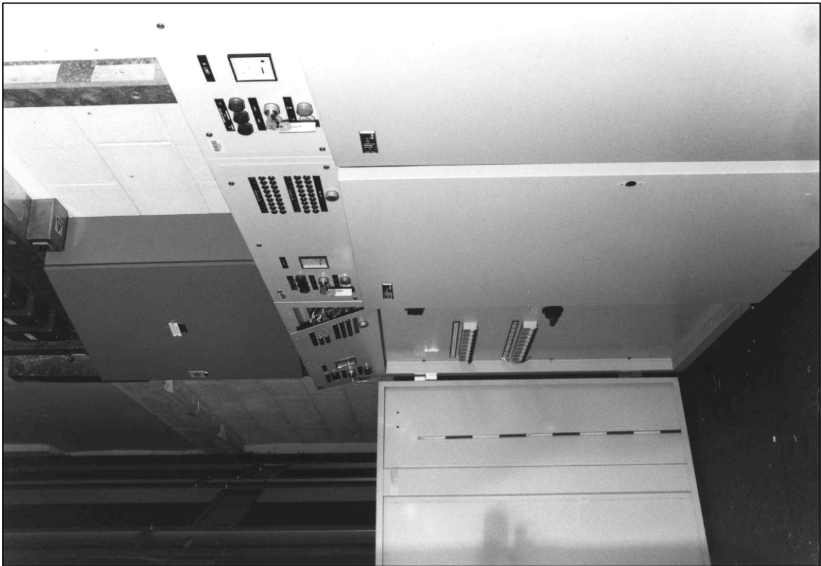
Plate 99: Control room (1F15), control panels on W side, looking S (photo 2/9) (top to left).
