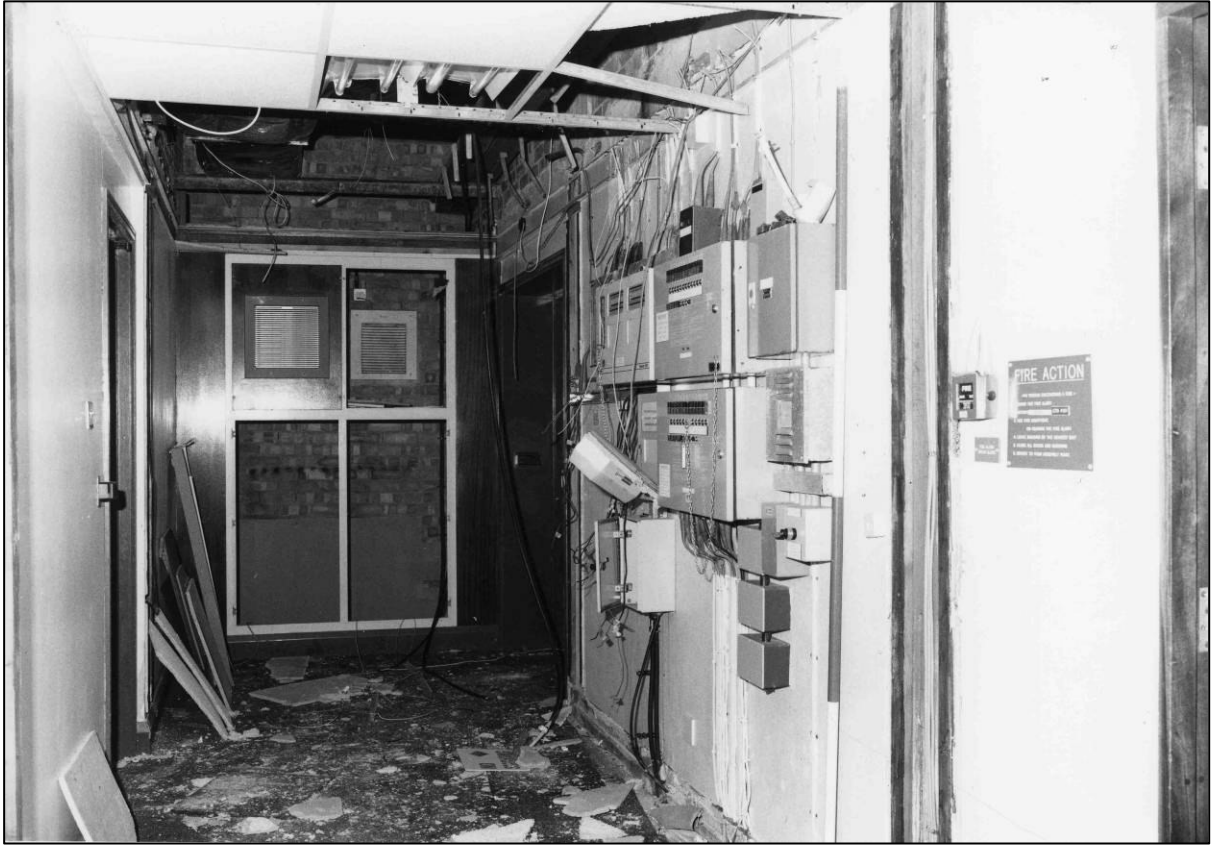
Plate 107: Corridor 1F19, fire alarm panels, looking NW (photo 2/17).
