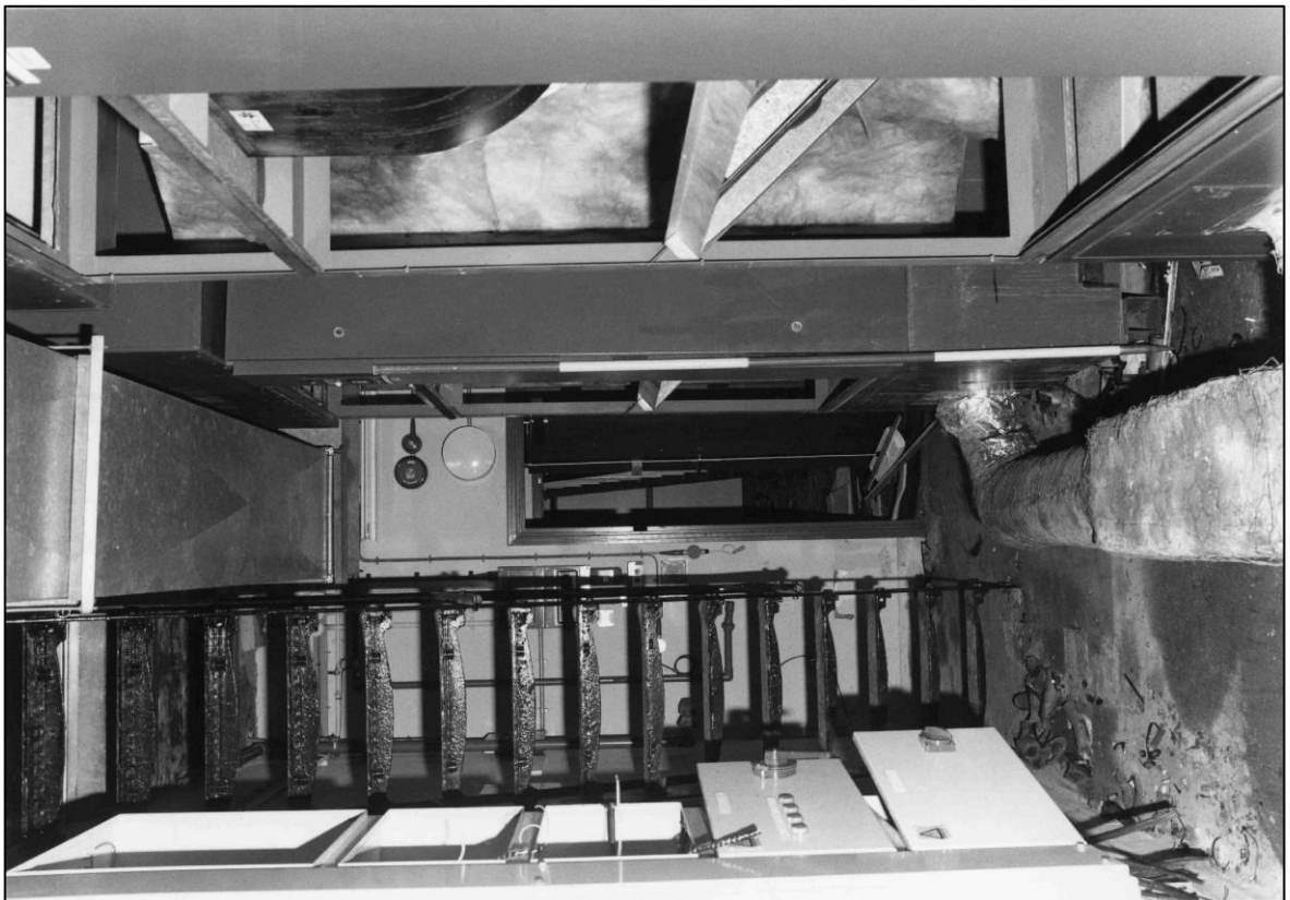
Plate 58: EBU Plant Room (GF21), looking NW (photo 5/3) (top to left).
