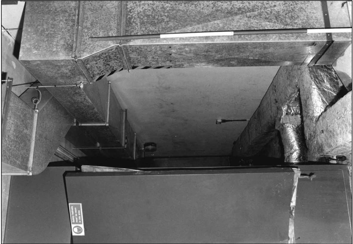
Plate 57: EMS/FSA Plant Room (GF15), looking SE (photo 5/1) (top to left).
