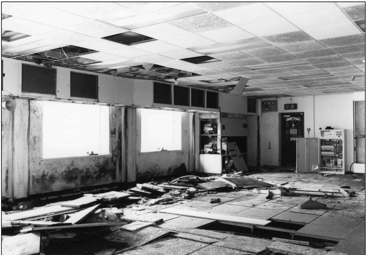
Plate 68: Apparatus Room 2B (GF31), looking NE (photo 5/8).
