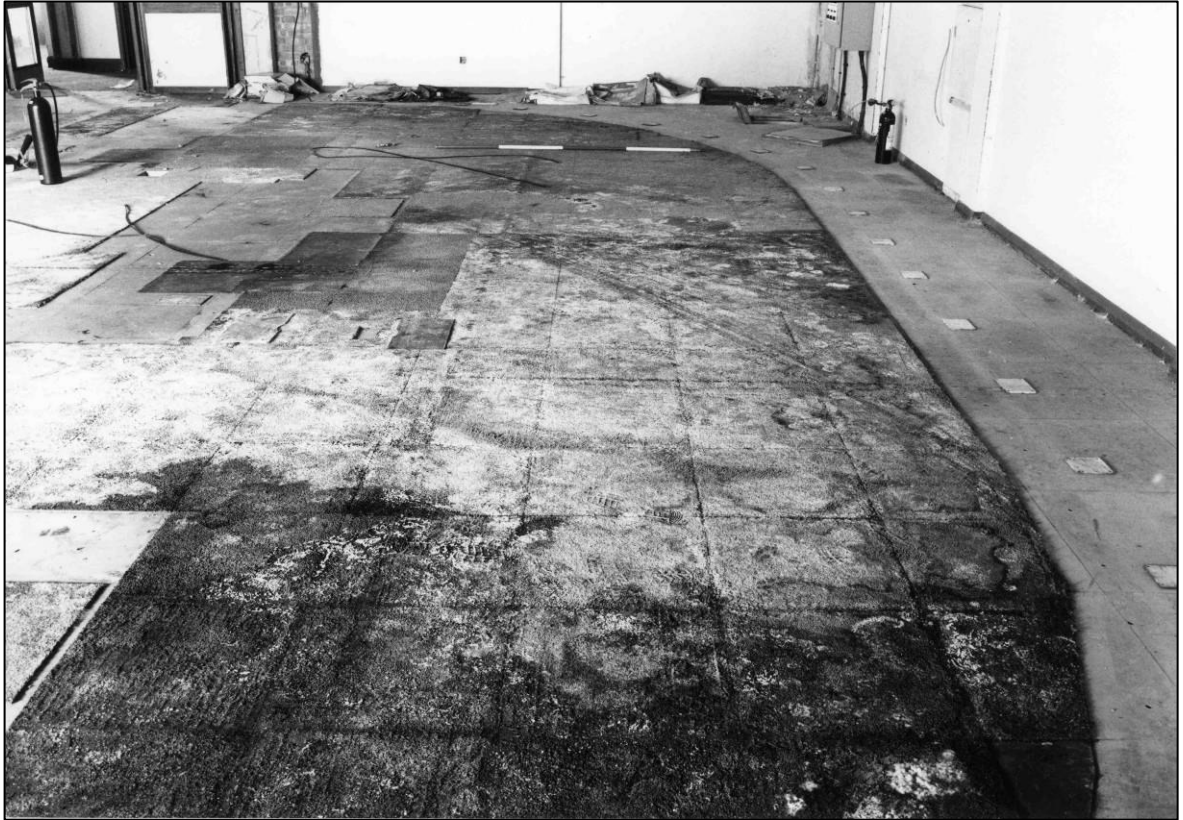
Plate 109: Interim Control Room (1F25), curve of former structure to W side, looking SW (photo 3/10).
