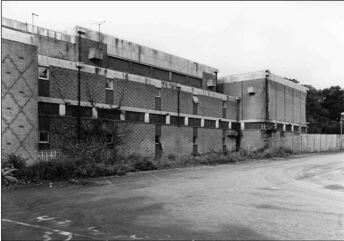
Plate 19: Control Centre complex, central part and N end of E elevation, looking W (photo 7/11).
