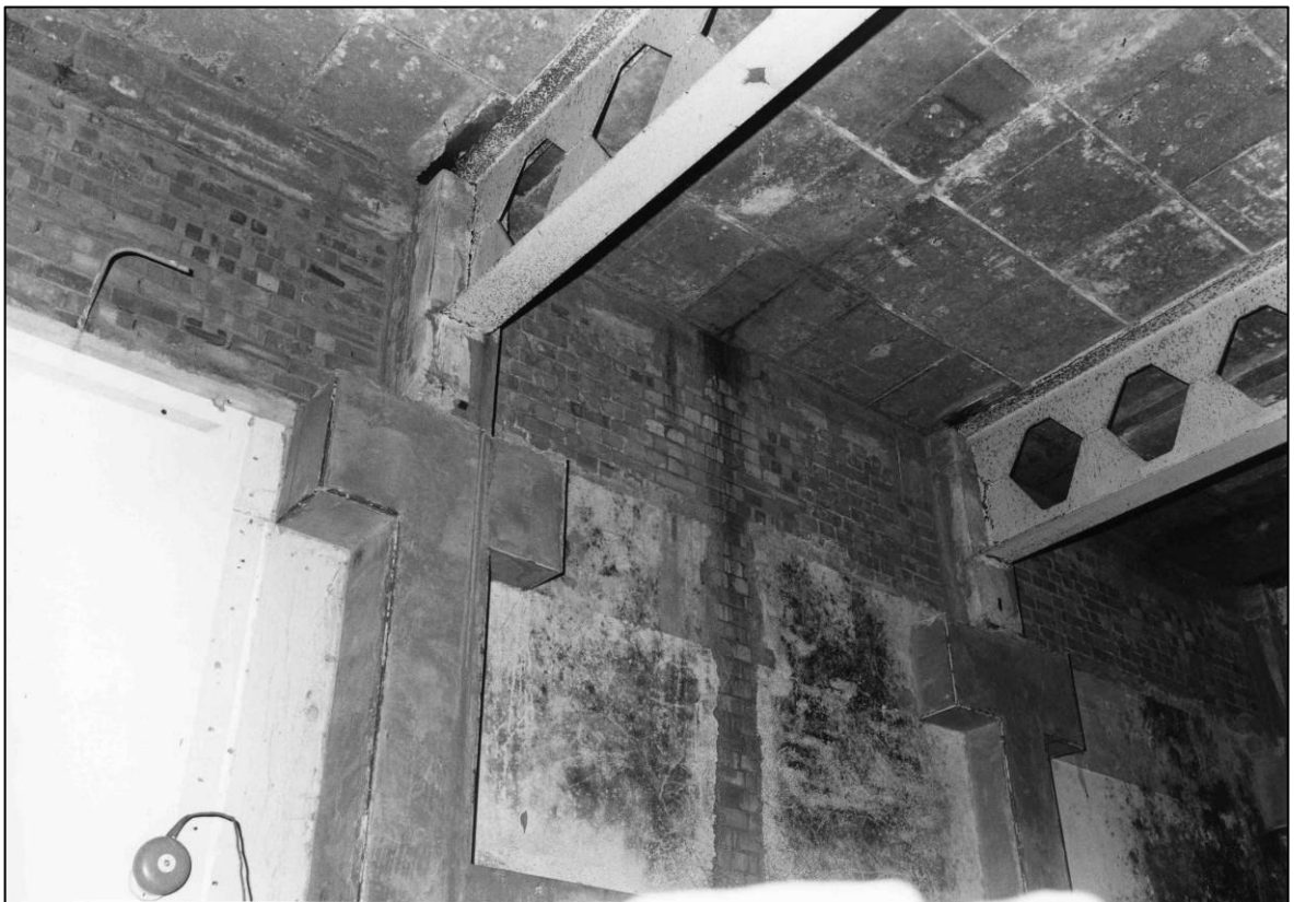
Plate 114: Interim Control Room (1F25), concrete frame and girders to N wall, looking N (photo 3/11).
