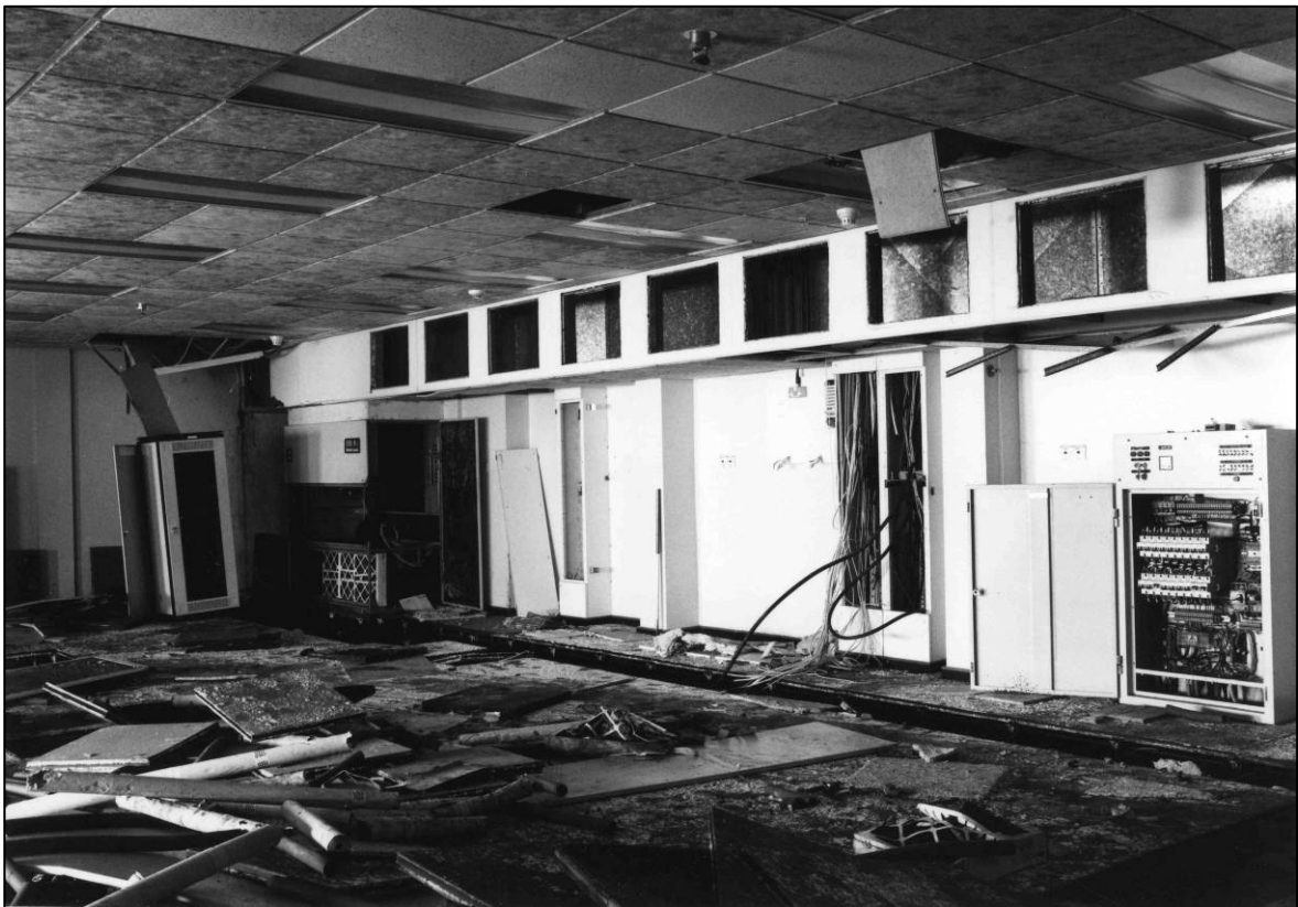
Plate 64: Apparatus Room 2A (GF30), looking E (photo 5/5).
