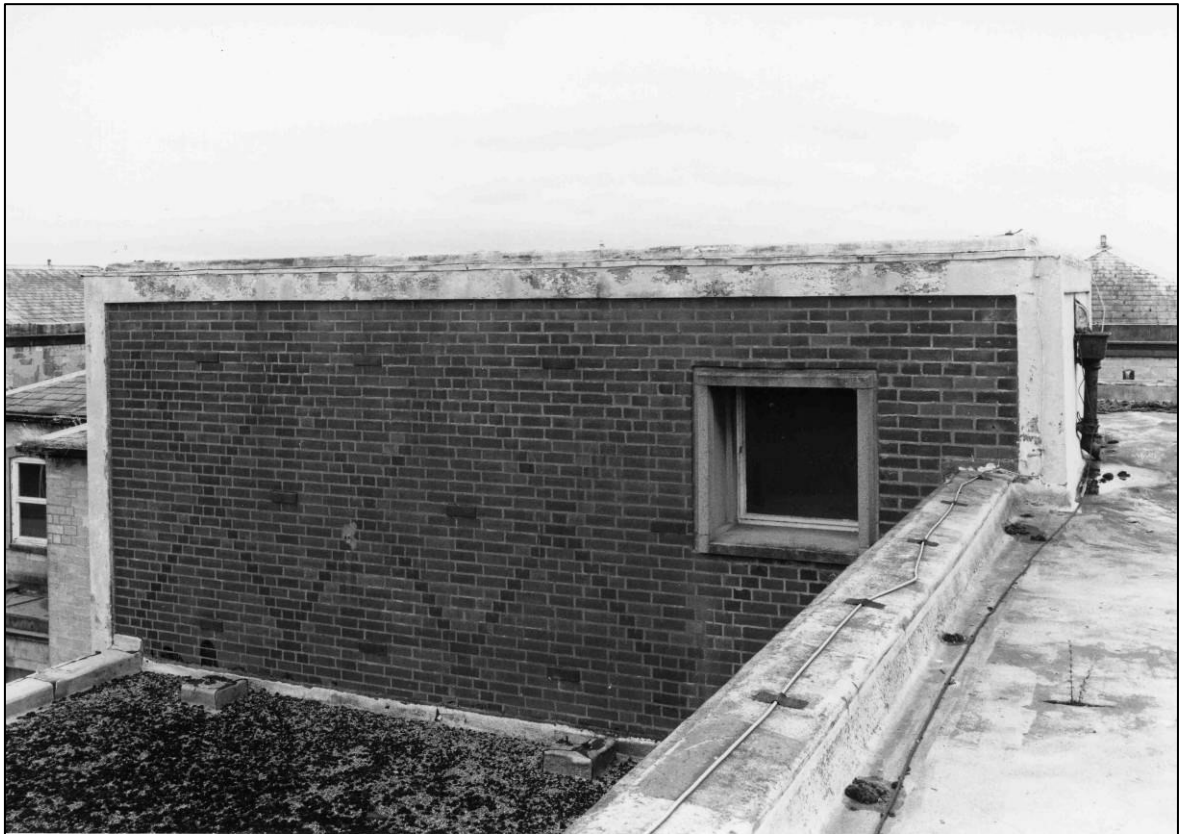
Plate 14: Control Centre complex, uppermost N external elevation of stair tower at S end of E elevation, looking E (photo 9/5).
