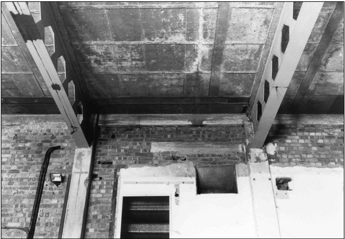
Plate 112: Interim Control Room (1F25), concrete frame and girders to S wall, looking SE (photo 3/12).
