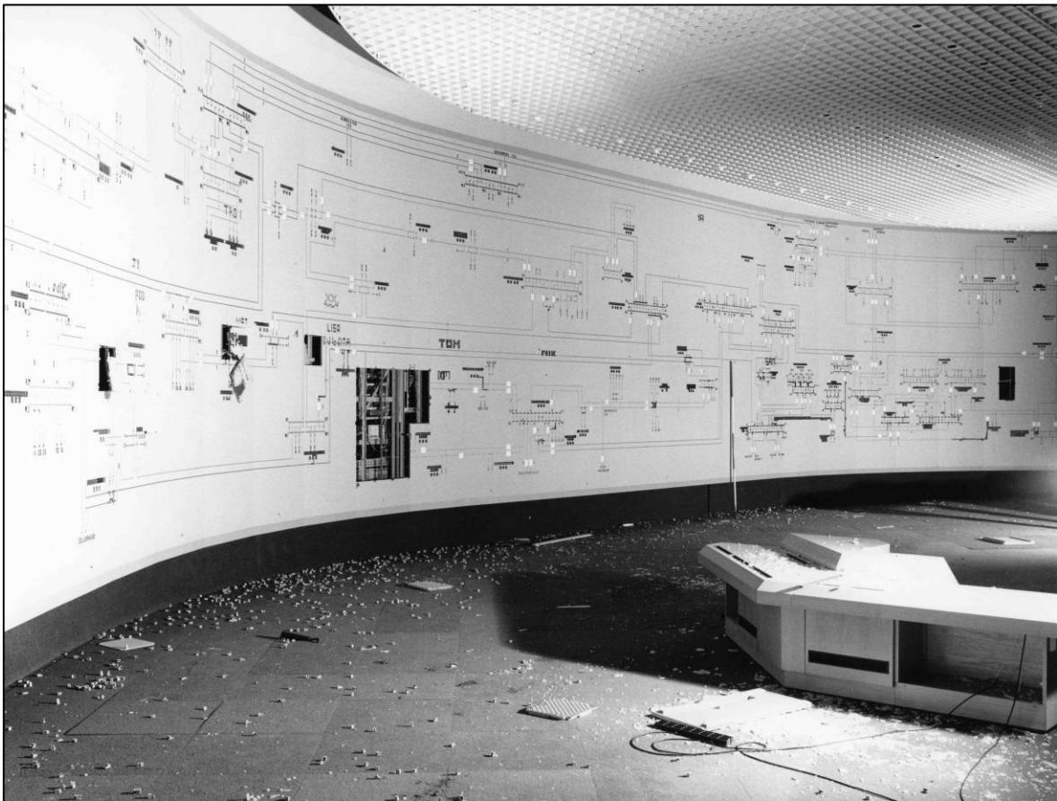
Plate 88: Control room (1F15), general view of mimic board, looking NE (photo 1/1).
