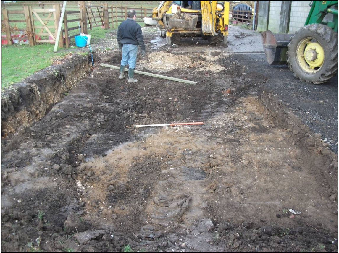
Plate 1: Exposed stratigraphy in main trench after removal of cinder track, looking NW.
