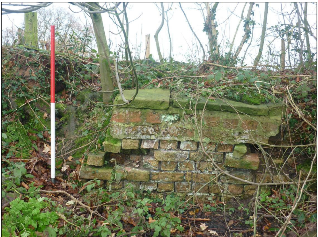
Plate 4: Stone coping and brickwork at north end of east side of the pond, looking E (photo 1/40).
