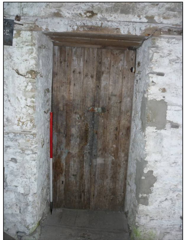
Plate 46: Garage (Site 36b), doorway at east end of north wall (elevation 19) of first floor room 1F12, looking N (photo 7/907).
