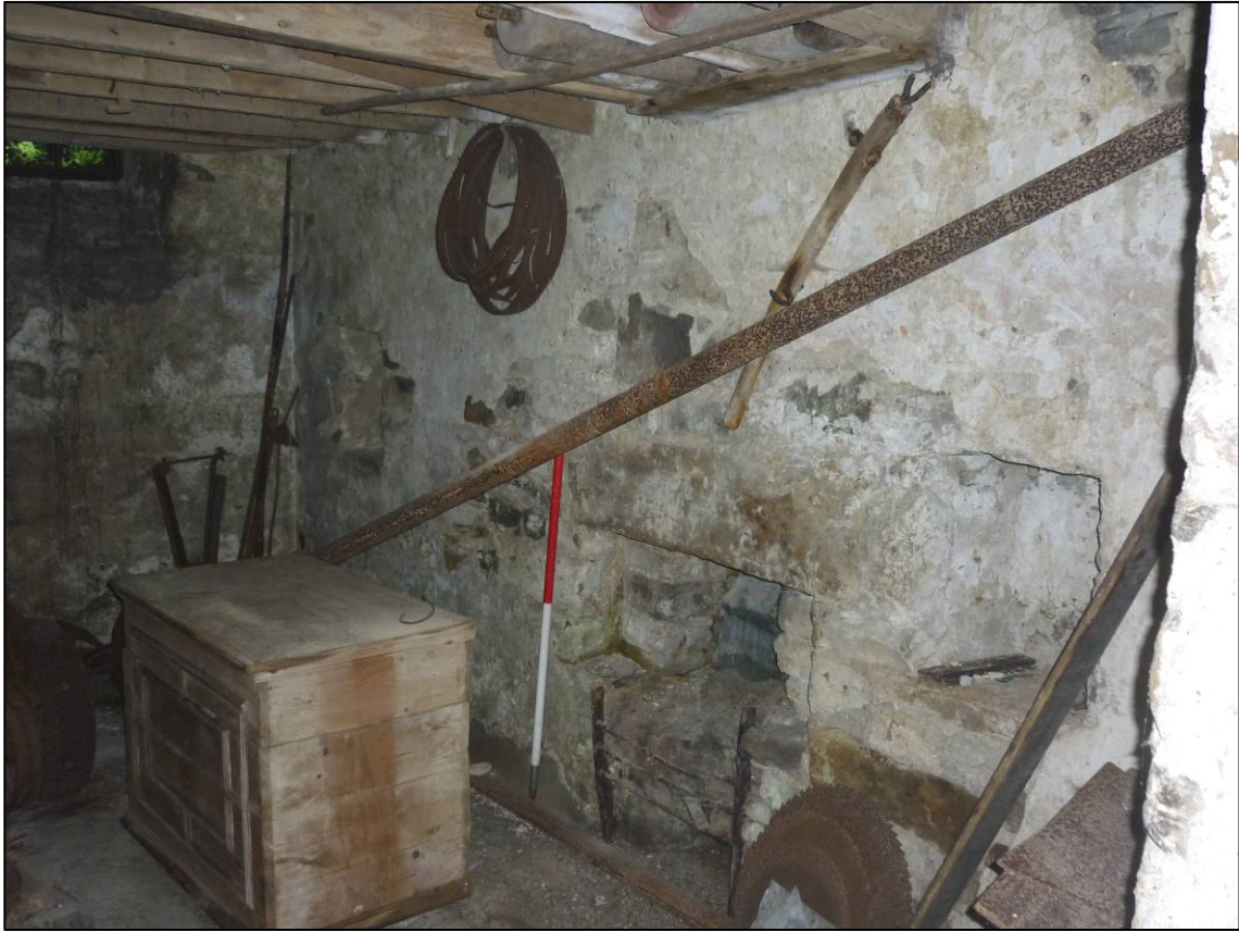
Plate 32: Mill (Site 36a), east wall of ground floor room G4 (elevation 15), looking NE (photo 7/079).
