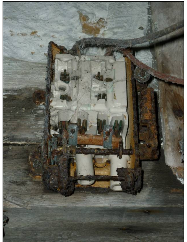
Plate 65: Power house (Site 32), isolator over east doorway, looking E (photo 6/758).
