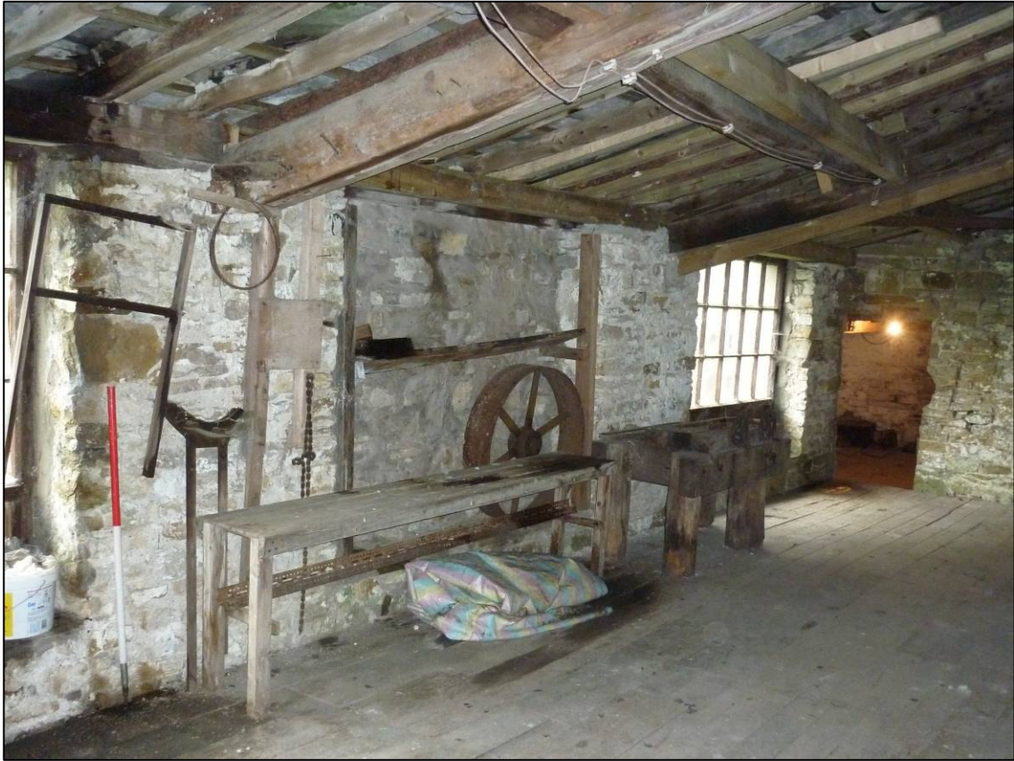
Plate 47: Garage (Site 36b), south wall (elevation 21) of first floor room 1F12, looking S (photo 7/936).
