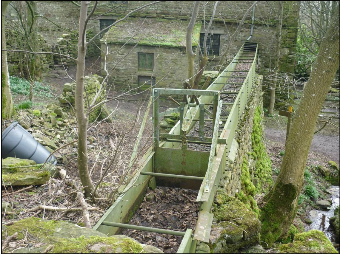
Plate 25: Mill Gill survey area, launder and sluice mechanism (Site 29h), looking SE (photo 8/757).
