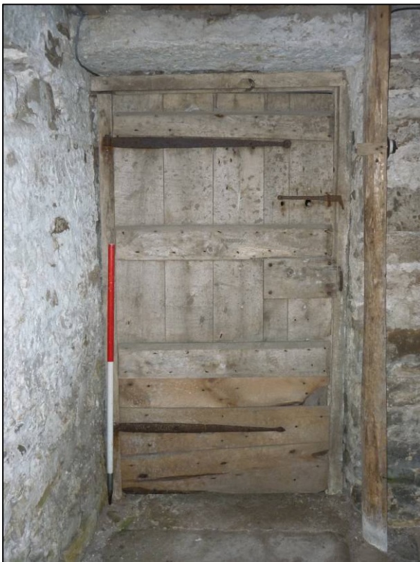
Plate 50: Kiln range (Site 36c), rear of door in west wall (elevation 22) of ground floor room G6, looking W (photo 7/116).
