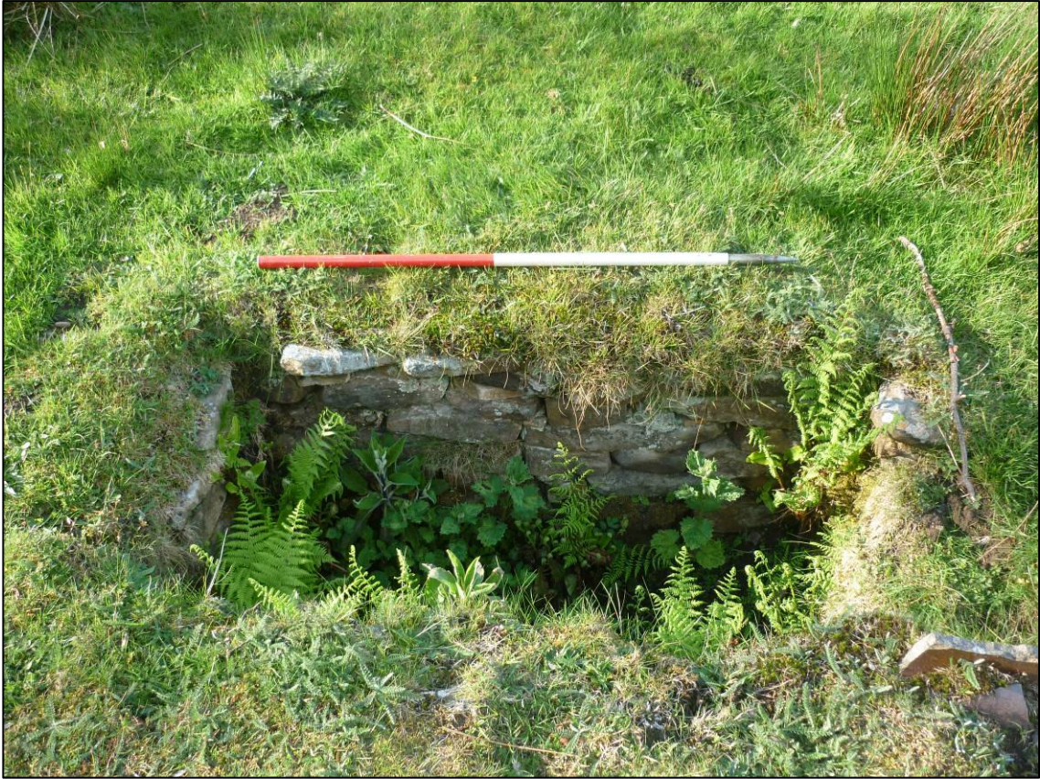
Plate 8: Leas House survey area, inspection pit on line of 1913 culvert (Site 12b), looking N (photo 4/980).
