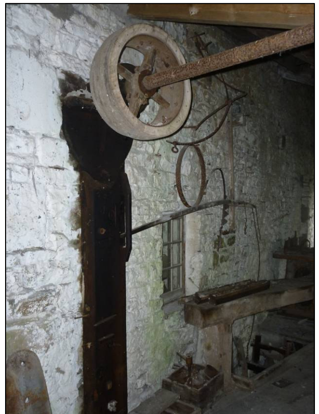
Plate 60: Garage (Site 36b), pulley with wooden casing on line shaft in first floor room 1F12, looking NE (photo 7/925).
