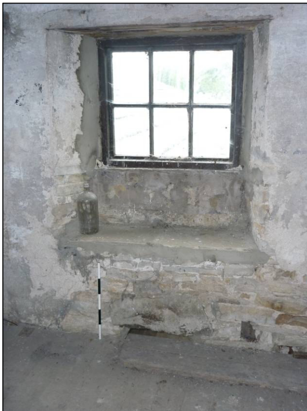
Plate 39: Mill (Site 36a), window at east end of south wall (elevation 11) in second floor room 2F15, looking S (photo 7/887).
