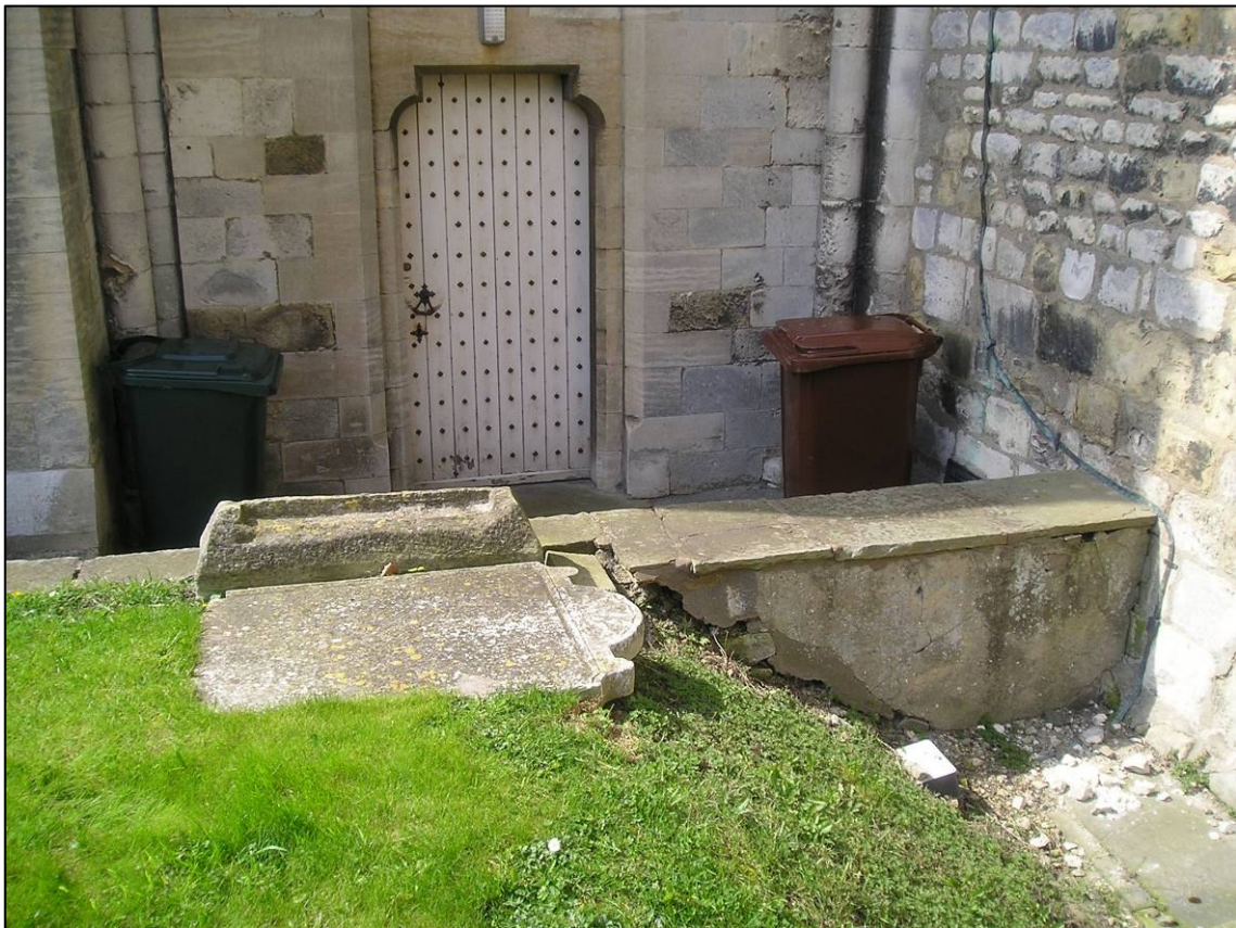
Plate 3: Location of proposed new extension, showing differences in ground levels and existing door into south-west tower, looking north-west.
