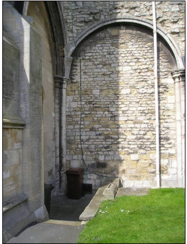
Plate 2: Location of proposed new extension, showing blocked bay of south arcade, looking north.
