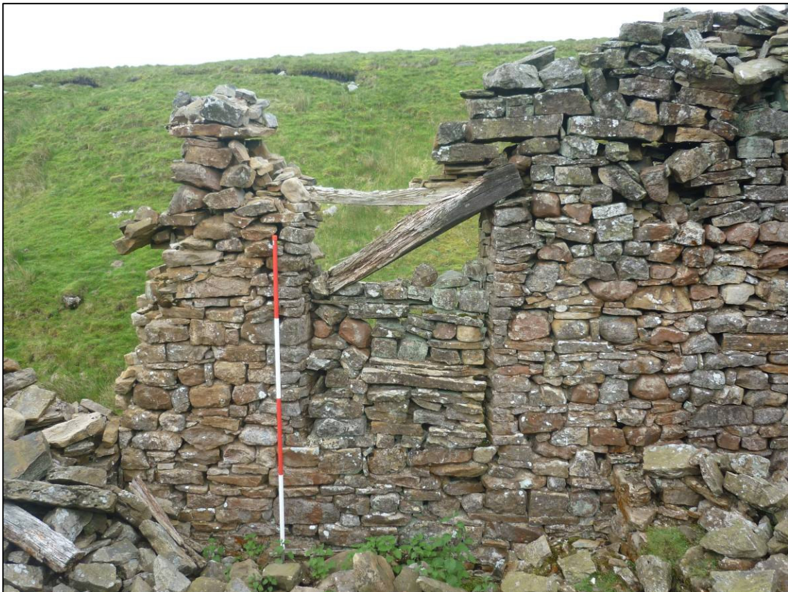
Plate 24: Window in centre of south internal wall of smelt mill (SAR 31.1, elevation 14), looking S (photo 1/427).
