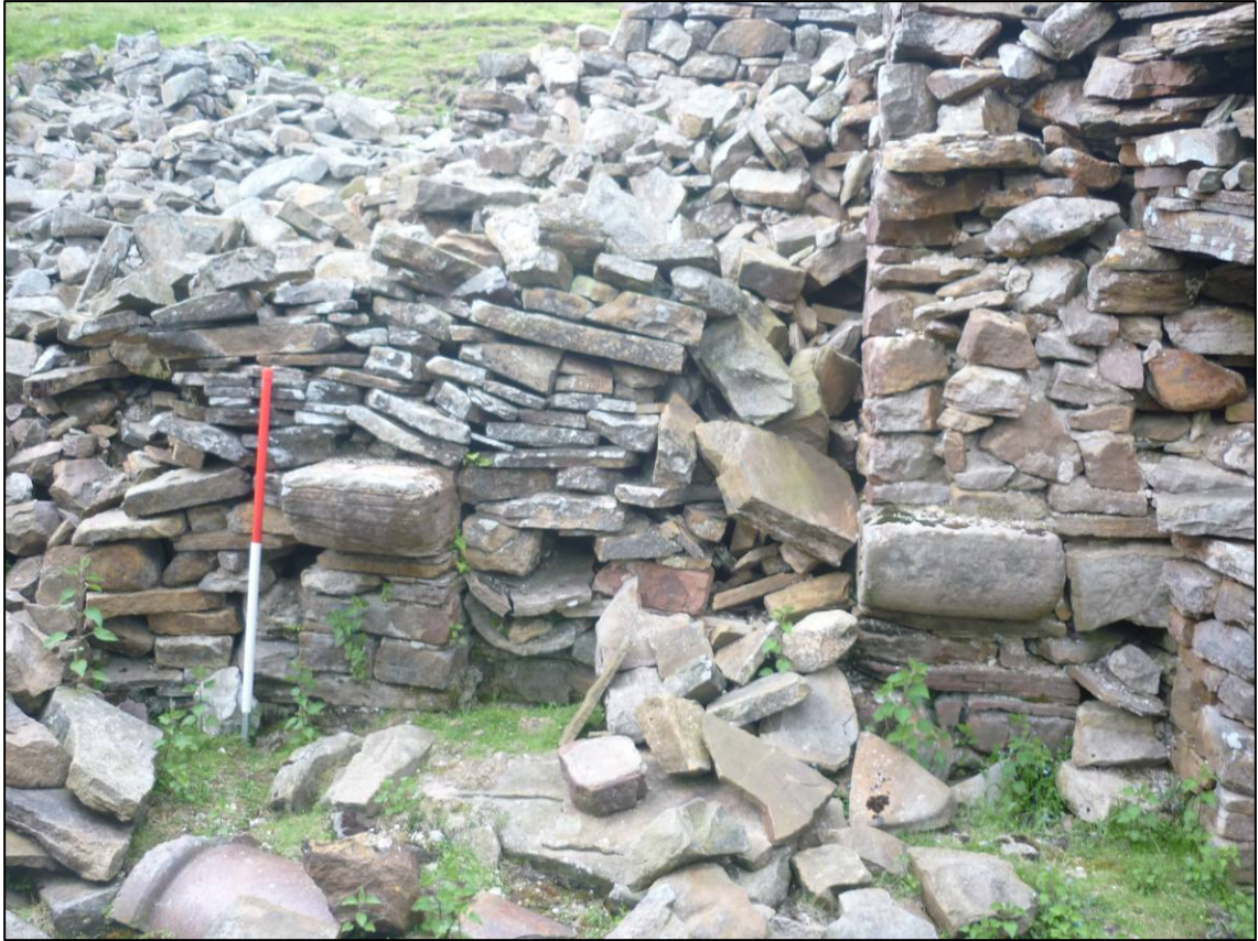
Plate 14: View of ore hearth (SAR 37) with drystone blocking on north side of smelting room (elevation 12), looking N (photo 1/457).
