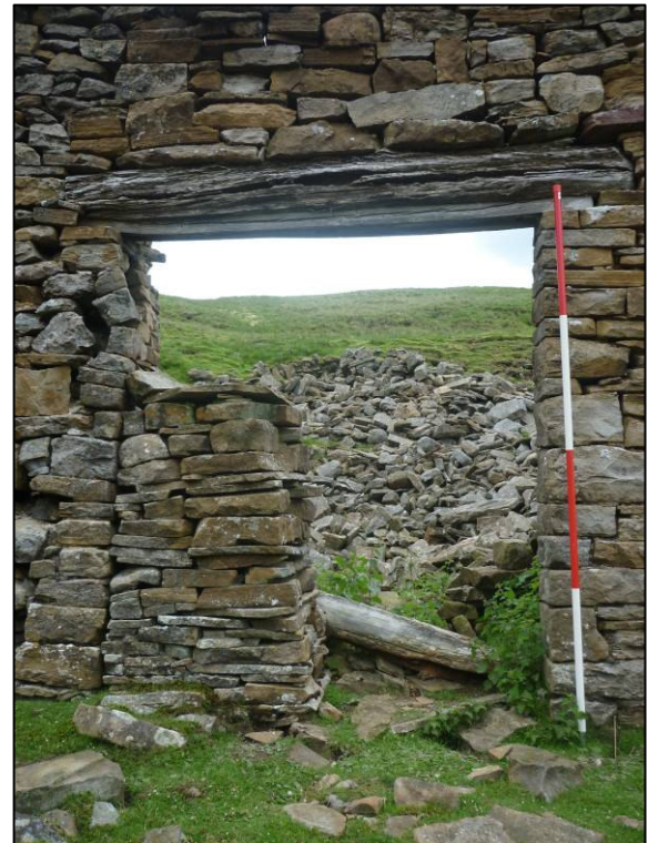
Plate 7: Opening in south wall of blowing room (SAR 31.1, elevation 5), looking S (photo 1/421).
