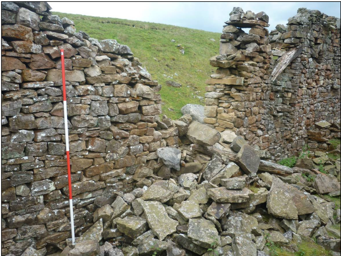
Plate 13: Internal elevation of south wall of smelting room (part of SAR 31.1, elevation 14), looking SW (photo 1/428).
