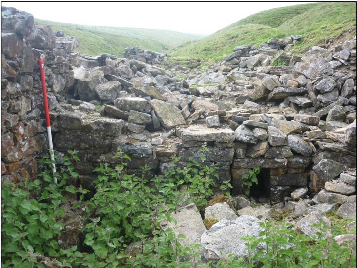
Plate 17: 'Cleaning door' opening in east side of possible settling chamber (SAR 50, elevation 17), looking W (photo 1/467).
