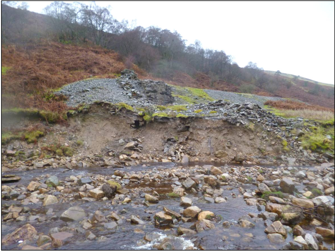
Plate 1: General view of eroding structures on Sir Francis Mine dressing floor, looking NW, November 2012 (photo 1/208).
