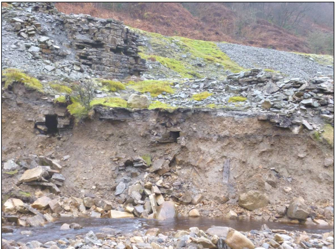
Plate 2: Detailed of eroding structures on Sir Francis Mine dressing floor, looking NW, November 2012 (photo 1/209).
