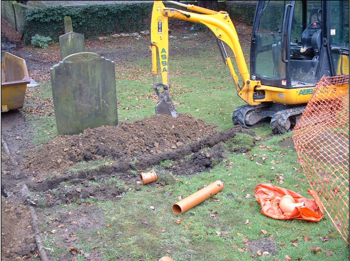
Plate 8: Excavation of Trench 3 on south side of path towards Trench 4, looking E.
