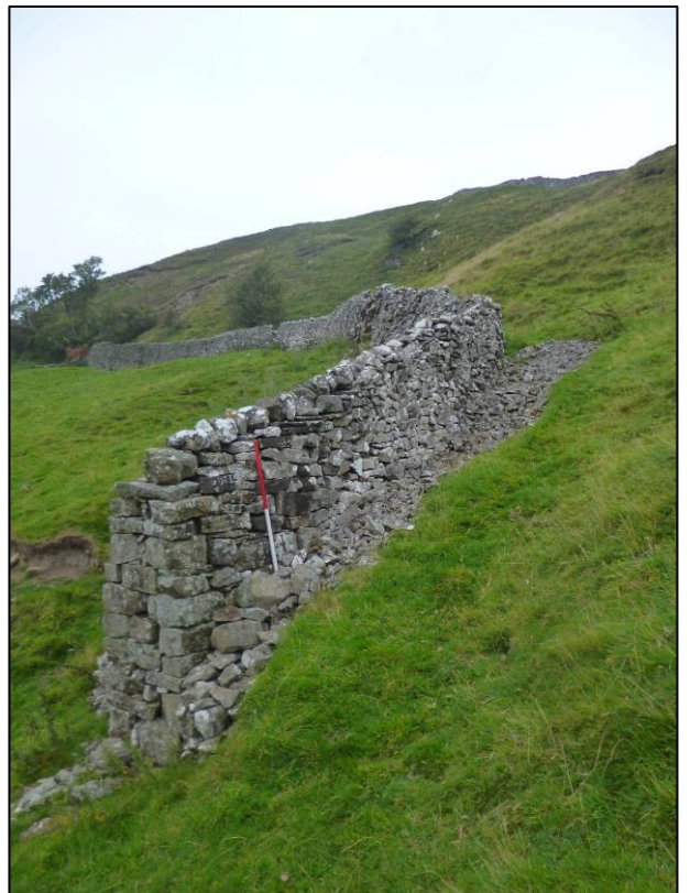
Plate 6: East face of wall to north of east gateway, looking NW (photo 1/960).
