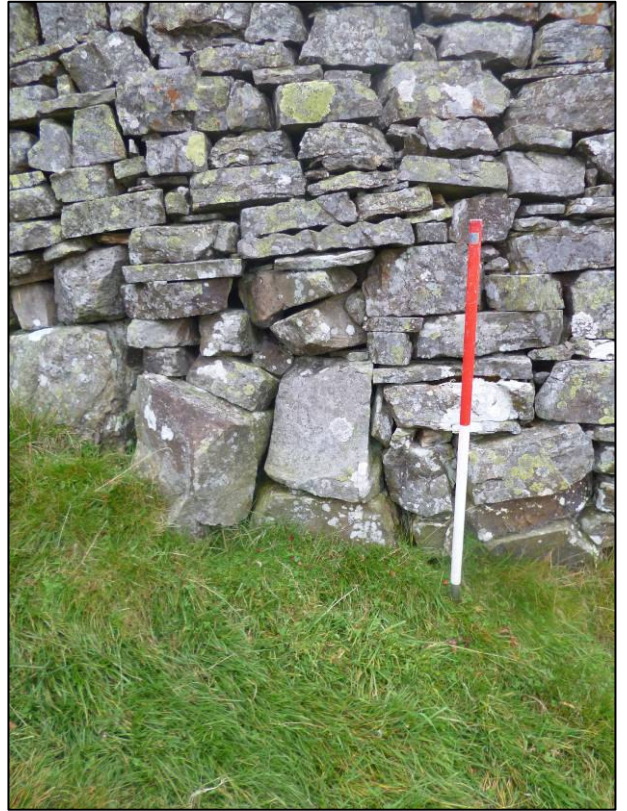
Plate 4: Possible blocked feature in south face of wall west of corner orthostat, looking NE (photo 1/923).
