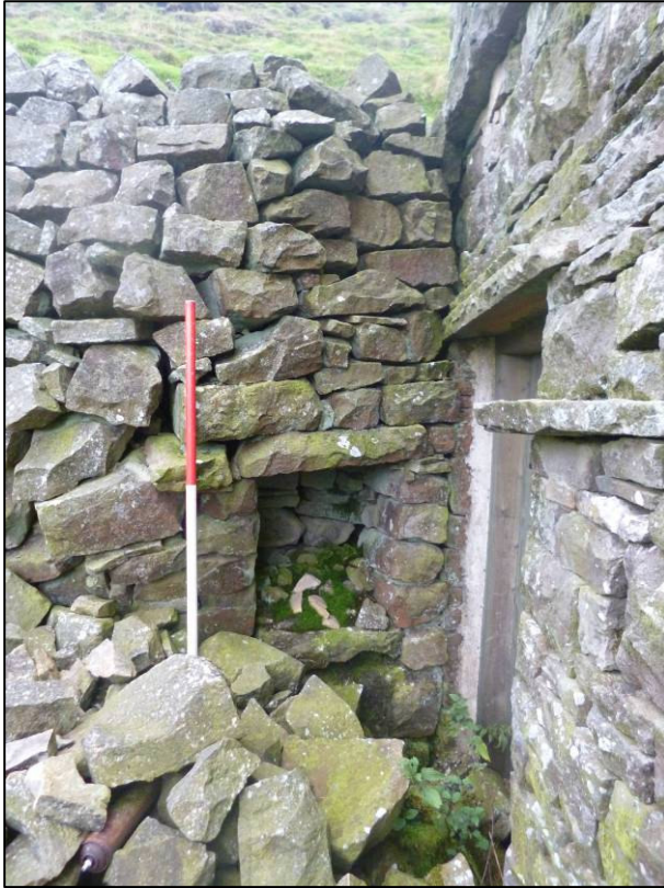
Plate 3: Recess in south face of wall west of barn, looking N (photo 1/903).
