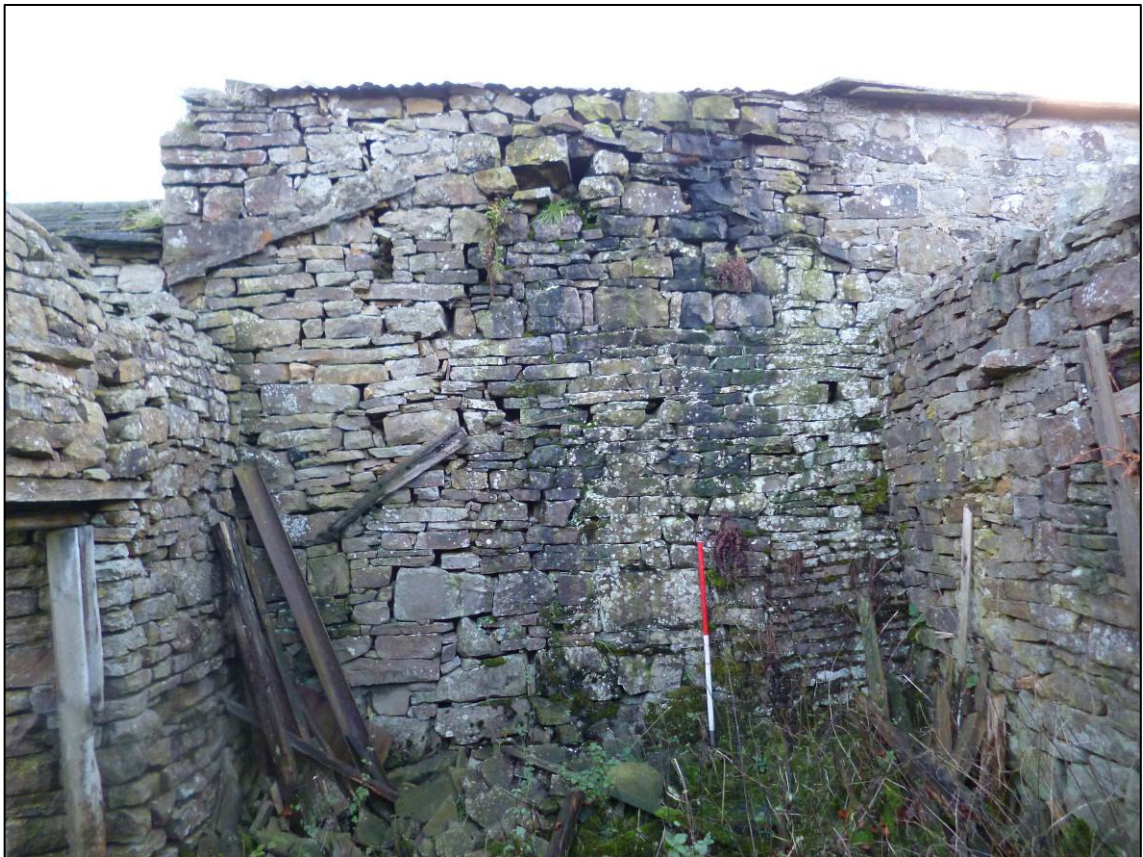
Plate 15: North external wall of house within North Structure, showing shadow of roof and blocked doorway to right, looking SE (photo 3/253).
