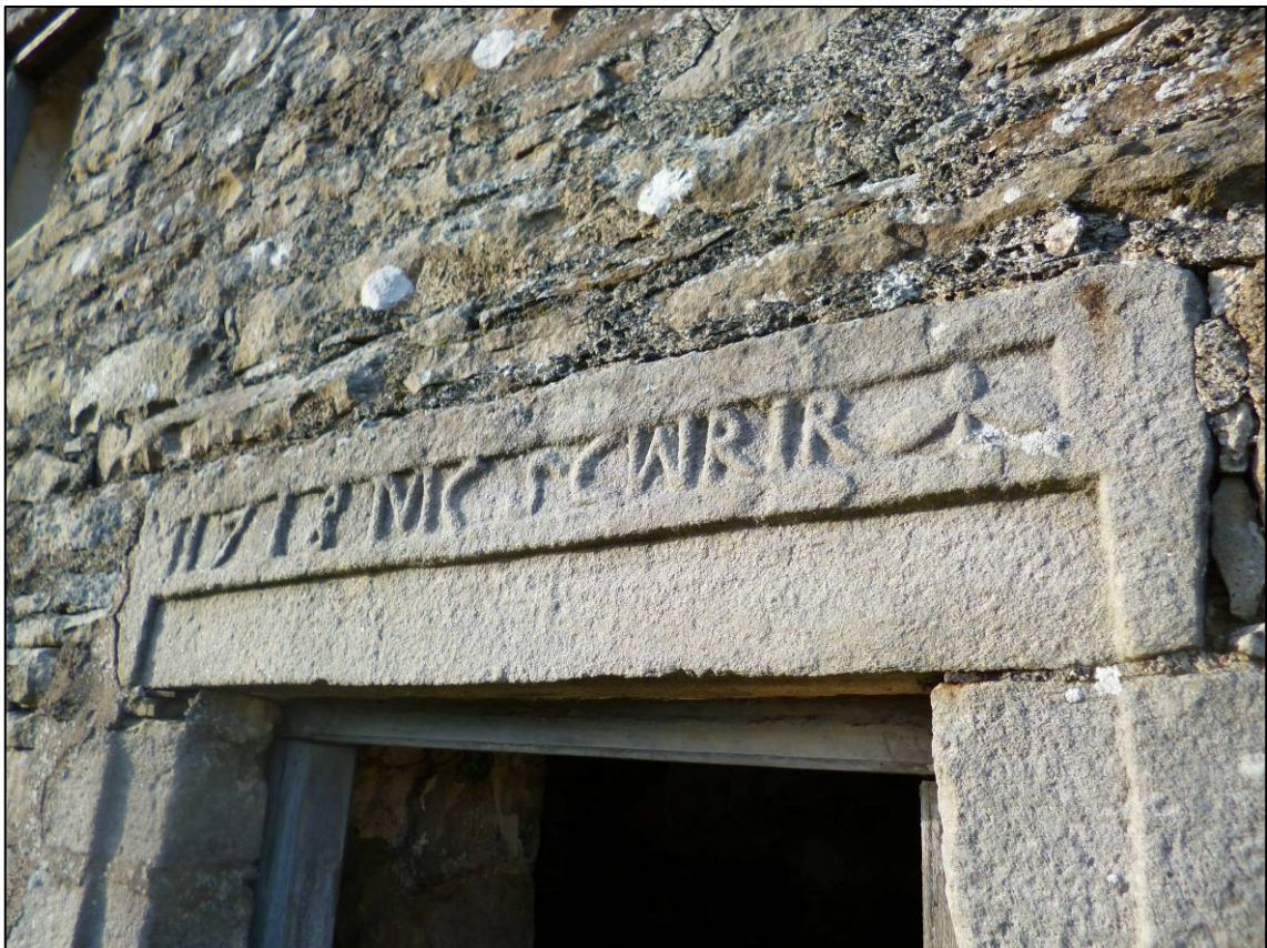
Plate 4: Panel above west cell doorway in south elevation of house, looking NW (photo 3/305).
