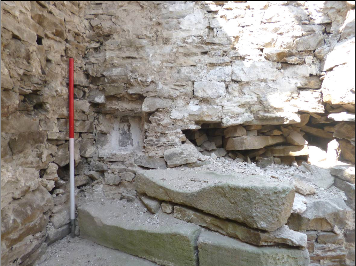
Plate 12: Recess (possible window?) at head of stairs, west end of north wall of west cell, looking NW (photo 4/058).
