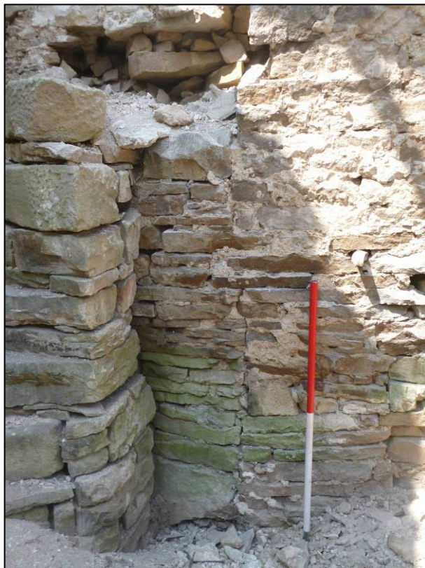
Plate 10: Blocked opening hidden by stairs in west ground floor cell, looking NW (photo 4/055).
