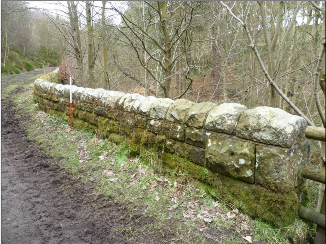
Plate 10: Parapet of revetment wall (Site 17/5), east of Rivelin Bridge, looking NW (photo 3/886).
