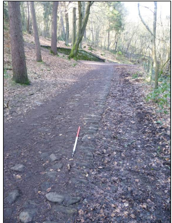
Plate 9: Exposed kerb in Wyming Brook Drive east of Millstone Hole, looking NW (photo 2/825).
