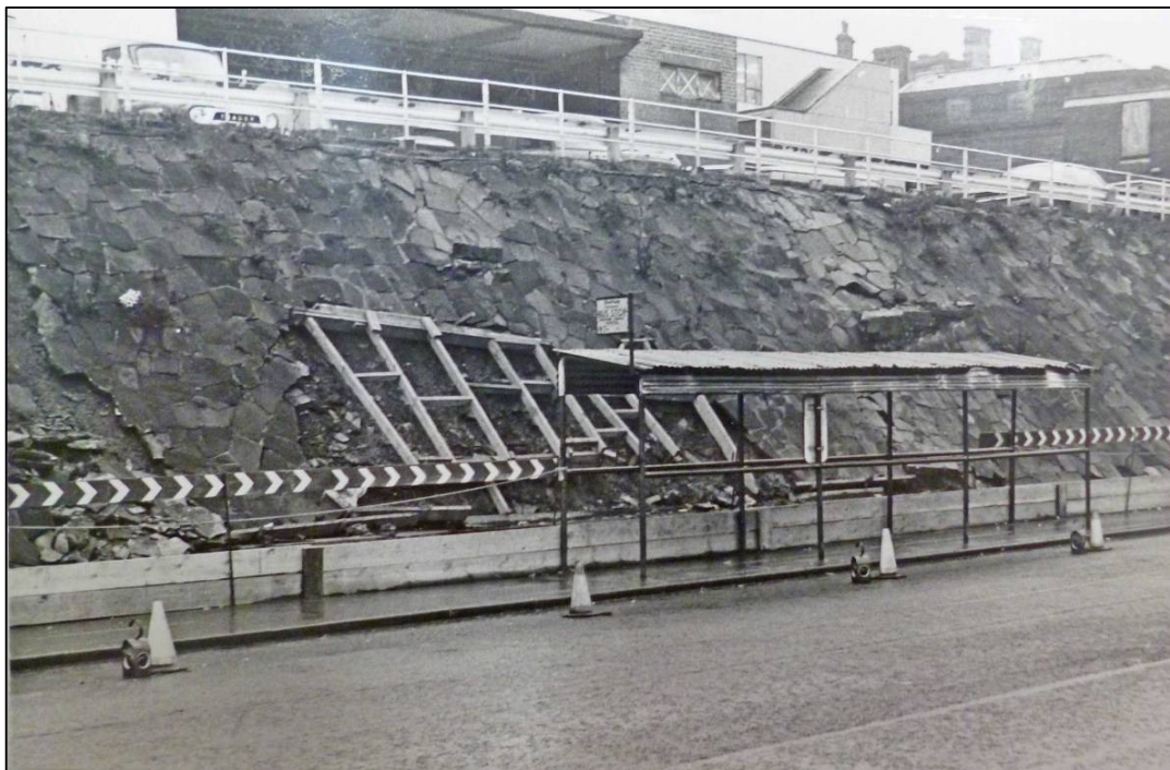
Plate 46: Collapsing paving covering the steep north-facing slope to Castlegate, photographed by Pauline Beswick, May 1972 (MSA Box file - Sheffield Castle Project File) (photo 3/884).
