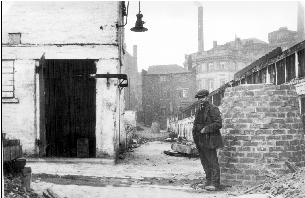
Plate 9: Demolition of Shambles Slaughter House, newly built sewer manhole (for a new road for the continuation of Bridge Street) right, Lady's Bridge Hotel and Exchange Brewery in background, taken by J B Himsworth, September 1929 ( www.picturesheffield.com , y00890).
