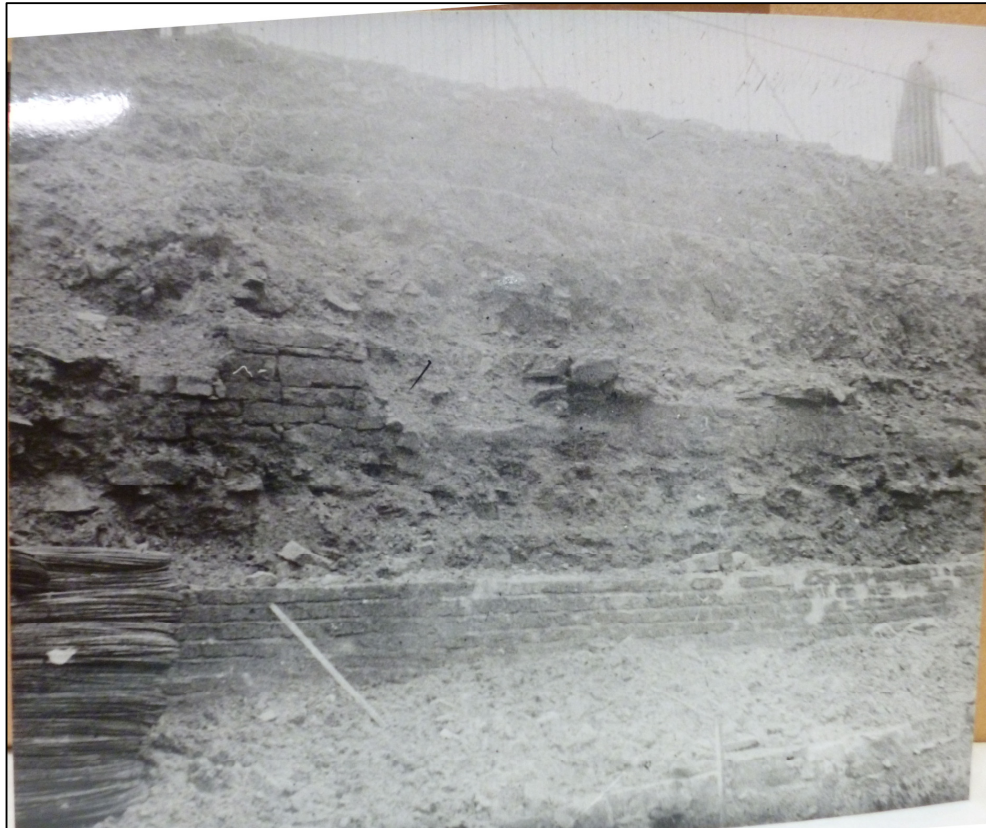
Plate 41: Stepped bank on south side of Castlegate created by cutting back behind the former retaining wall to Chandlers Row (photo 2/683).
