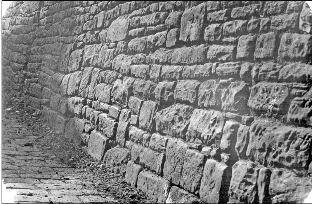
Plate 5: Retaining wall on west side of Castle Folds Lane, taken by J B Himsworth, September 1928 ( www.picturesheffield.com , y00898).
