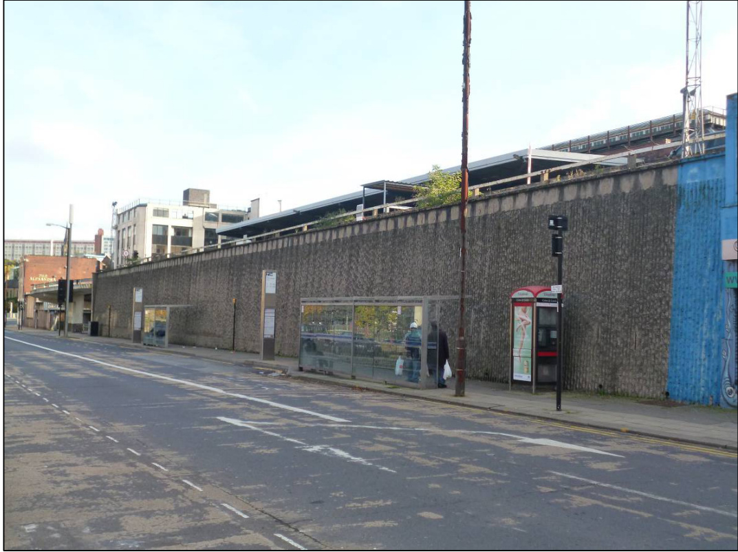
Plate 33: 1972 retaining wall on south side of Castlegate, with North Loading Dock above (photo 4/388).
