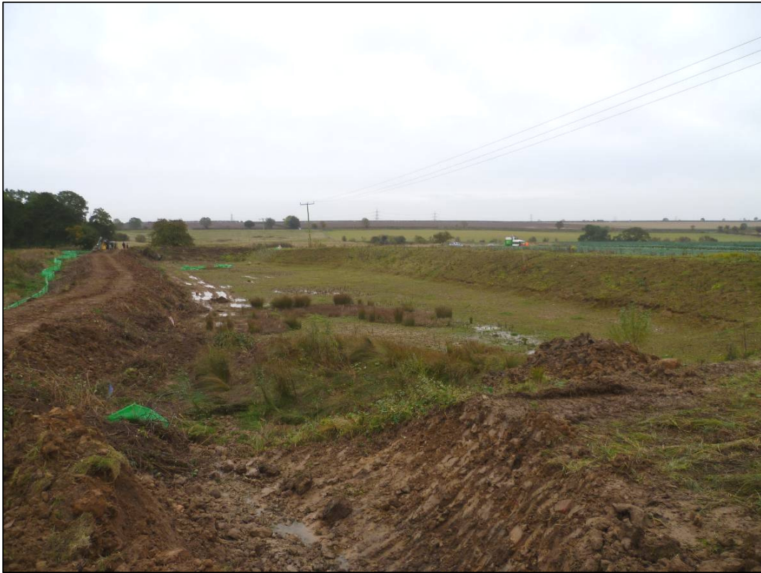
Plate 1: Central pond prior to start of work, showing cut through northern dam, looking SW.
