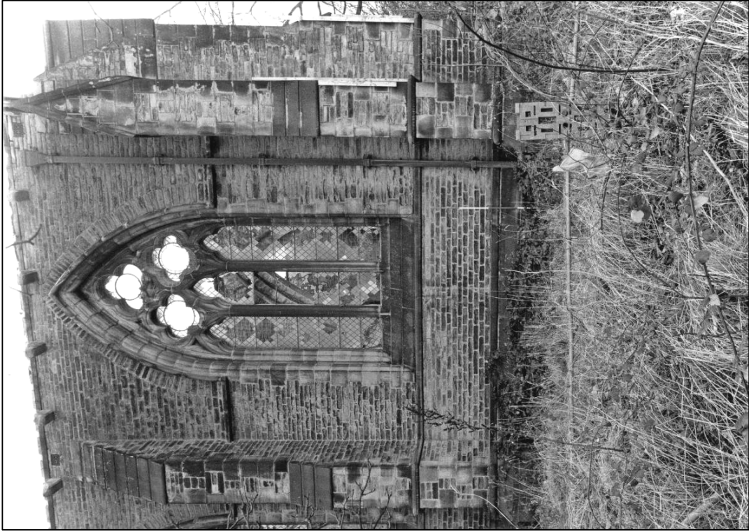
Plate 5: Typical window, east end of south elevation, looking N (photo 2/18) (top to left).
