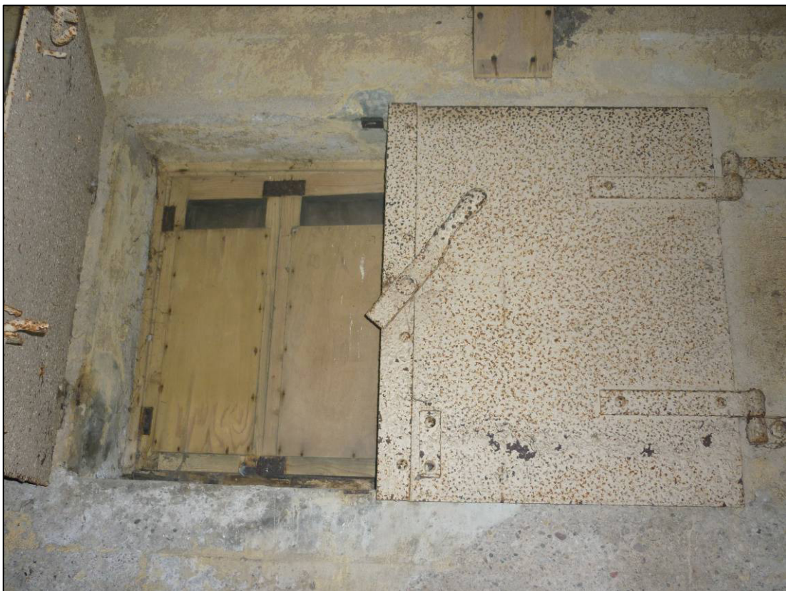
Plate 26: Building R4, internal north elevation of west room, showing blast shutters and folding wooden shutters, looking N (photo 3/282, January 2012).
