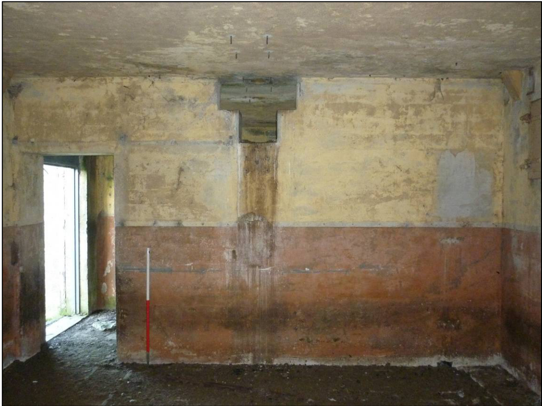
Plate 29: Building R4, east internal elevation of central room, showing decoration, fittings for sliding door, T-shaped opening and roof bolts, looking NE (photo 2/982, December 2011).
