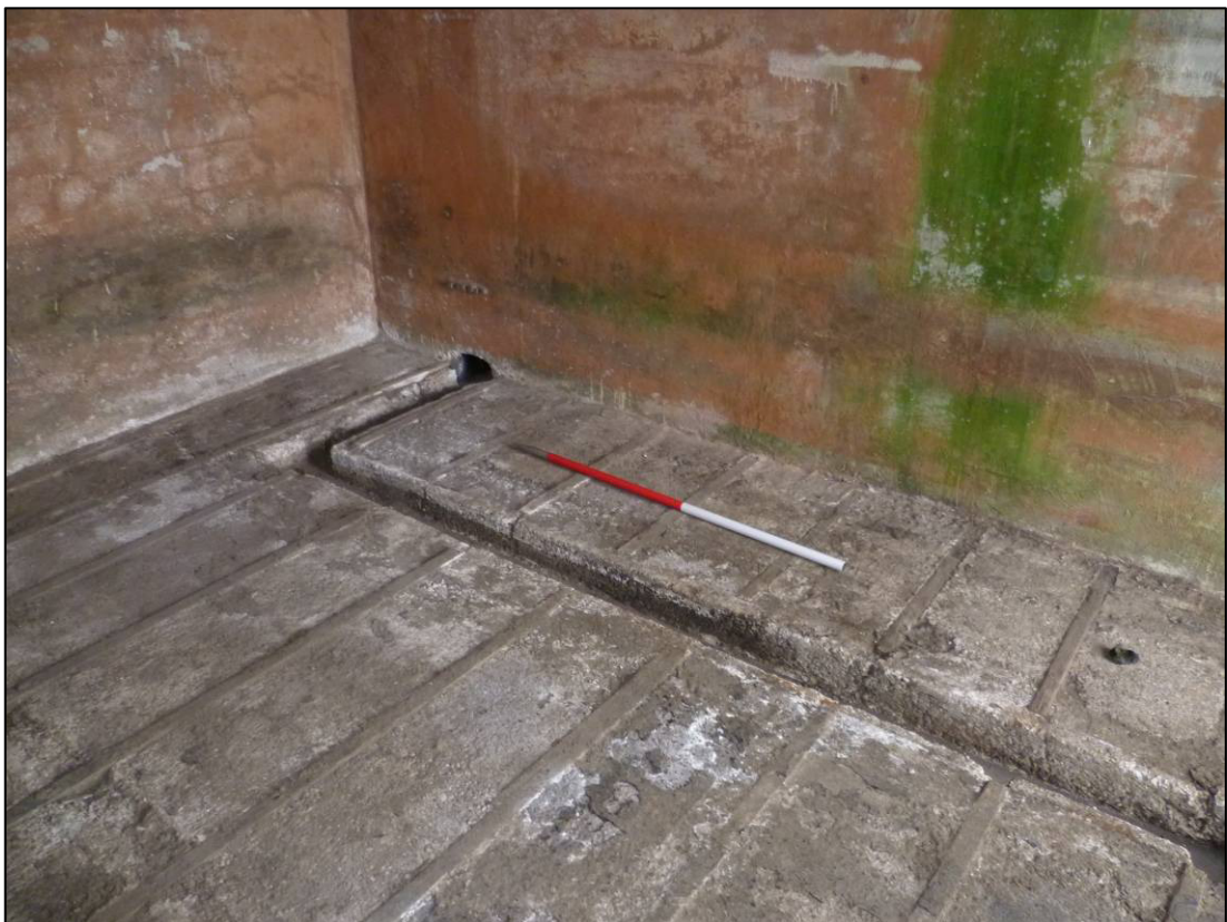
Plate 30: Building R4, floor of east room after clearance showing cable ducts and battens in concrete floor, looking E (photo 4/587, February 2012).
