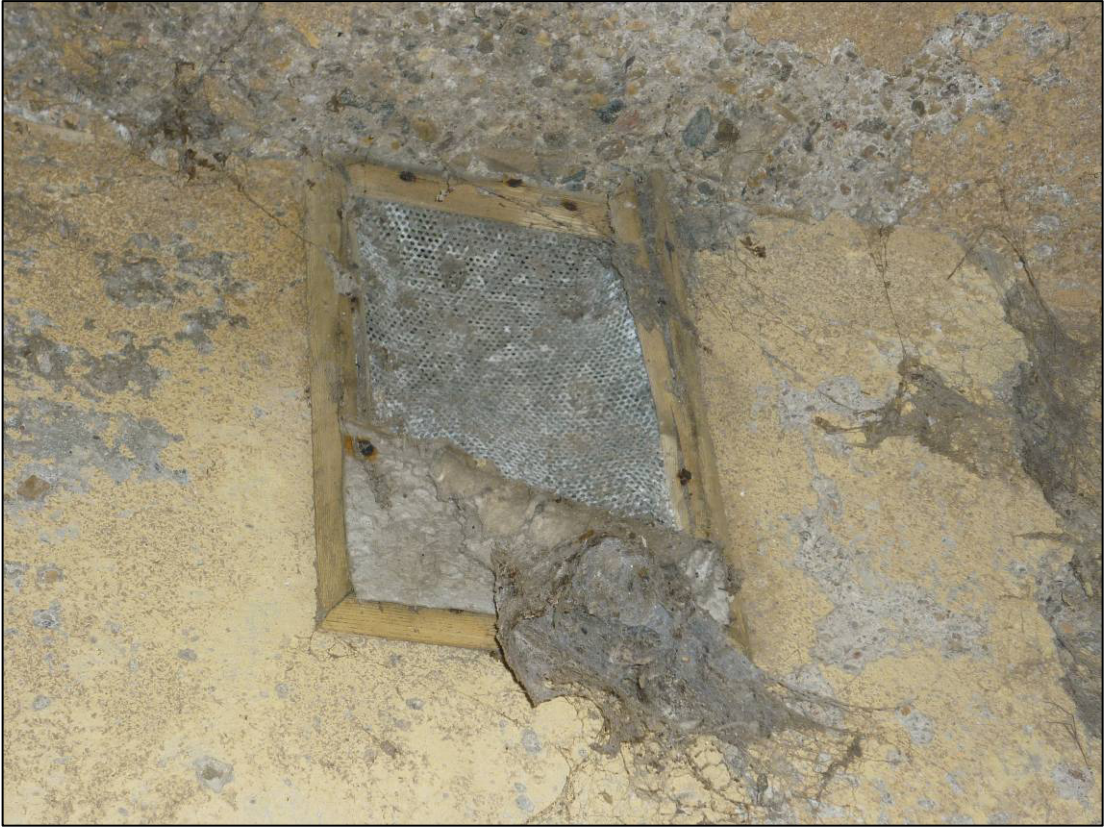
Plate 27: Building R4, east internal elevation of east room, detail of covered vent, looking NE (photo 2/981, December 2011).
