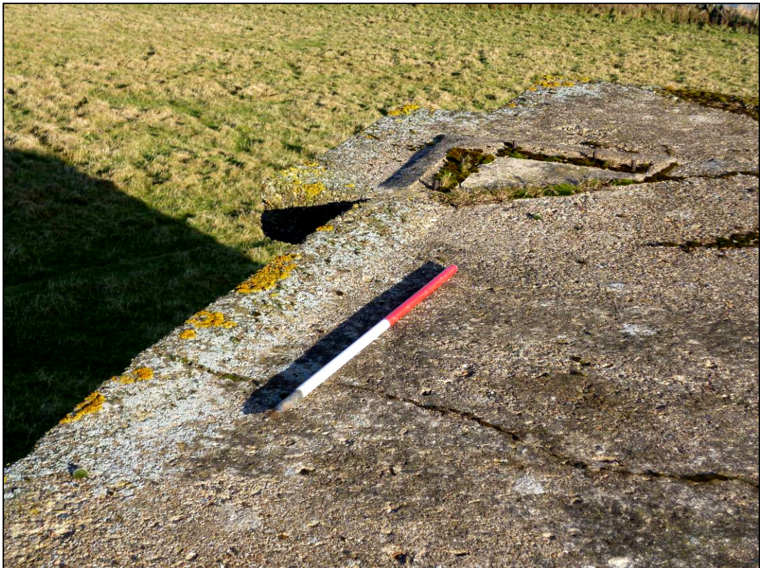
Plate 22: Roof of Building R4, showing base of radar array and lip over doorway D1, looking NE (photo 5/385, December 2012).
