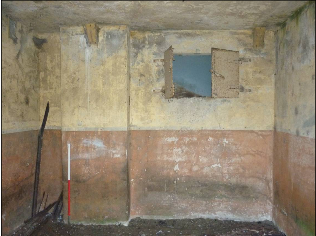
Plate 25: Building R4, internal south elevation of east room showing decoration, blast doors to window and triangular wooden blocks, looking S (photo 2/978, December 2011).
