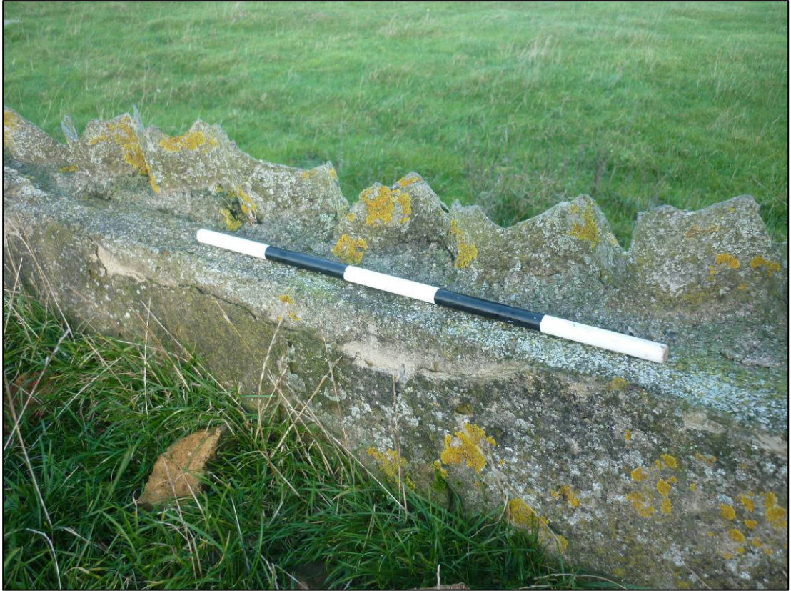
Plate 39: Building A11, remains of asbestos wall on east side, looking N (photo 2/941, December 2011).
