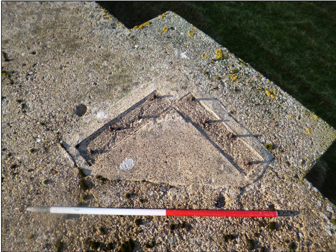
Plate 23: Roof of Building R4, north-west base of radar array, looking NW (photo 5/384, December 2012).
