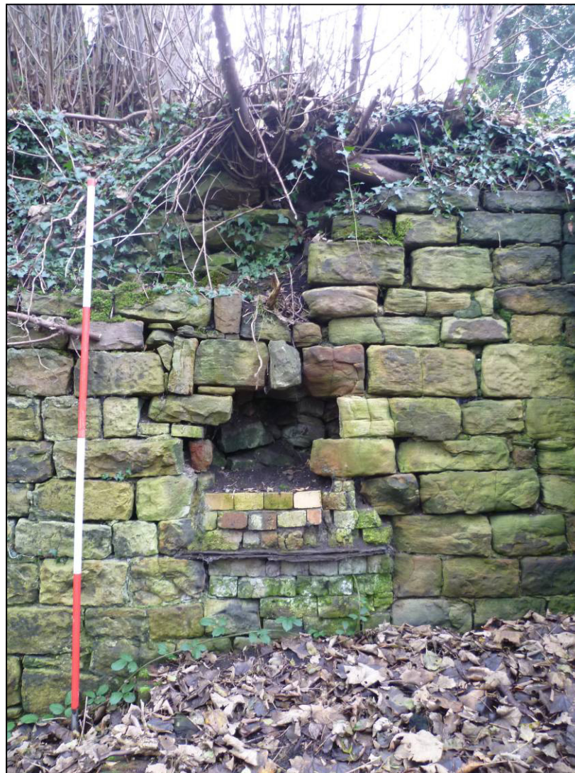
Plate 18: Area 3 dam wall prior to repair, looking S (photo 1/387).
