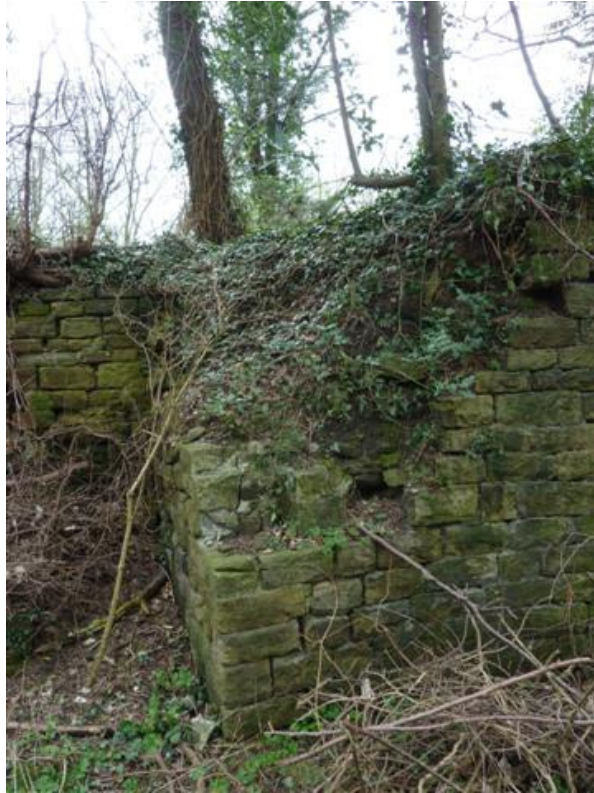
AREA 2 – coursed rubble wall section with collapsed corner. This corner is to be rebuilt to the height of adjacent wall sections, strengthened using helibars and re-pointed
