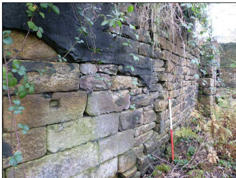
Plate 3: Area 1 dam wall prior to repair, showing displacement at fracture, looking W (photo 1/375).
