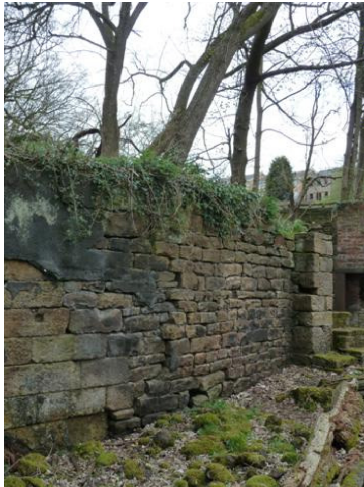
AREA I – junction of coursed rubble and ashlar where outward displacement of the rubble masonry has occurred. This area is to be re-pointed and strengthened with bed joint reinforcement where displacement has occurred
