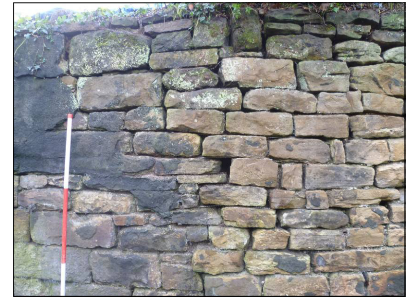
Plate 5: Area 1 dam wall, detail of vertical fracture, looking S (photo 2/413).
