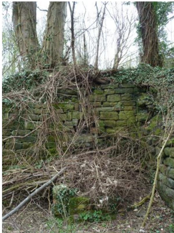
AREA 3 – coursed rubble section with voids and fractures, This section is to be re-pointed, cracks are to be repaired and missing stones are to be reinstated
