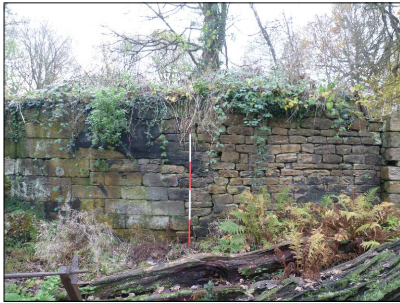
Plate 1: Area 1 dam wall prior to repair, looking S (photo 1/373).
