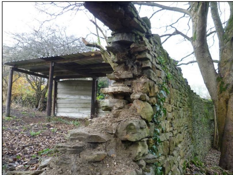
Plate 24: Area 4 boundary wall prior to repair, showing double skin and core, looking NW (photo 1/367).
