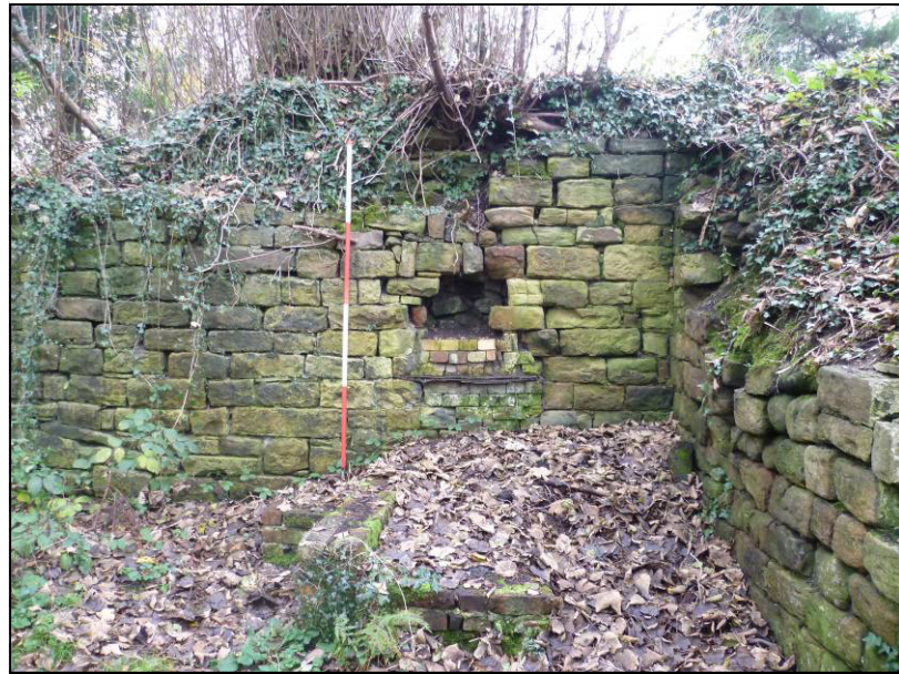
Plate 17: Area 3 dam wall prior to repair, looking S (photo 1/386).
