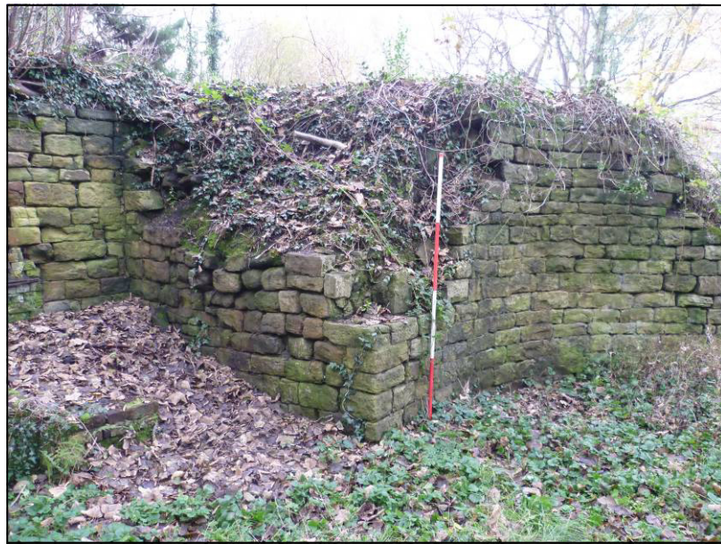
Plate 9: Area 2 dam wall prior to repair, looking SW (photo 1/379).
