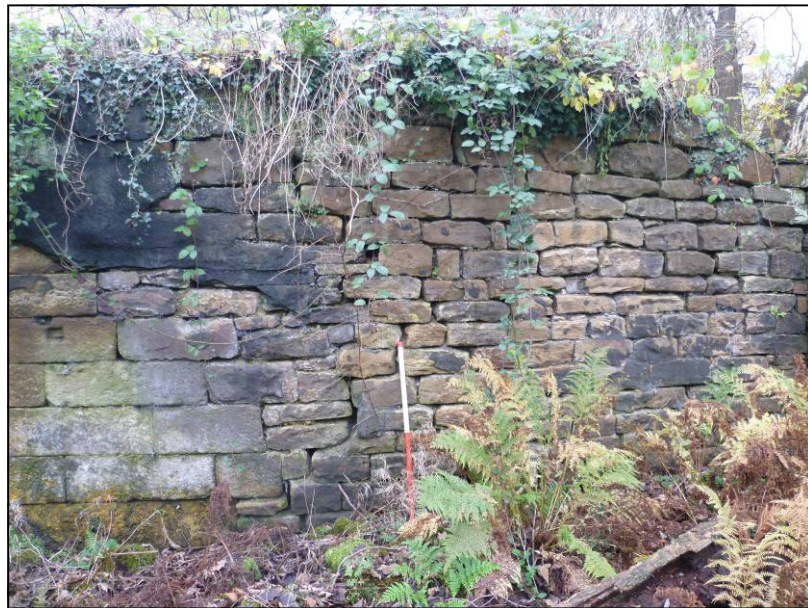
Plate 2: Area 1 dam wall prior to repair, showing vertical fracture, looking S (photo 1/377).
