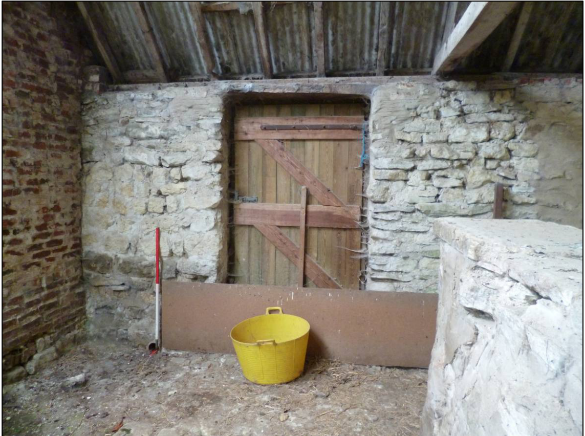
Plate 12: 'To-be-demolished' building, doorway at north end of east wall, looking E (photo 1/592).
