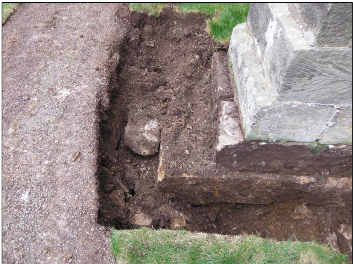
Plate 4: Trench 2 under excavation, showing foundations of southern buttress (208) and construction backfill (204), looking N.
