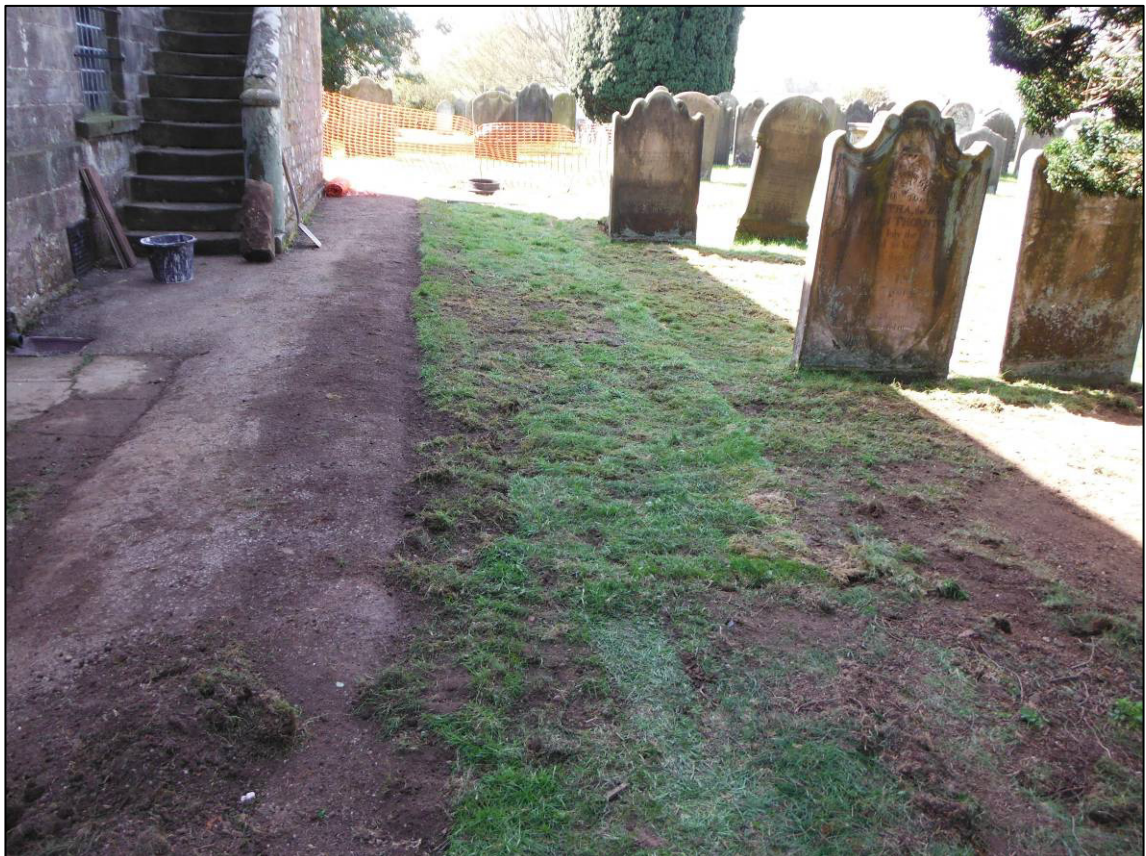
Plate 12: Trench 4 reinstated after installation of Trench Arch worm bed drainage system, looking W.
