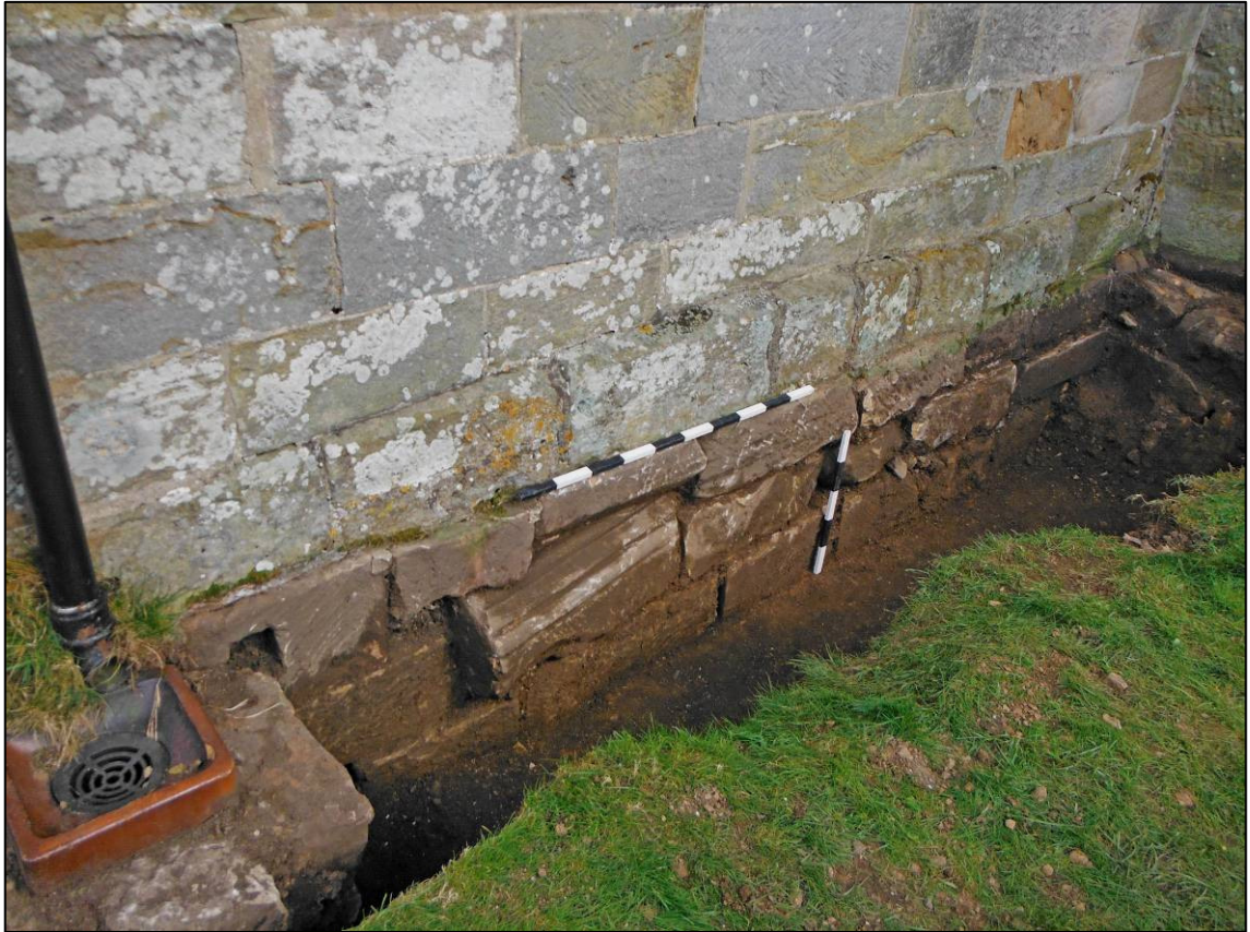
Plate 1: Excavated Trench 1, showing reused stone in foundations (107) of south wall of church, looking NE.
