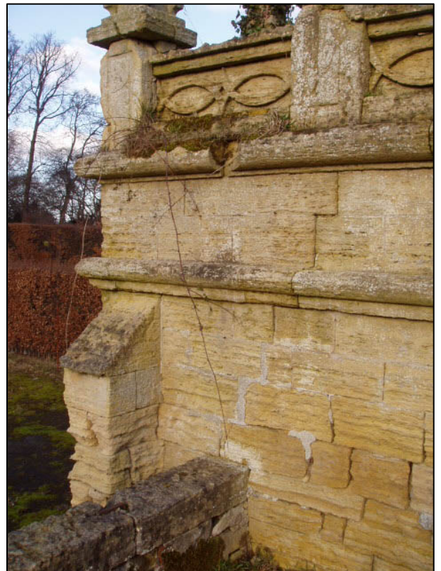
Plate 8: North-west corner of central cell, showing stringcourse and parapet, looking N (Peter Pace photograph).
