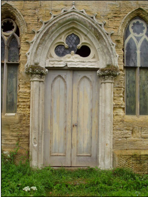
Plate 5: Door to central cell in north elevation, looking SE (Peter Pace photograph).
