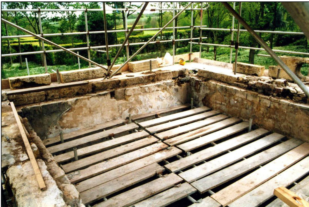
Plate 12: Central cell after removal of concrete roof, showing profile of former cross-vault, looking E (photo 5/34).
