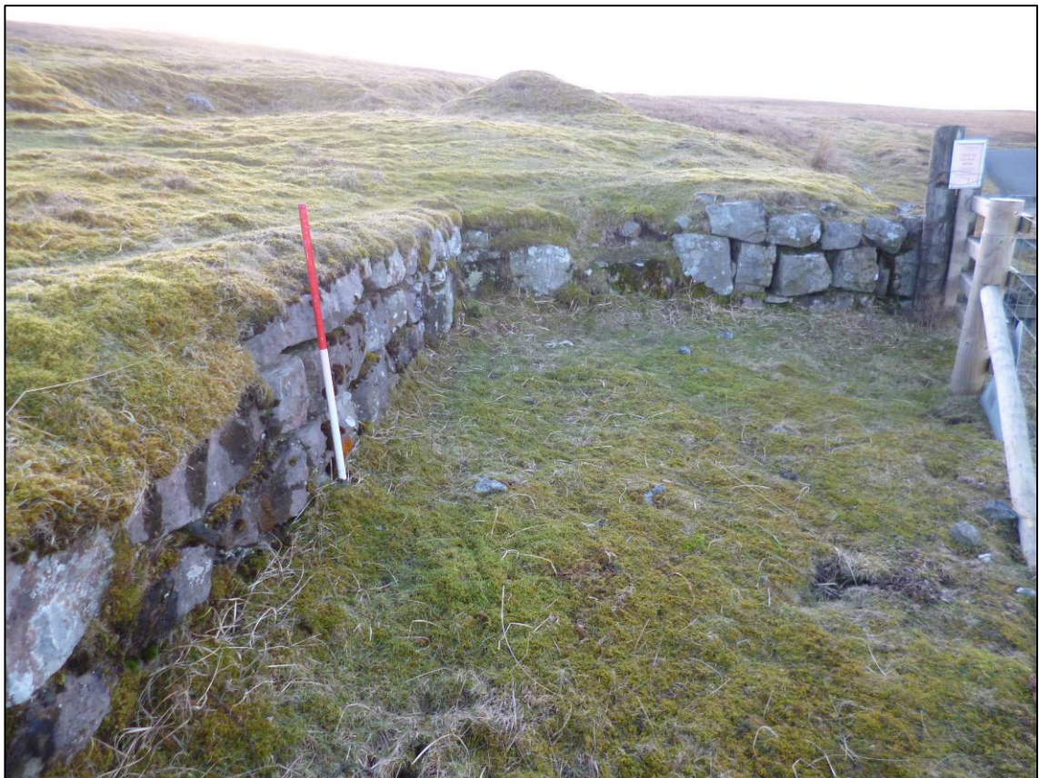
Plate 36: Loading bay (Site 25) adjacent to Reeth to Tan Hill road, looking W (photo 3/074).
