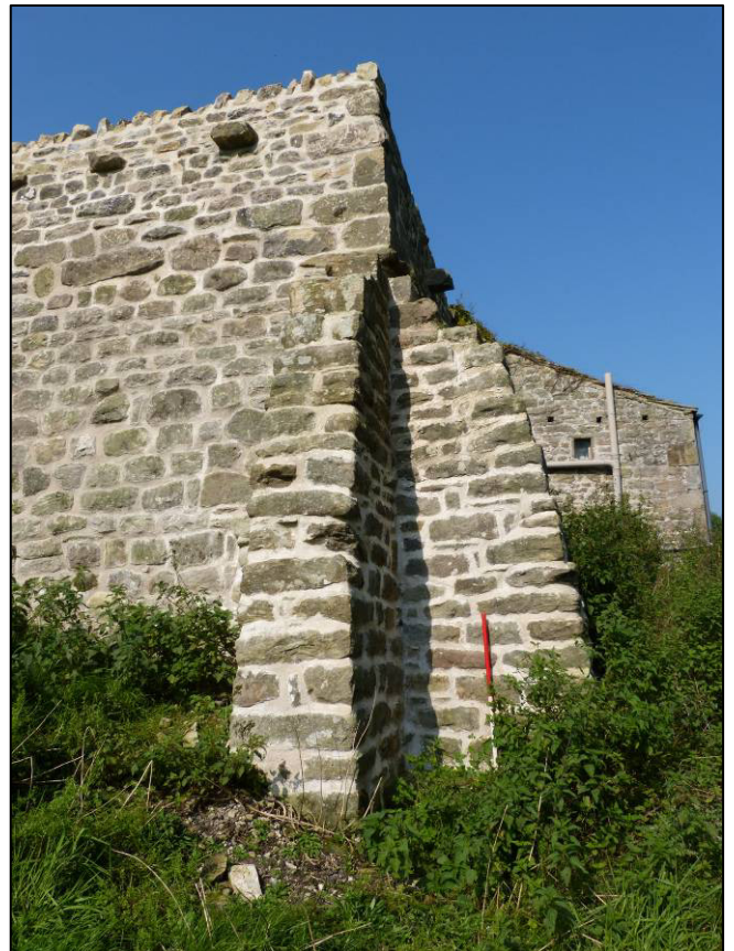
Plate 41: Retaining walls, north-east of chapel, corner buttress, works complete, looking NW (photo 7/593).
