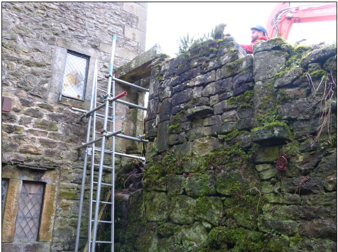
Plate 28: Retaining wall to sunken area north of chapel, doorway and fireplace, looking W (photo 3/393).
