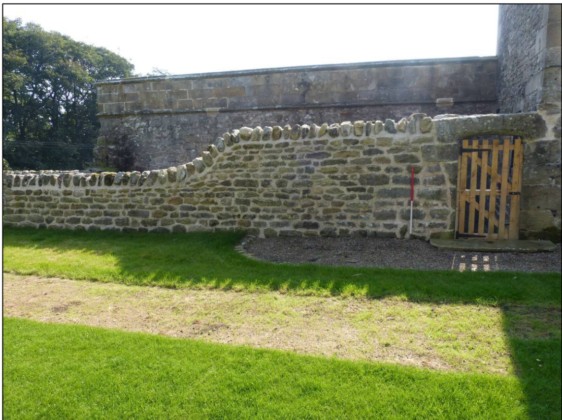
Plate 42: Sunken area to north of chapel, rebuilt doorway in west end of revetment wall, looking SE (photo 7/571).
