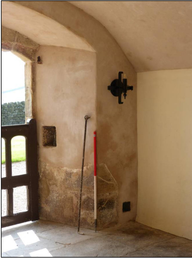
Plate 19: Tower, lower ground floor entrance chamber interior, works complete, looking S (photo 7/602).
