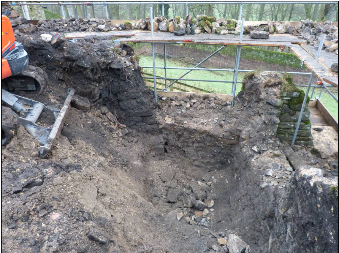
Plate 30: Retaining wall, north-east of chapel, dismantling wall showing earlier buttress, looking NE (photo 4/443).
