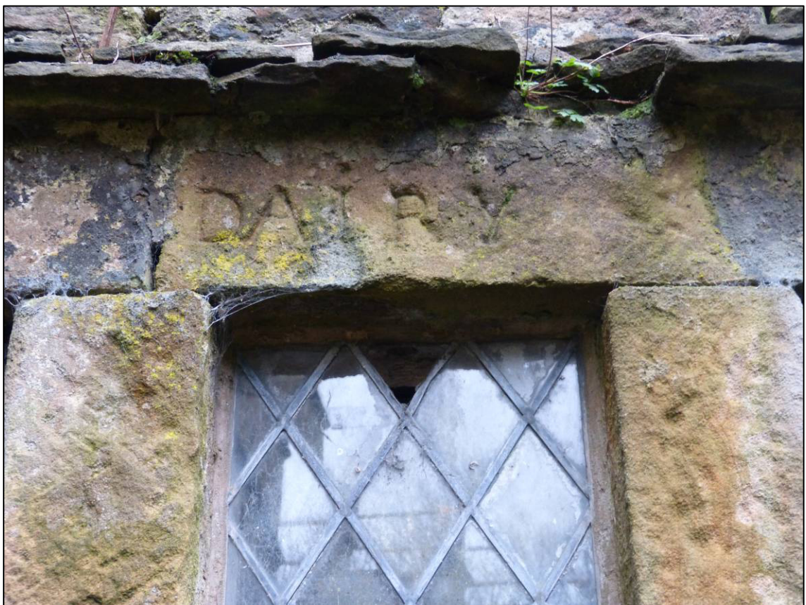
Plate 16: Domestic block, lower ground floor, east gable, window inscription, looking SW (photo 3/398).
