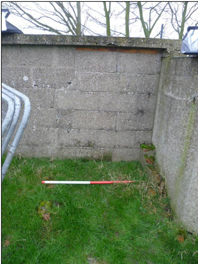
Plate 52: Structure F (gun emplacement), brick stub walls off end of shelter with blocked opening, looking E (photo 6/722).
