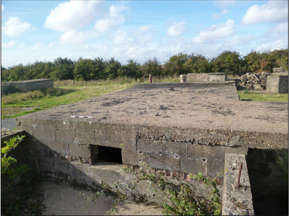
Plate 38: Structure B (command post), east end and roof of Room 3, looking SW (photo 2/162).
