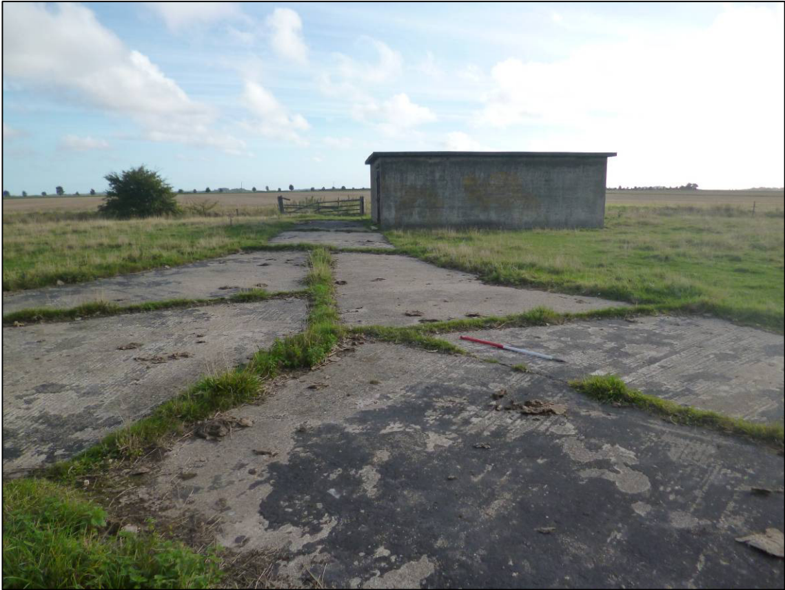
Plate 21: Concrete roadway with bitumen coating, west of Structure E, looking NE (photo 2/082).
