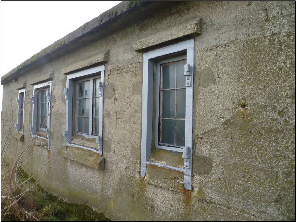
Plate 64: Structure E (gun store), east elevation windows during conservation, looking SW (photo 4/708).
