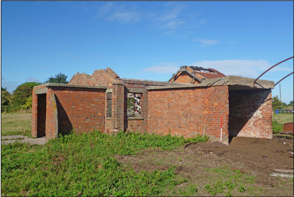
Plate 11: Structure A3 (cookhouse), showing south and east linking structures, looking NW (photo 1/578).
