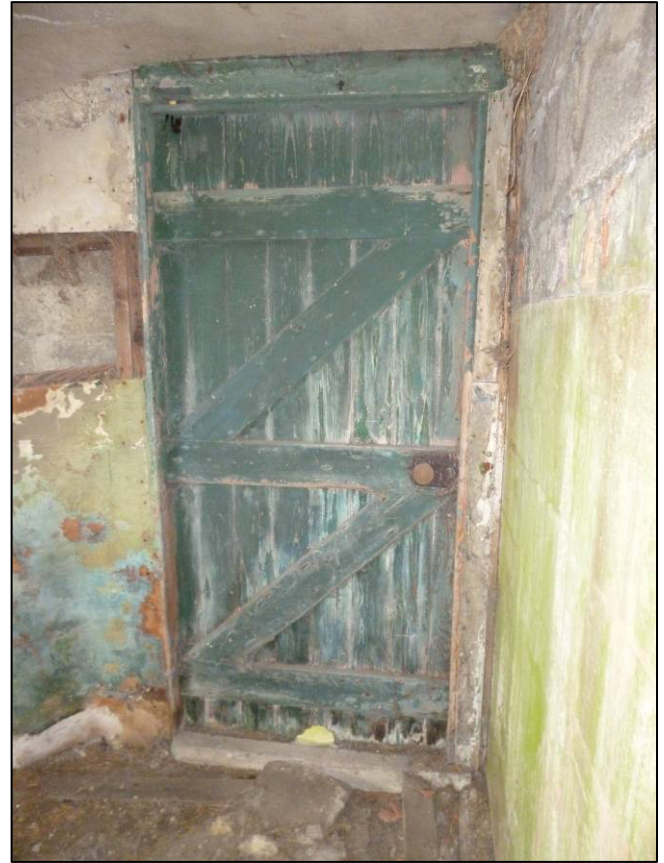
Plate 26: Structure B (command post), Room 3 interior, door in north wall, looking NW (photo 2/174).
