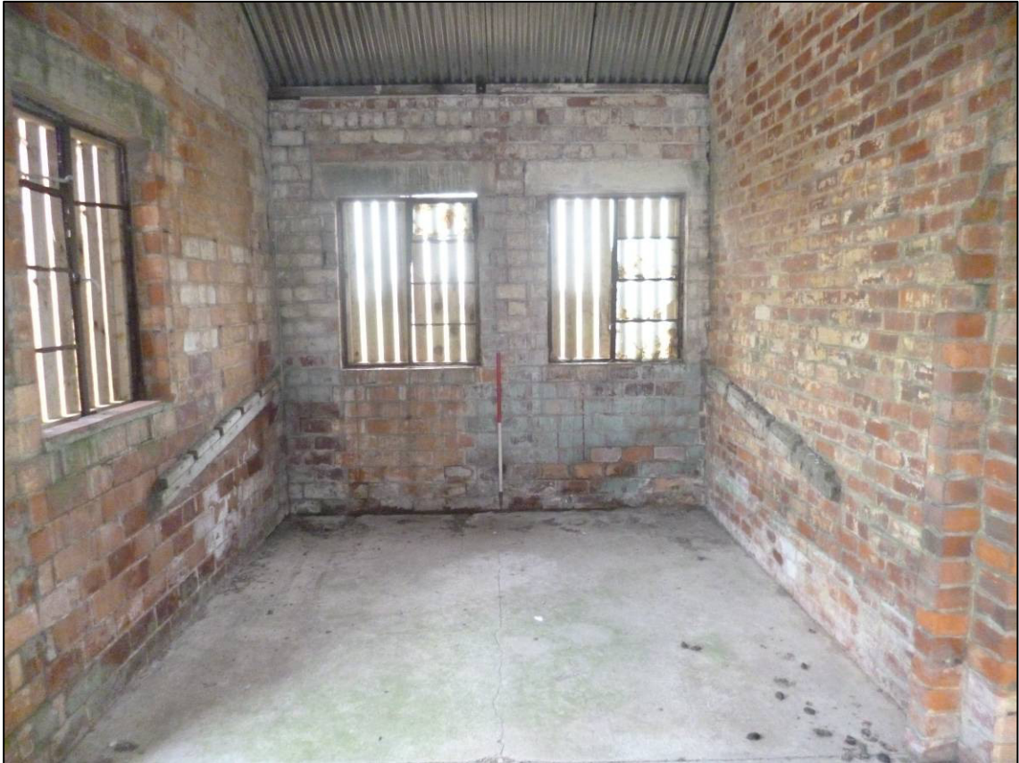
Plate 17: Structure A3 (cookhouse), interior of north cell after clearance and repairs, showing sloping timbers, looking E (photo 4/866).
