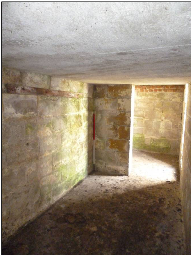
Plate 45: Structure C (gun emplacement), interior of west cell of shelter, looking SE (photo 2/203).
