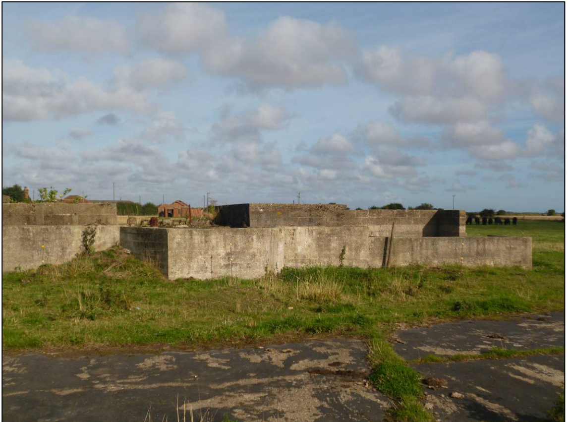
Plate 29: Structure B (command post), east end of south elevation, looking NW (photo 2/132).
