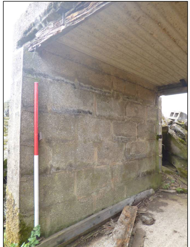
Plate 46: Structure D (gun emplacement), Type 1 ammunition recess on north-east side, looking NW (photo 3/295).
