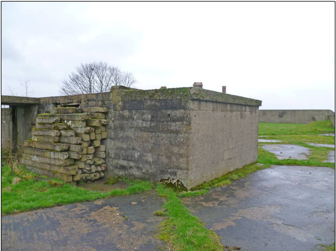
Plate 23: Structure B (command post), west end of north elevation, showing blocked doorway and extension to Room 3, looking SE (photo 6/699).
