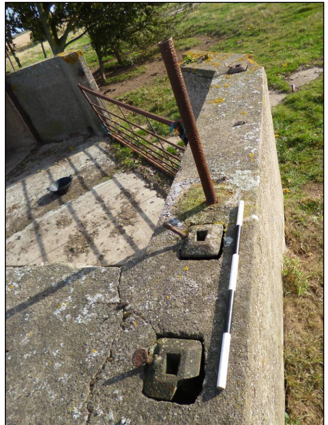
Plate 53: Structure F (gun emplacement), camouflage fittings on south-east side, looking NW (photo 2/116).
