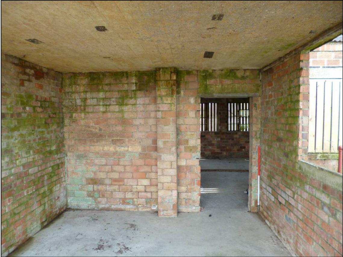
Plate 19: Structure A3 (cookhouse), central part of east elevation (within east link structure) after clearance, looking W (photo 4/863).
