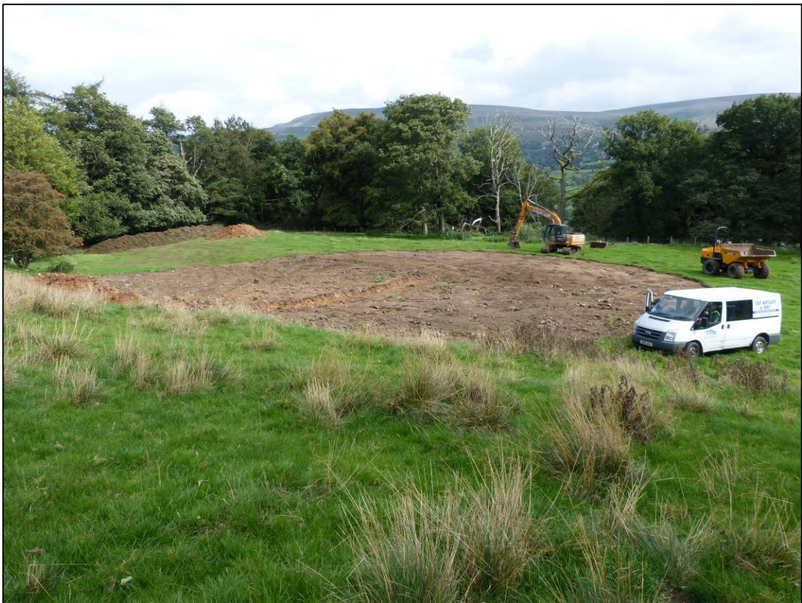
Plate 6: General view of completed topsoil stripping and exploratory trench, looking SE (photo 2/226).
