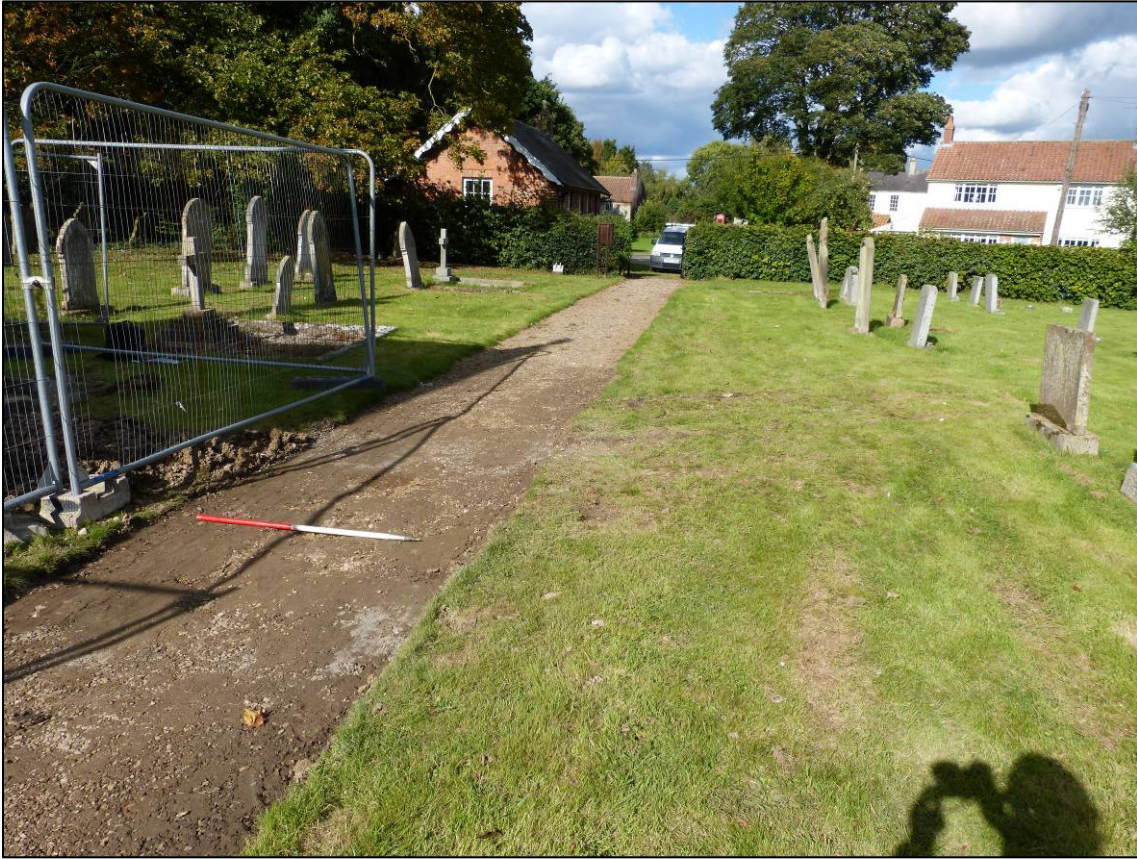
Plate 8: Position of new inspection chamber adjacent to footpath to the east of the church, looking N.
