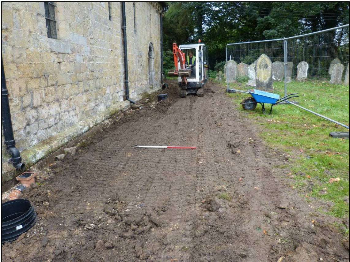
Plate 7: Phase 3 re-profiling work along the north wall of the church, after completion of drainage excavations, looking W.
