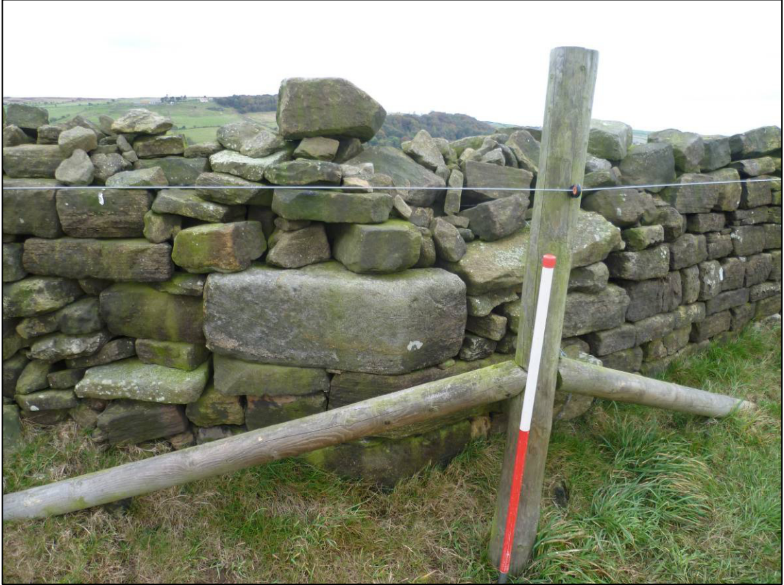
Plate 7: Angled quoins at change of angle, between crosses 27 and 28, south side, prior to repair (photo 1/295).
