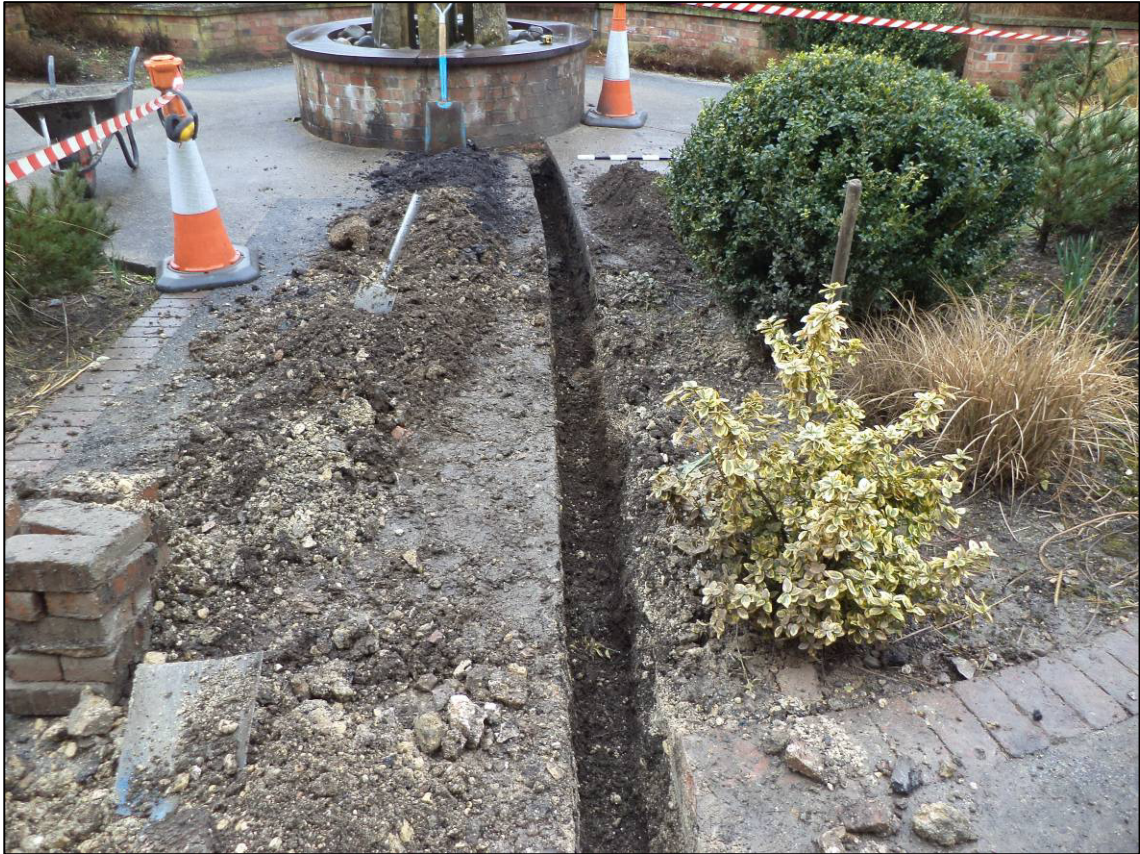
Plate 1: General view of excavated longer trench arm, looking NW towards water feature.
