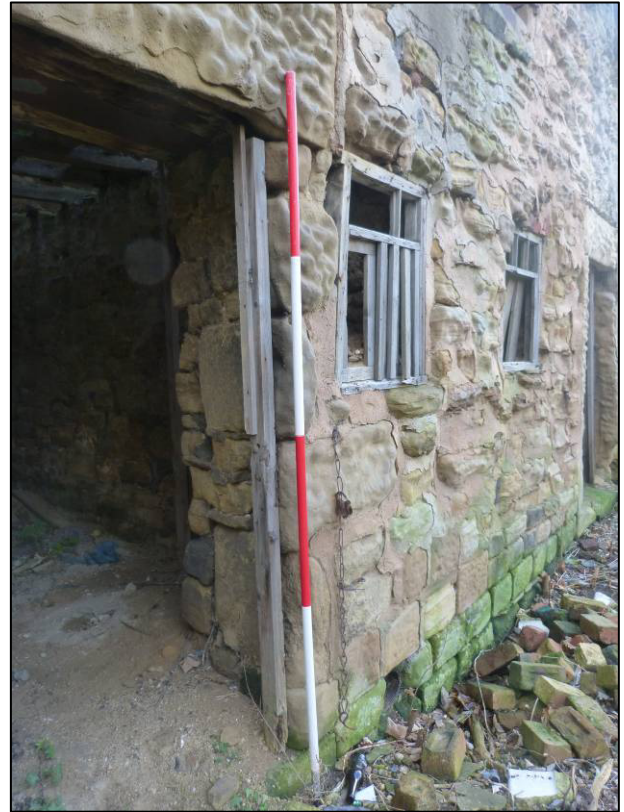
Plate 7: East range, north part, west elevation, doorway to north cell, looking SE (photo 1/364).
