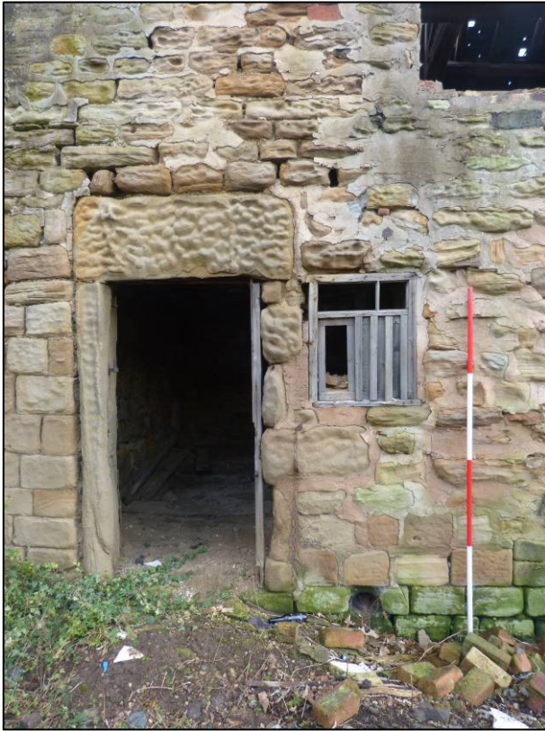
Plate 6: East range, north part, west elevation, doorway and window to north cell, looking E (photo 1/359).
