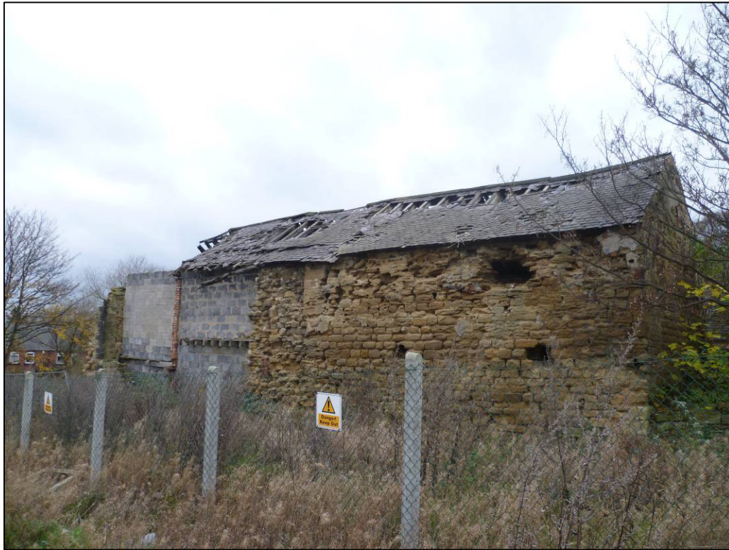
Plate 3: East side of north-south agricultural range, showing collapsing roof and recent repairs, looking SW.
