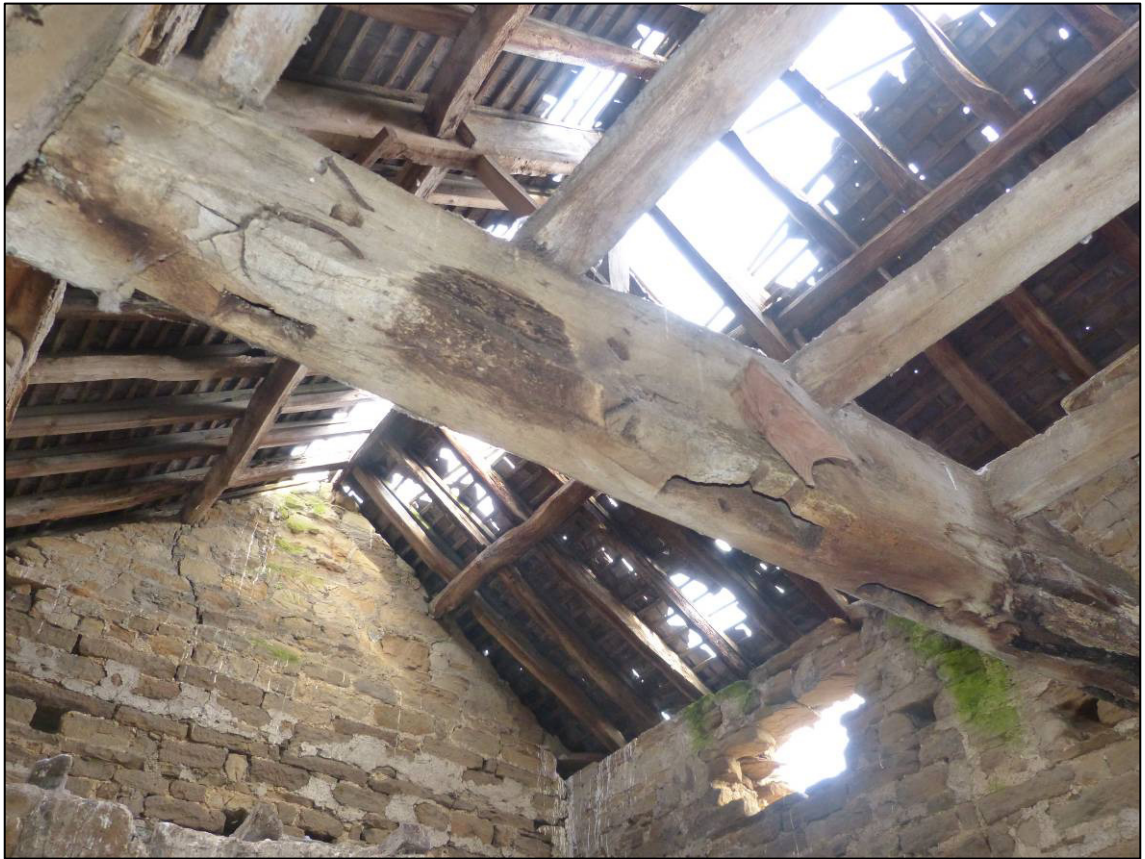
Plate 10: East range, north part, re-used tie-beam in south cell, looking NE (photo 1/385).
