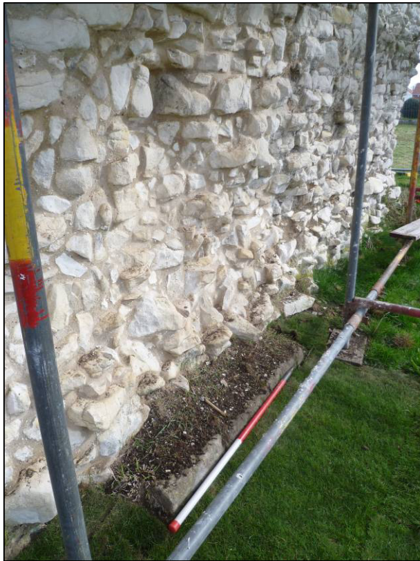
Plate 29: Castle (Site 6G), south external elevation, exposed plinth at base of wall with area of returfing, looking NE (photo 5/832).
