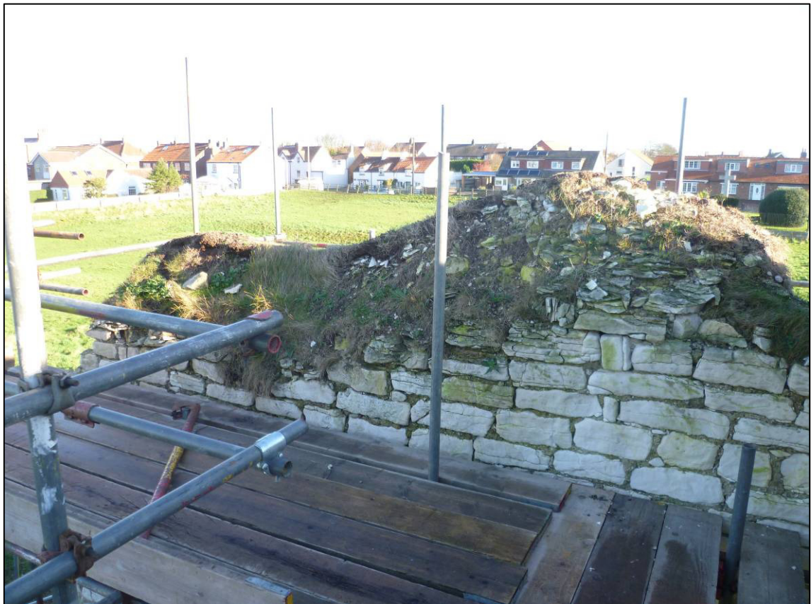
Plate 40: Castle (Site 6G), east internal wall top prior to clearance, looking SE (photo 3/301).
