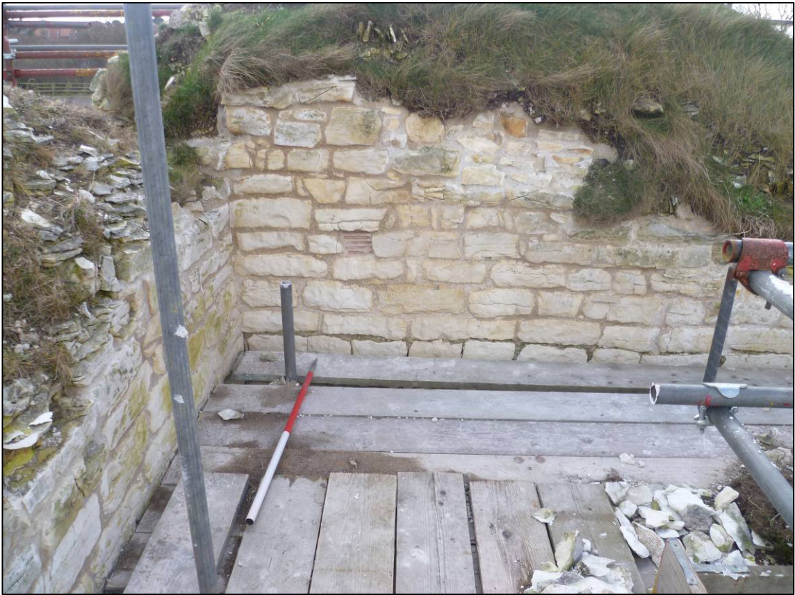
Plate 41: Castle (Site 6G), south internal wall top, east end, after repointing, looking S (photo 4/772).
