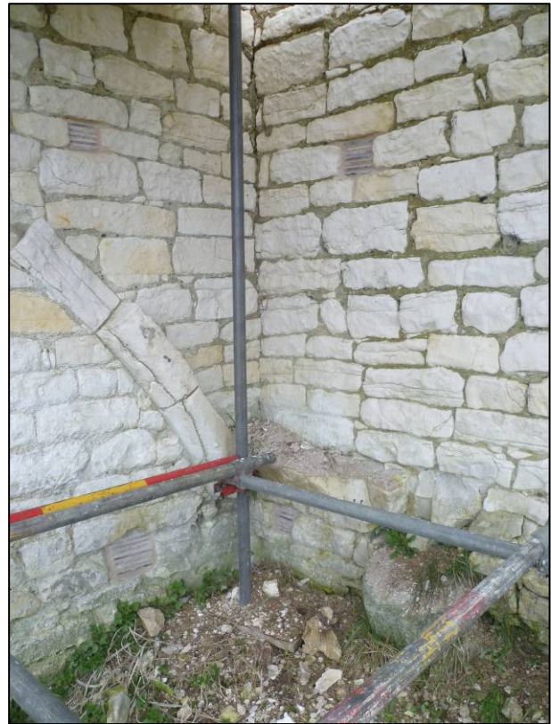
Plate 35: Castle (Site 6G), internal south-east corner after repair, showing springer for vault, looking SE (photo 4/797).
