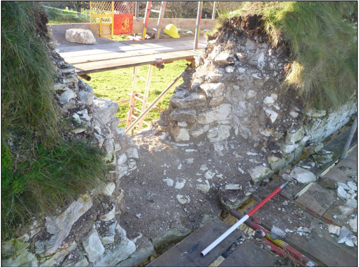
Plate 36: Castle (Site 6G), south internal wall top, window after clearance, looking SW (photo 3/270).
