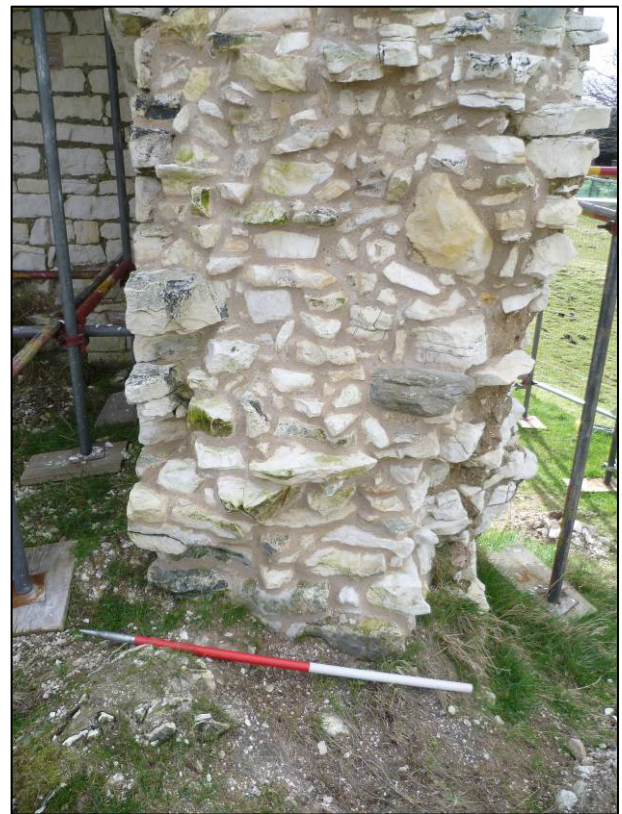
Plate 27: Castle (Site 6G), north end of west wall, window opening, after repair, looking S (photo 4/798).
