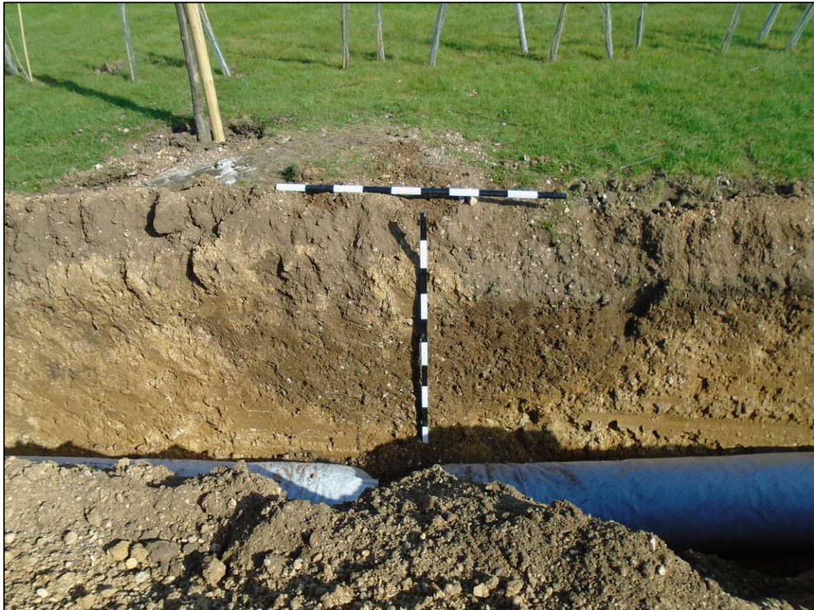
Plate 15: Ditch [127] in soakaway drain along east side of access road, looking E.
