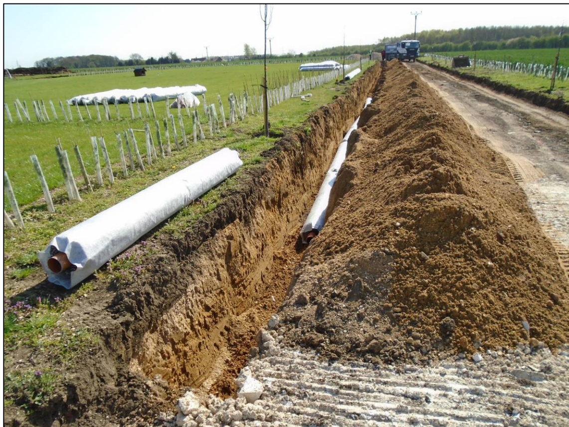
Plate 14: North end of soakaway drain along east side of access road after excavation, looking SW.
