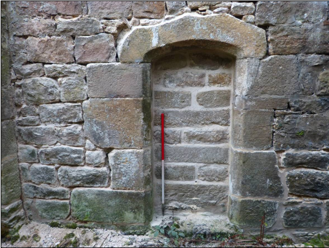
Plate 3: North side of doorway in north chapel wall, prior to unblocking, looking S (photo 1/809).
