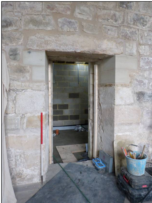
Plate 12: South face of unblocked and raised doorway in north wall of chapel, looking N (photo 5/269).
