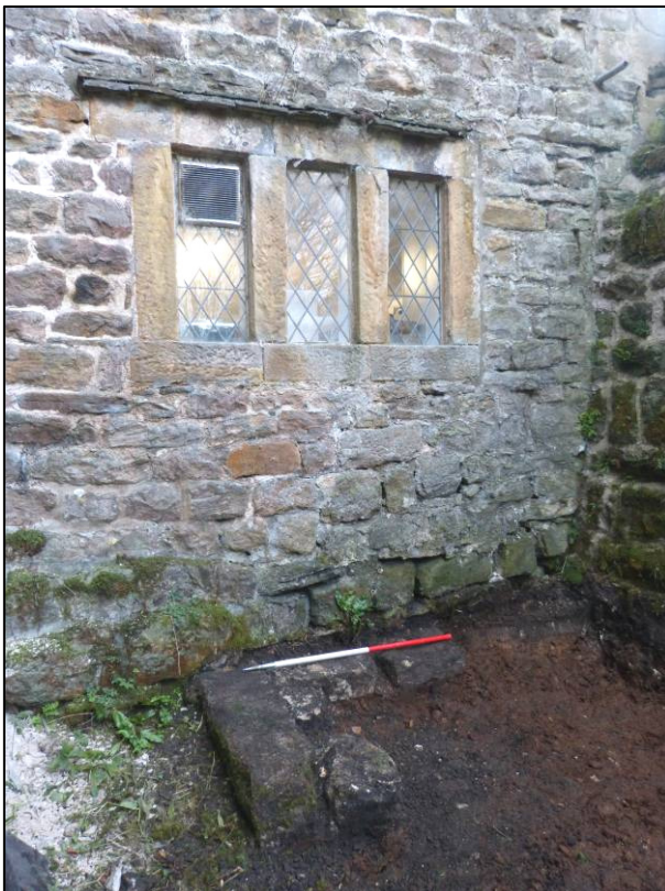
Plate 9: Footings at base of domestic range's east elevation in sunken area, looking NW (photo 1/819).
