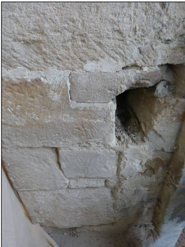
Plate 15: Draw bar recess and adjacent mason's marks in west jamb of doorway in north wall of chapel, revealed after unblocking, looking W (photo 4/019).
