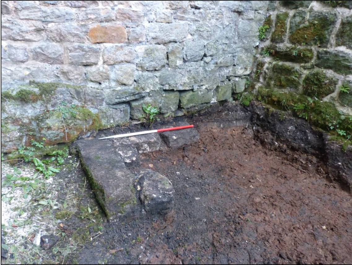
Plate 8: Footings at base of domestic range's east elevation in sunken area, looking NW (photo 1/820).
