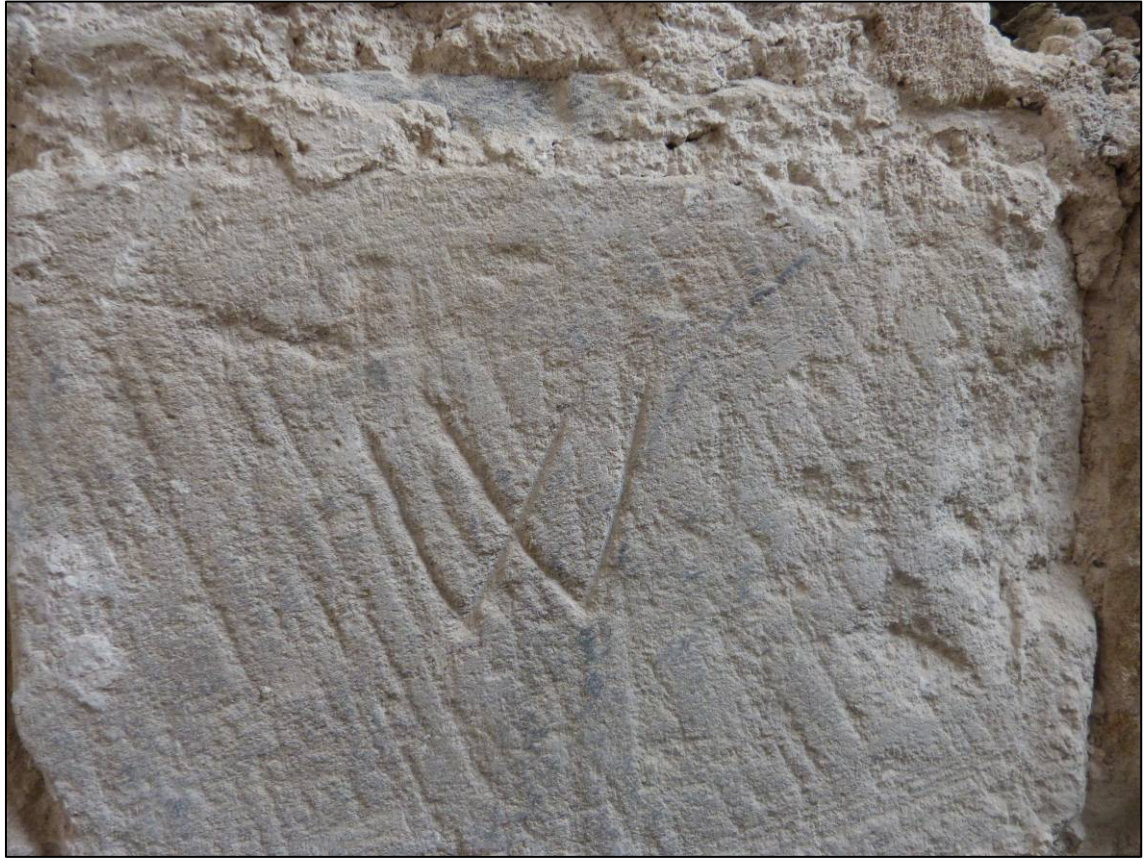
Plate 14: Mason's mark in west jamb of doorway in north wall of chapel, revealed after unblocking, looking W (photo 4/021).
