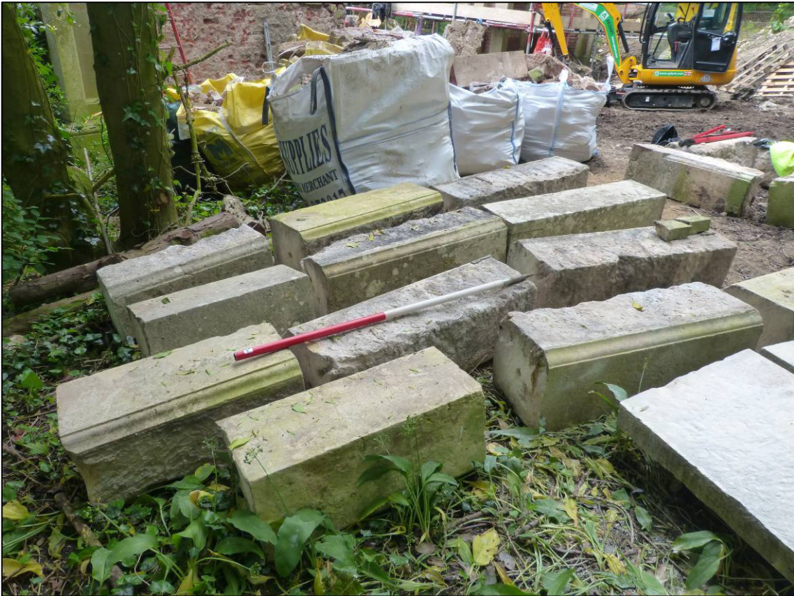
Plate 15: Dismantled dressings of south gate pier and wing wall, awaiting reconstruction (photo 2/086).
