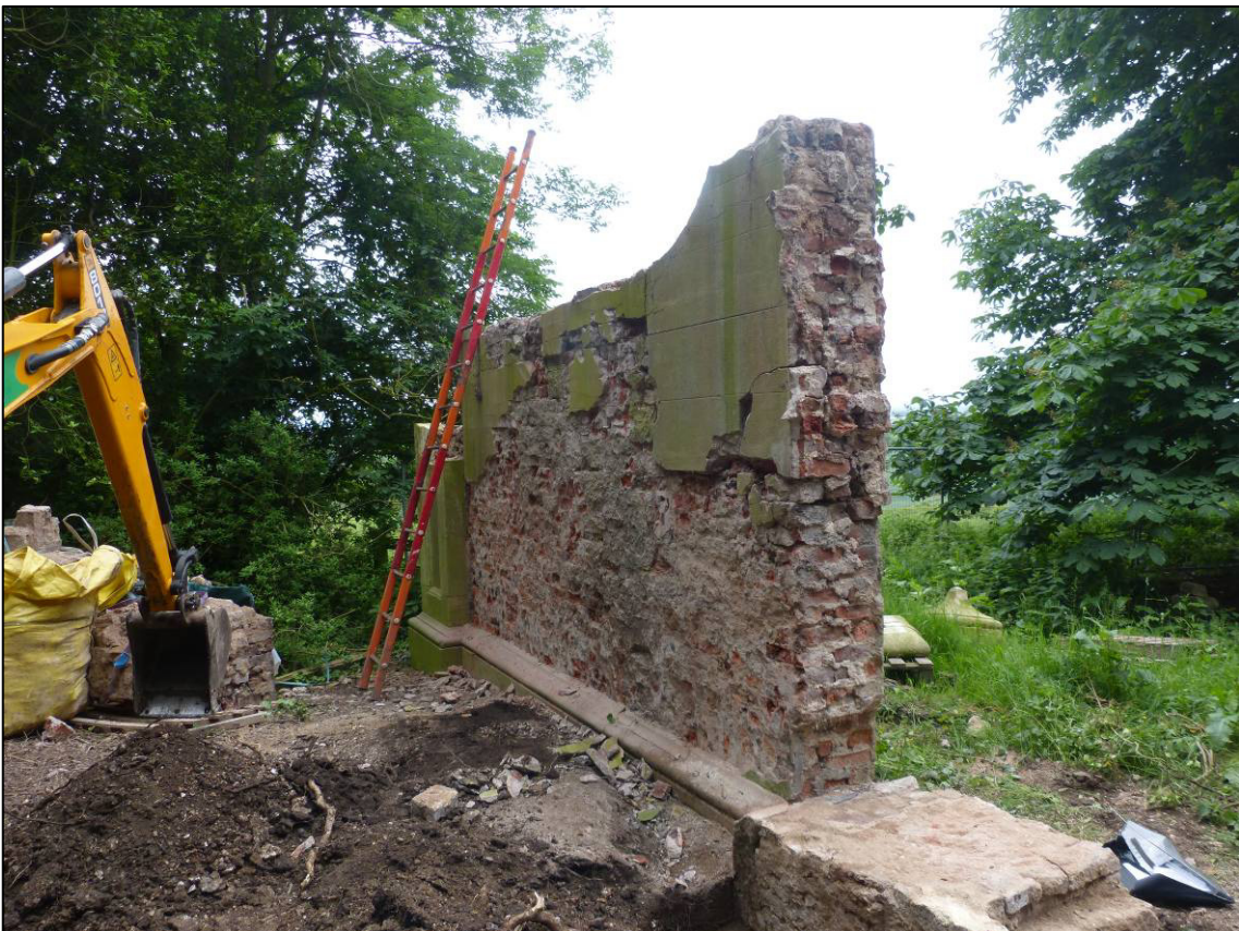
Plate 14: View of south wing wall after demolition of Pier 3, looking S (photo 2/063).
