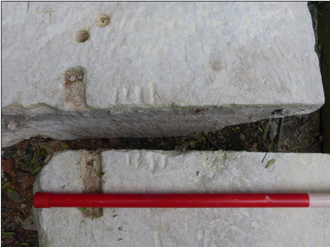
Plate 16: Dismantled south gate pier cap (Pier 3), showing assembly marks to underside (photo 2/065).
