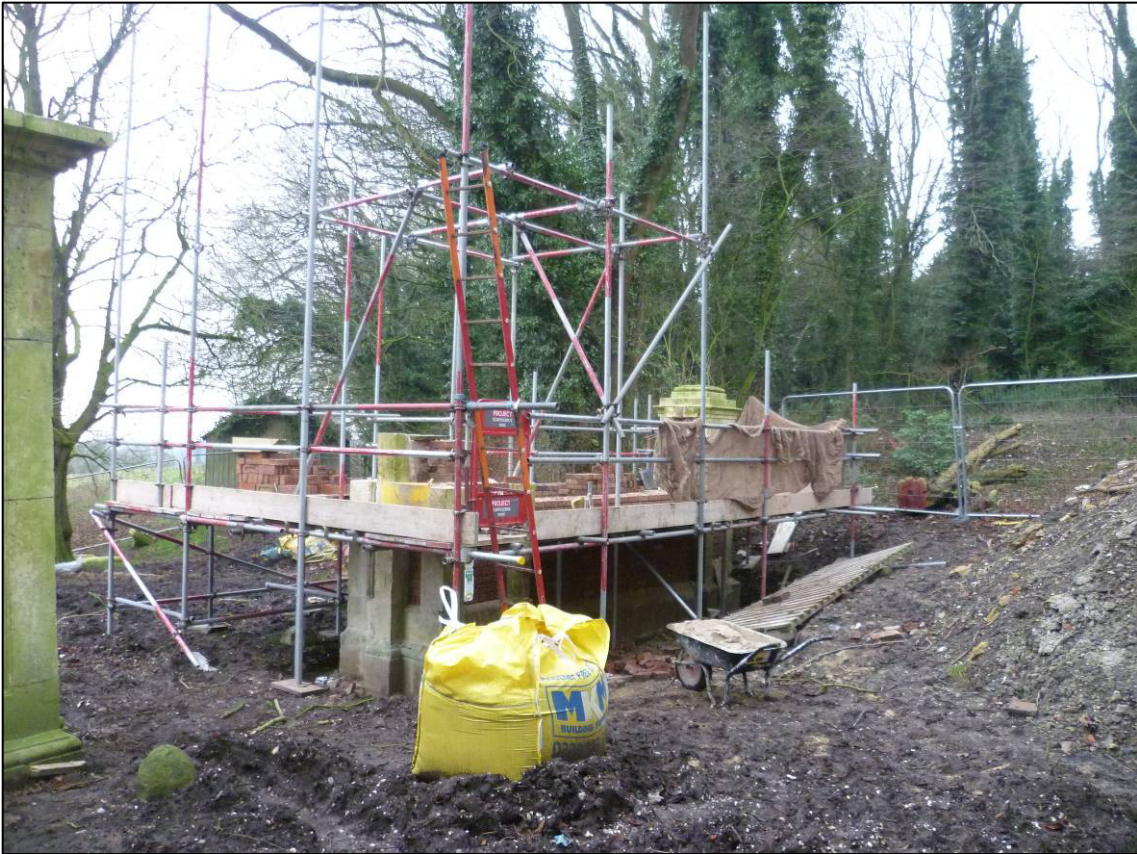
Plate 11: Restoration works underway on north side of gateway (Piers 1 and 2), looking W (photo 1/449).
