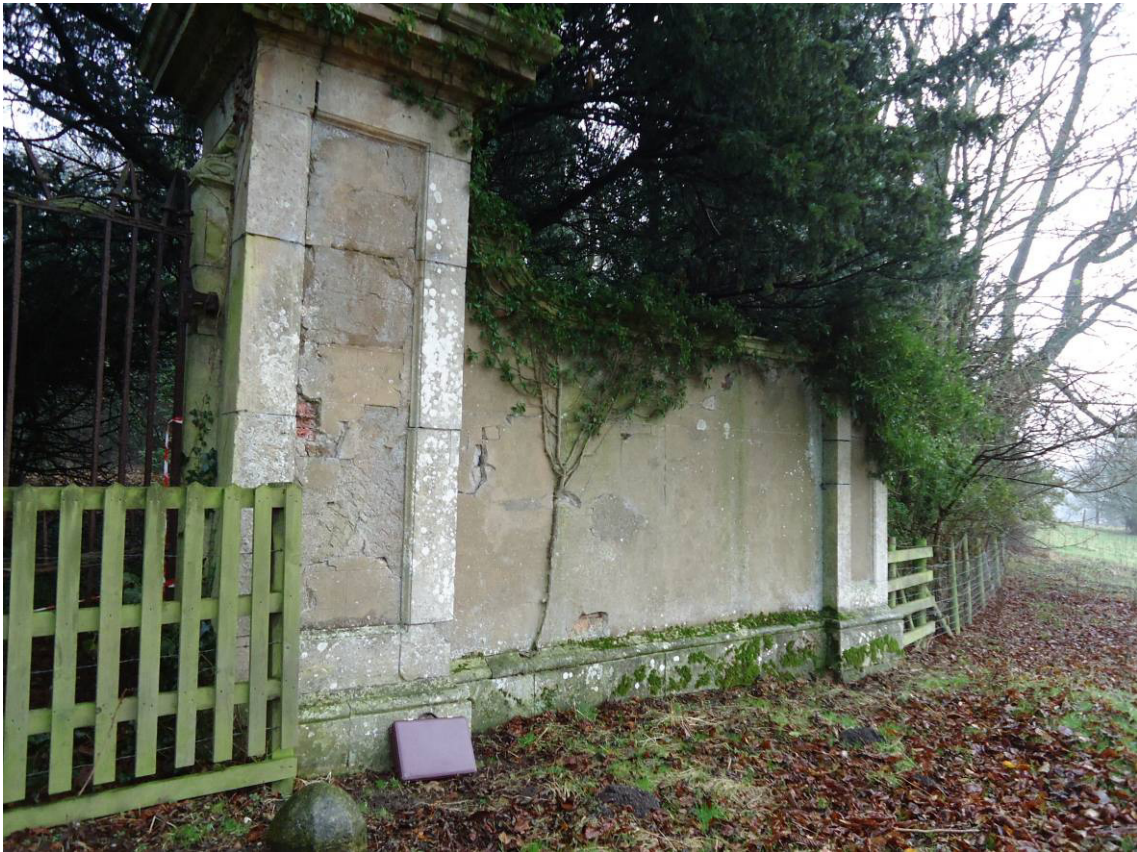
Plate 3: South side of gateway (Piers 3 and 4), west elevation, prior to restoration, looking E (December 2016) (photo courtesy Peter Pace).
