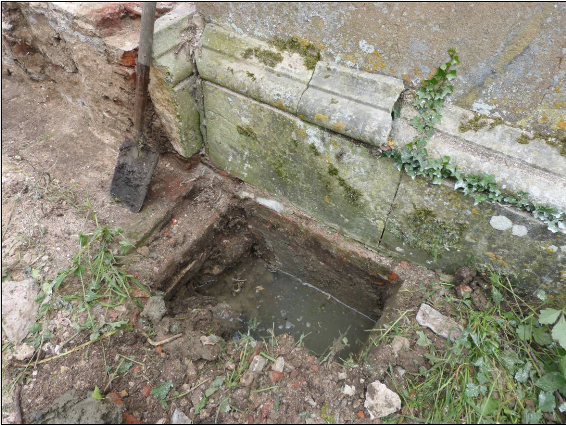
Plate 13: Footings of west side of south wing wall, and butting plinths to Pier 3 and wing wall, looking NE (photo 2/069).
