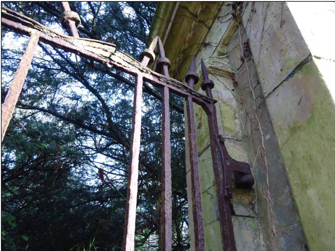
Plate 10: Detail of gate and damaged gate on Pier 3, prior to restoration, looking E (December 2016) (photo courtesy Peter Pace).
