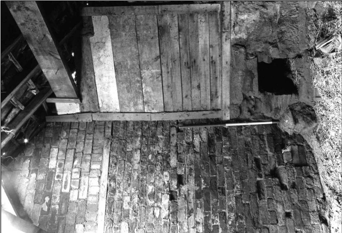
Plate 29: North cattle shade range, E cell, structure in NW corner, looking NW (photo 6/1) (top to left).
