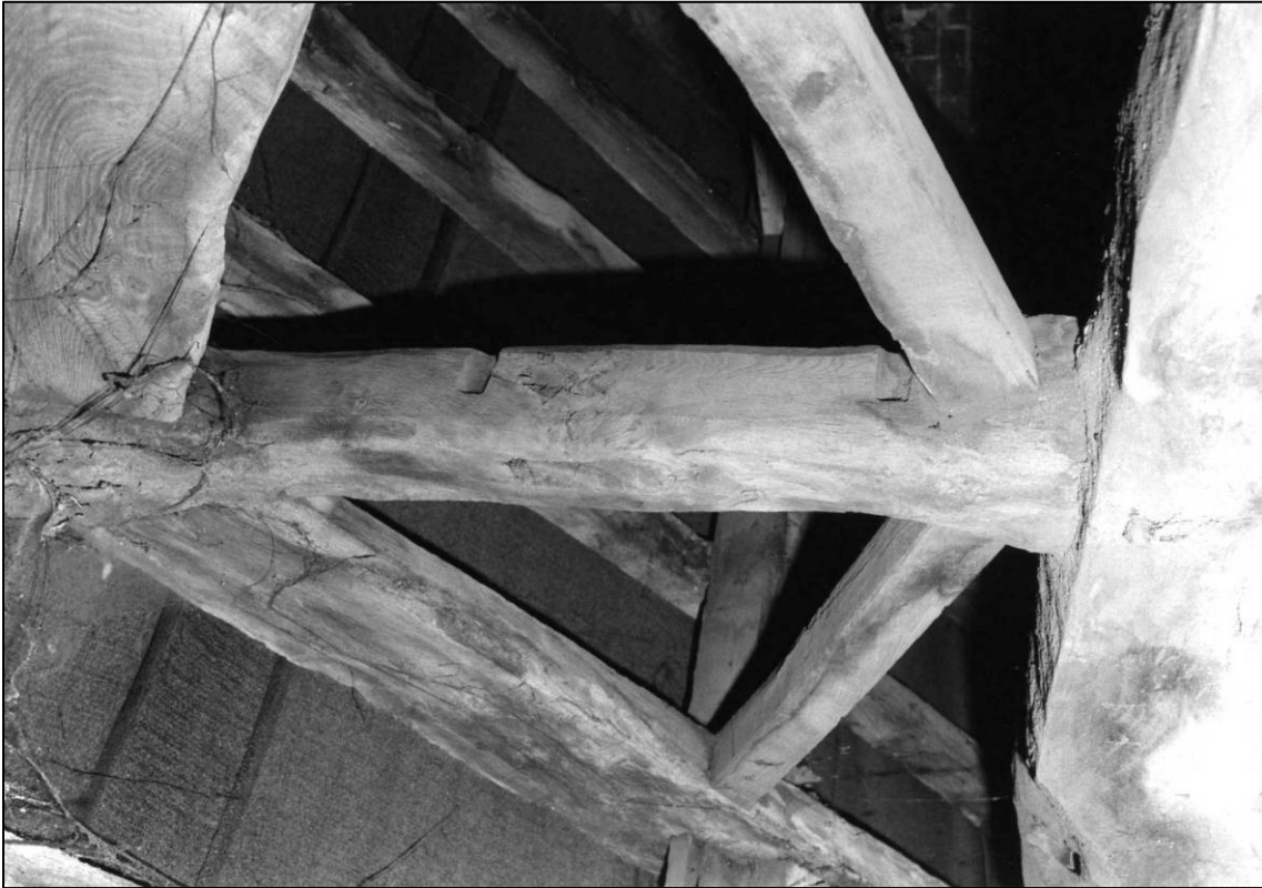
Plate 93: Barn Cottage range, N part, above central first floor room (Room 5), N face of S truss, looking SE (photo 12/5) (top to left).
