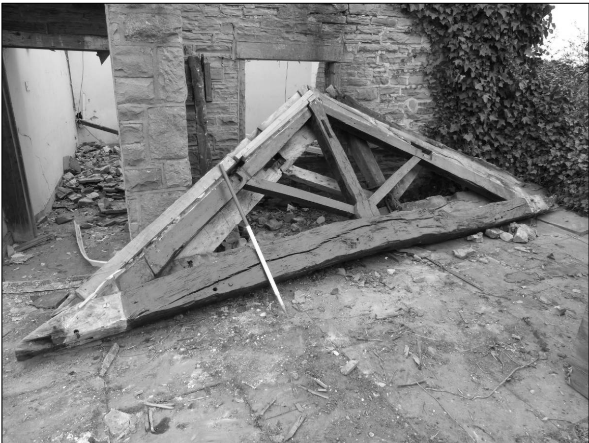
Plate 110: Barn Cottage range, S part, north and south roof trusses after removal (photo 10/955).
