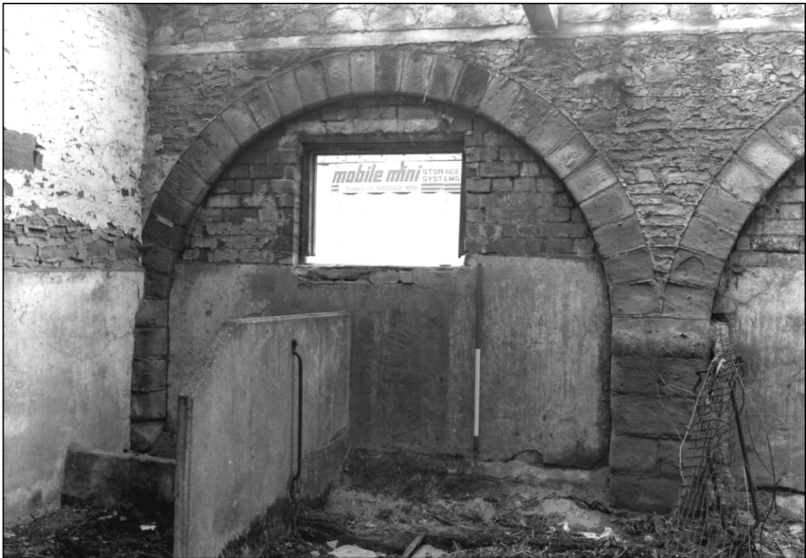
Plate 20: West coach house and stable range, N cell, blocked carriage opening, looking W (photo 2/15).
