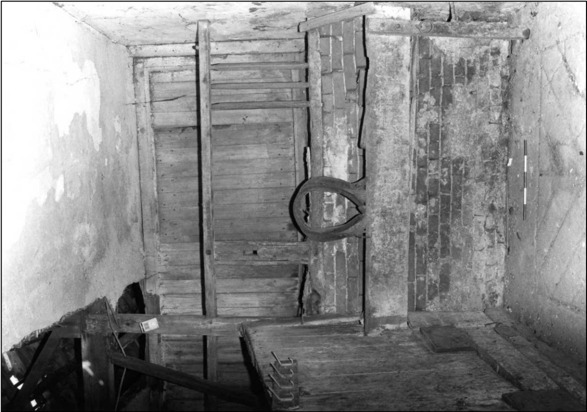
Plate 13: West coach house and stable range, S cell, E stall, looking N (photo 1/18) (top to left).
