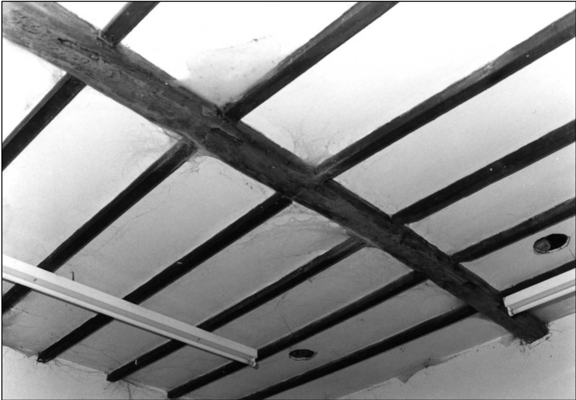
Plate 97: Barn Cottage range, S part, S ground floor room (Room 7), ceiling, looking SE (photo 4/6).
