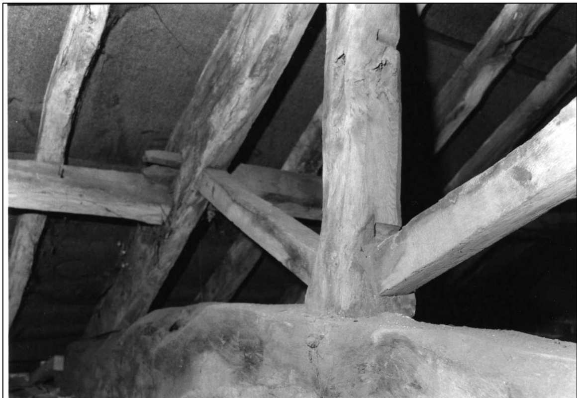
Plate 92: Barn Cottage range, N part, above central first floor room (Room 5), N face of S roof truss, looking SE (photo 12/4).
