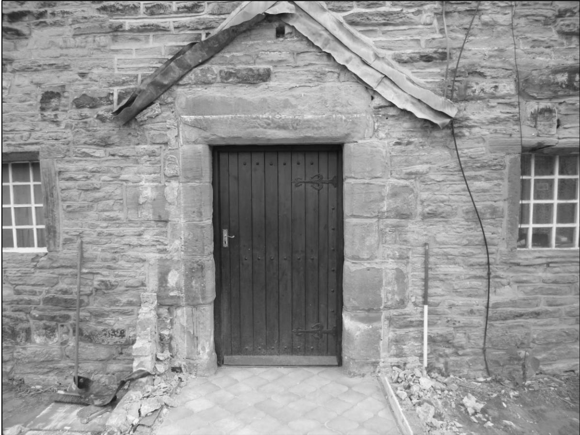
Plate 69: Barn Cottage range, N part, W elevation, doorway after demolition of porch, looking SE (photo 9/98).
