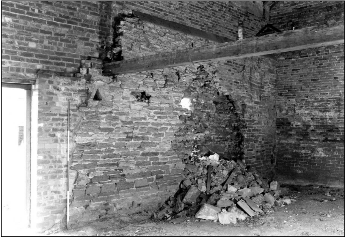
Plate 55: East barn range, interior, localised collapse in N end of W wall, looking NW (photo 5/5).
