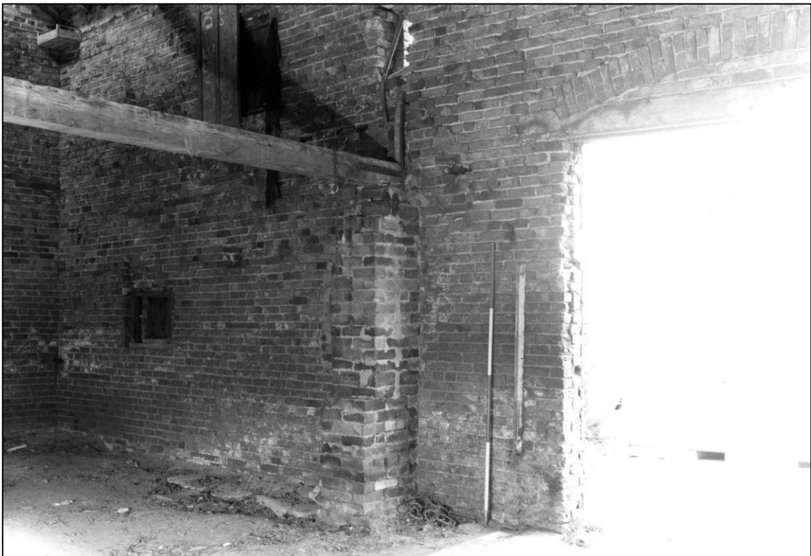
Plate 54: East barn range, interior, N end of E wall, looking NE (photo 5/7).
