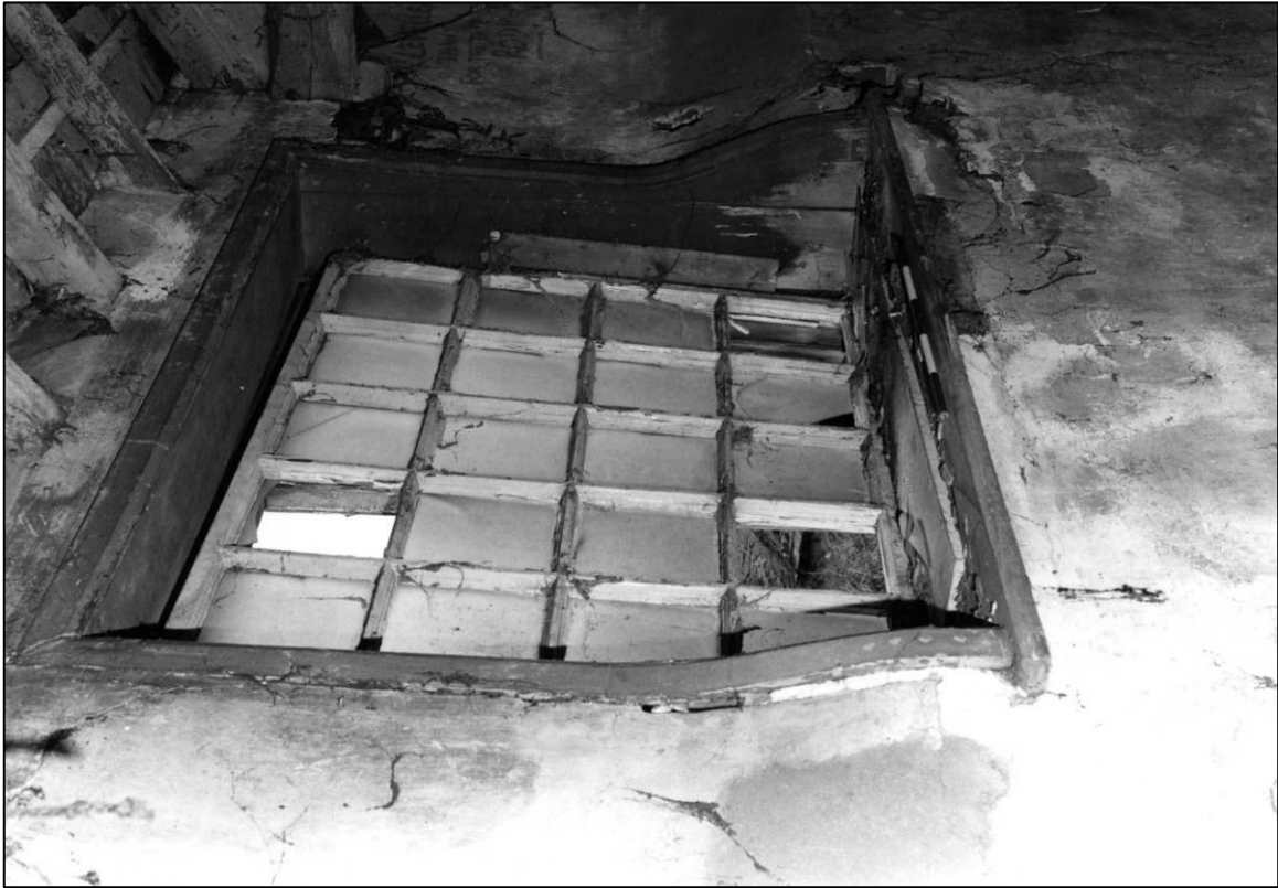
Plate 61: East barn range, S first floor cell, window in W wall, looking NW (photo 5/10) (top to left).
