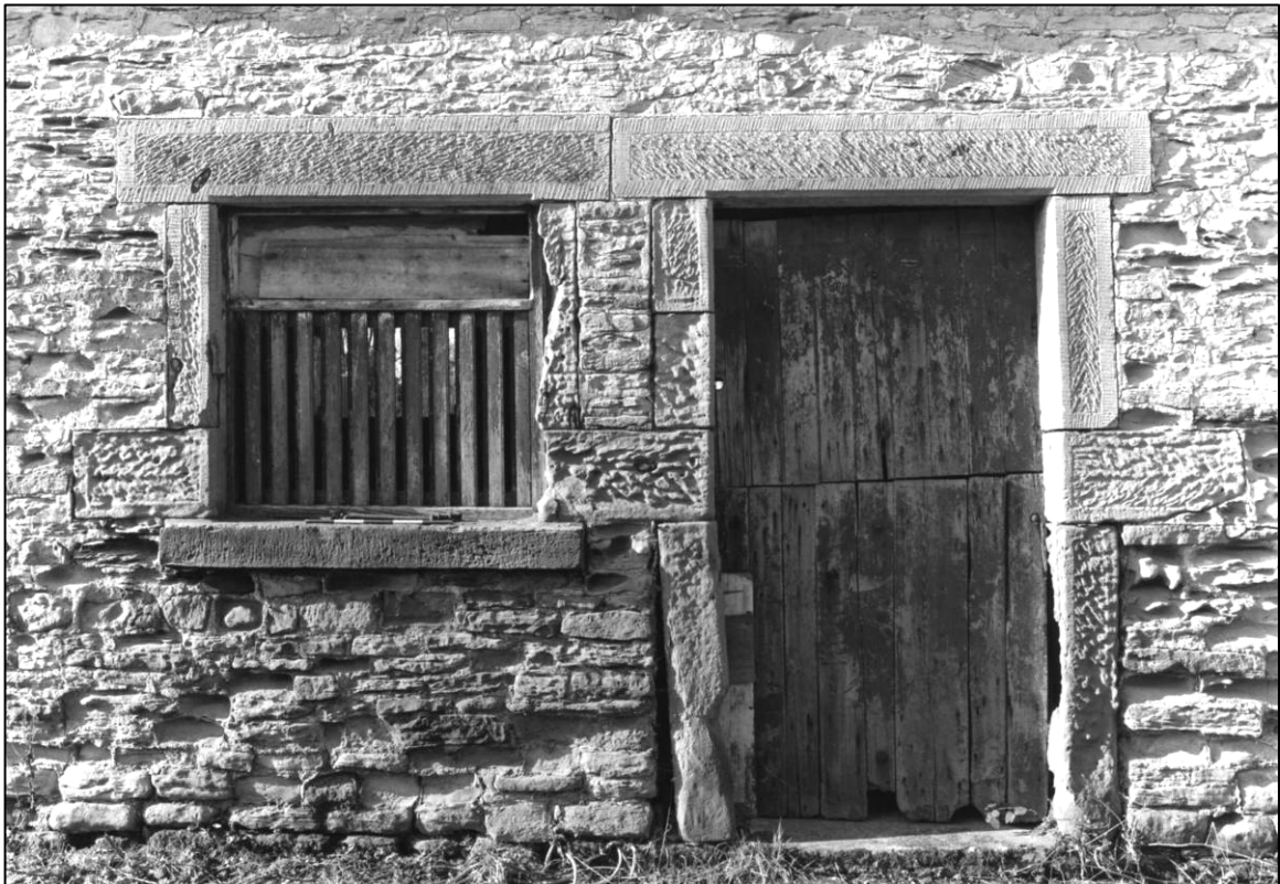
Plate 8: West coach house and stable range, E elevation, detail of door and window dressings, looking W (photo 1/10).
