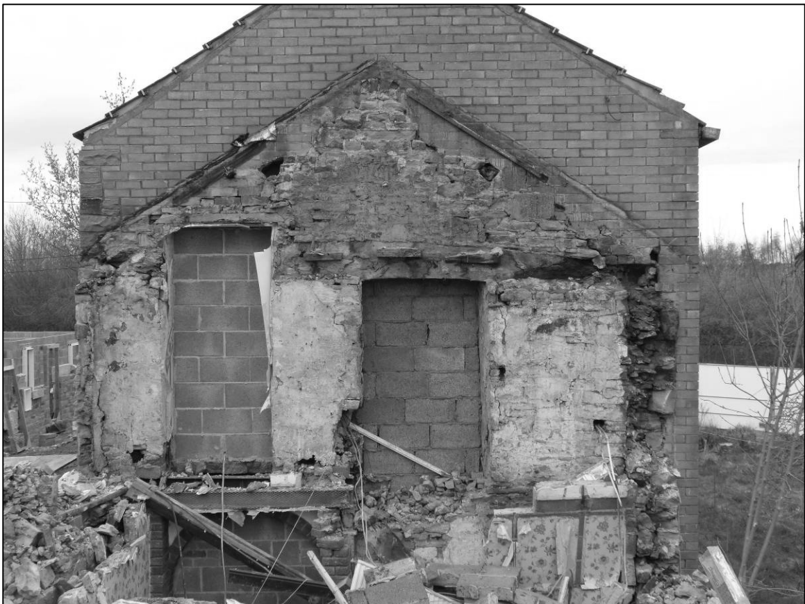
Plate 112: Barn Cottage range, S part after demolition, showing timber in wall and blocked doorway at first floor level (Room 9), looking N (photo 10/966).
