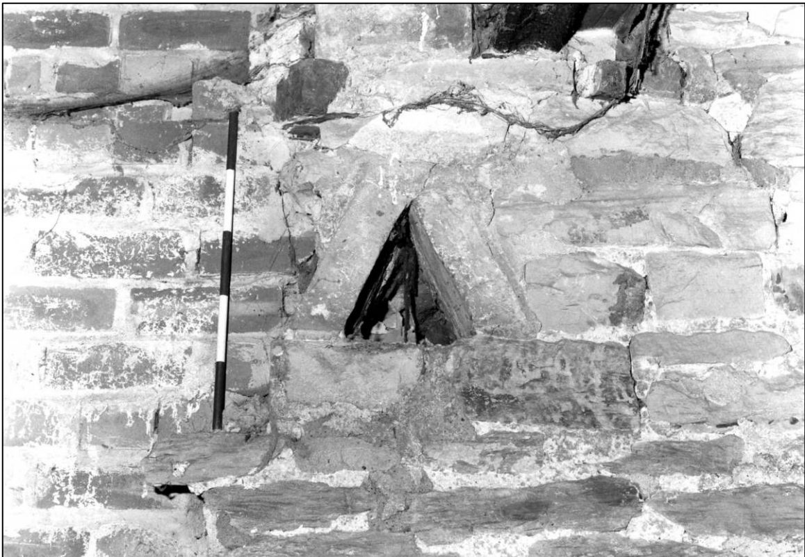
Plate 56: East barn range, W wall, triangular breather in W wall, looking W (photo 5/4).
