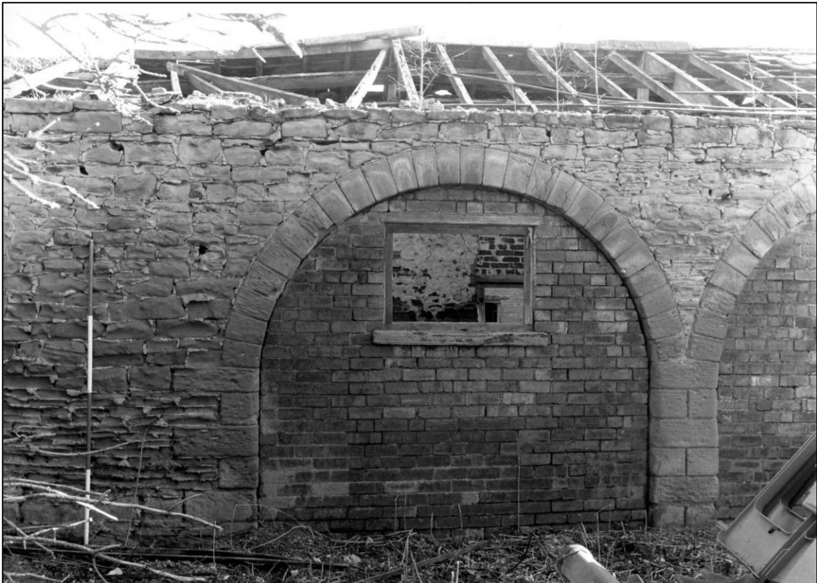
Plate 4: West coach house and stable range, W elevation, blocked carriage opening at N end, looking E (photo 1/1).
