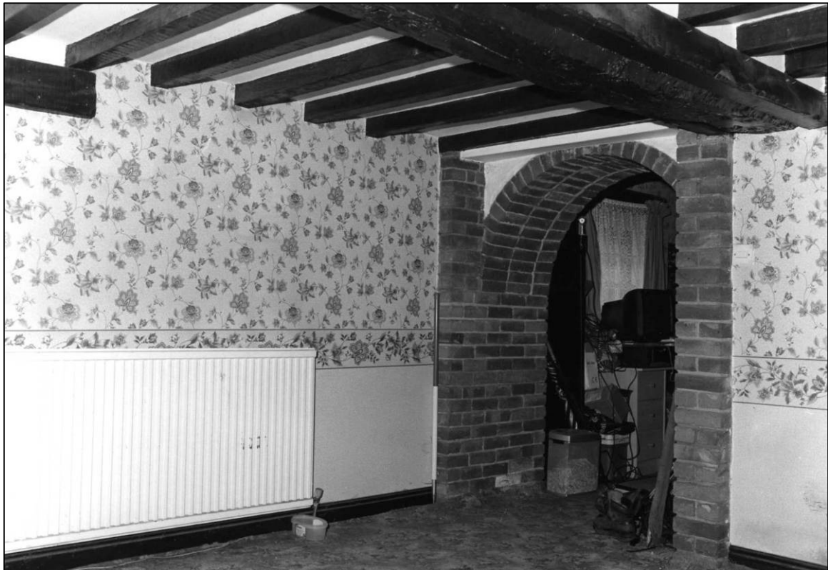
Plate 101: Barn Cottage range, S part, N ground floor room (Room 8), looking NW (photo 6/10).
