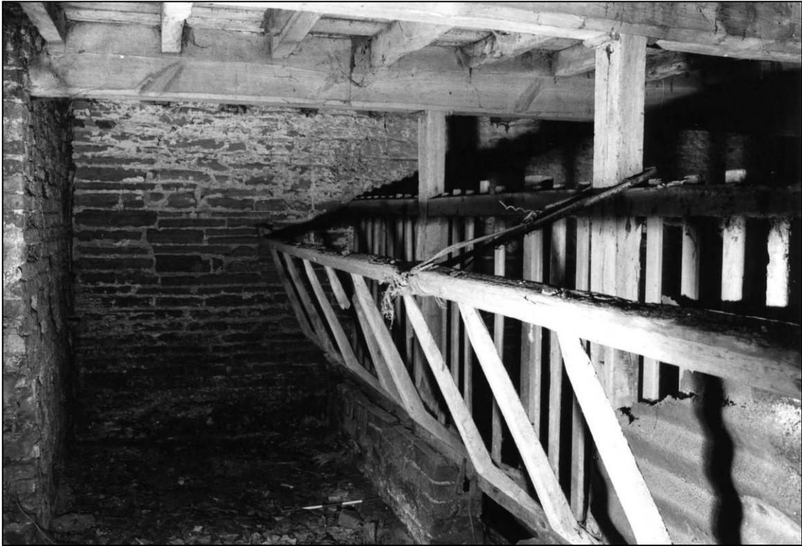
Plate 43: East barn range, S ground floor cell, hay rack, looking W (photo 4/11).
