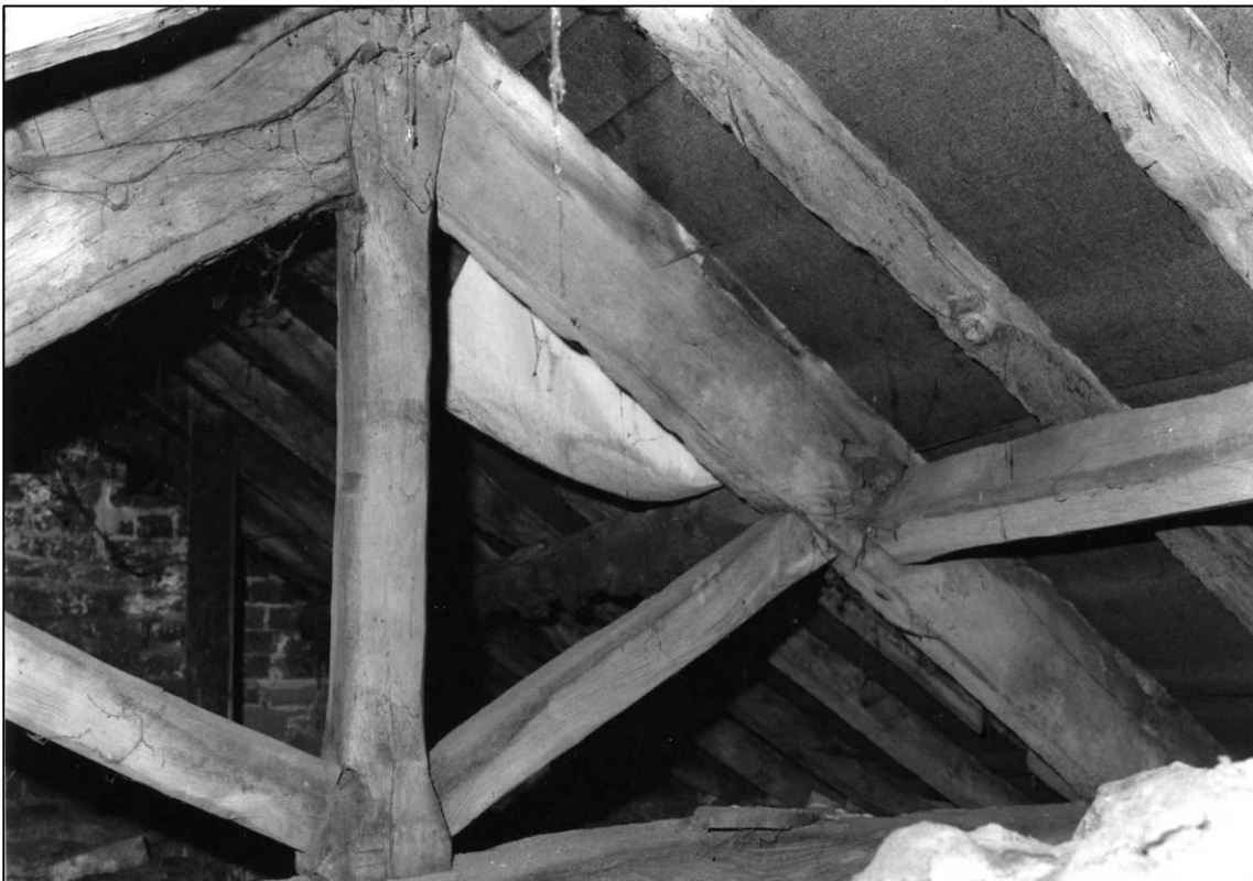
Plate 94: Barn Cottage range, N part, above N first floor room (Room 4), S face of N truss, looking NE (photo 12/7).
