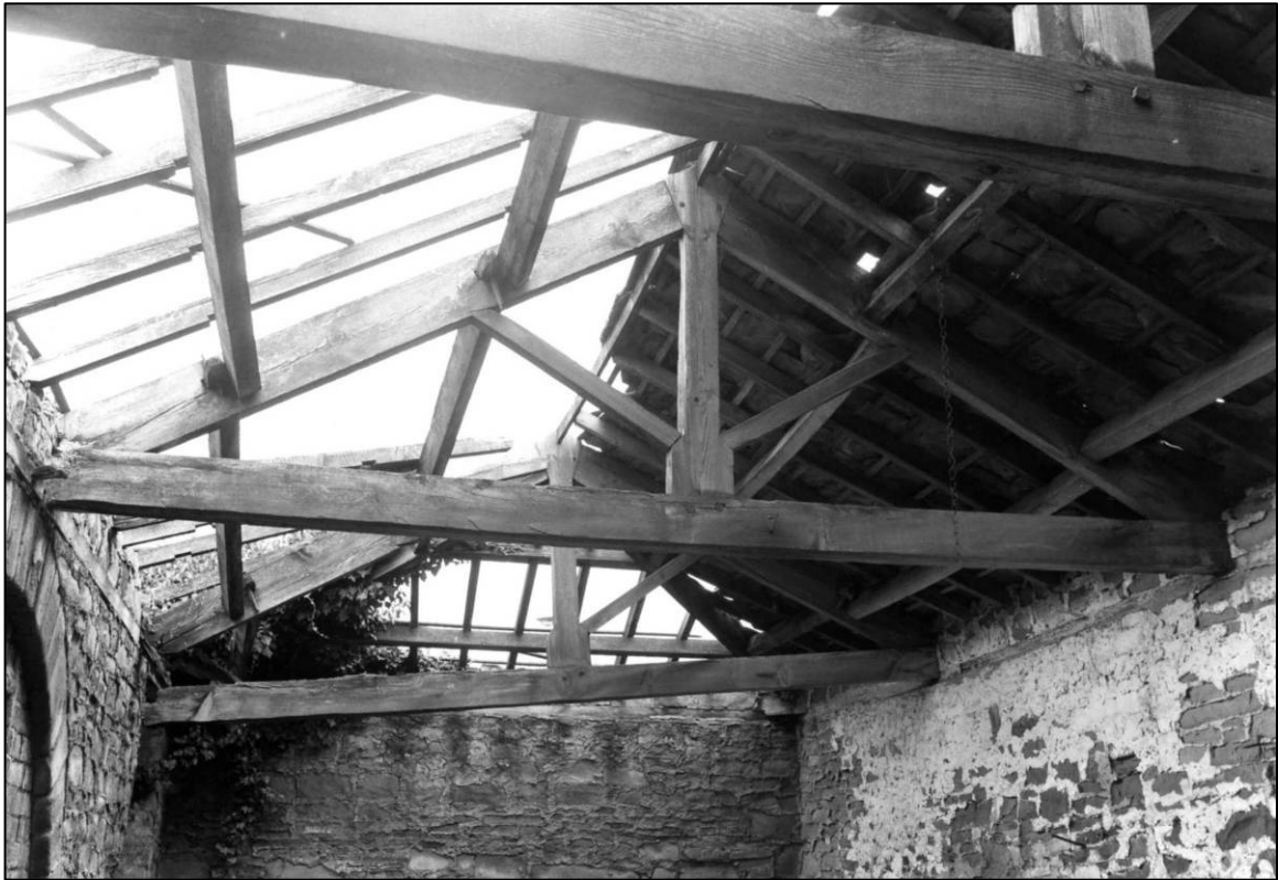
Plate 23: West coach house and stable range, N cell, roof trusses, looking N (photo 2/14).
