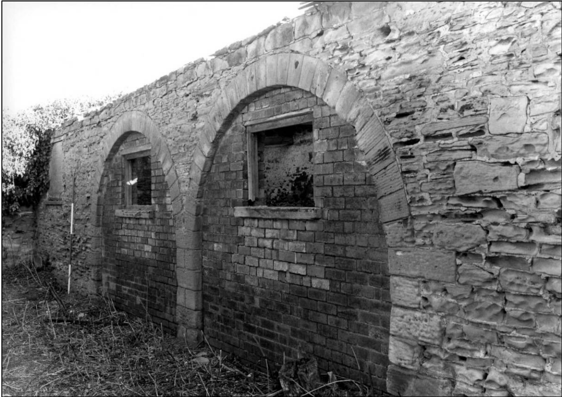
Plate 5: West coach house and stable range, W elevation, blocked carriage openings at N end, looking NE (photo 1/3).
