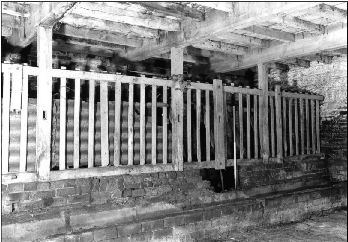
Plate 44: East barn range, S ground floor cell, hay rack, looking SW (photo 4/13).
