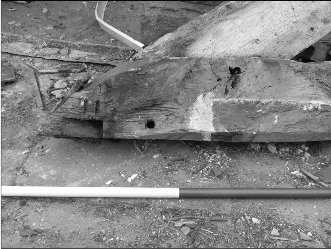
Plate 111: Barn Cottage range, S part, roof truss after removal, detail of carpenter's marks (photo 10/959).
