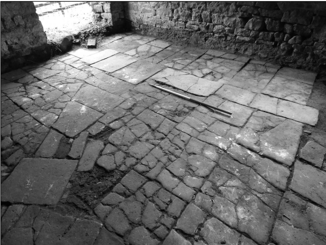
Plate 20: Flagstone floor in east side of furnace room, after clearance and cleaning, showing east end of covered culvert (D) and angled channel (F), looking SE (photo 4/158).
