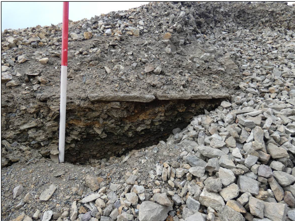
Plate 28: Exposed flagstones and waste material below main revetment wall (K), looking S (photo 2/374).
