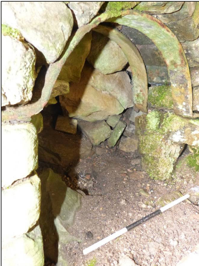
Plate 14: East draw arch, iron bands to draw hole, looking NW (photo 1/907).
