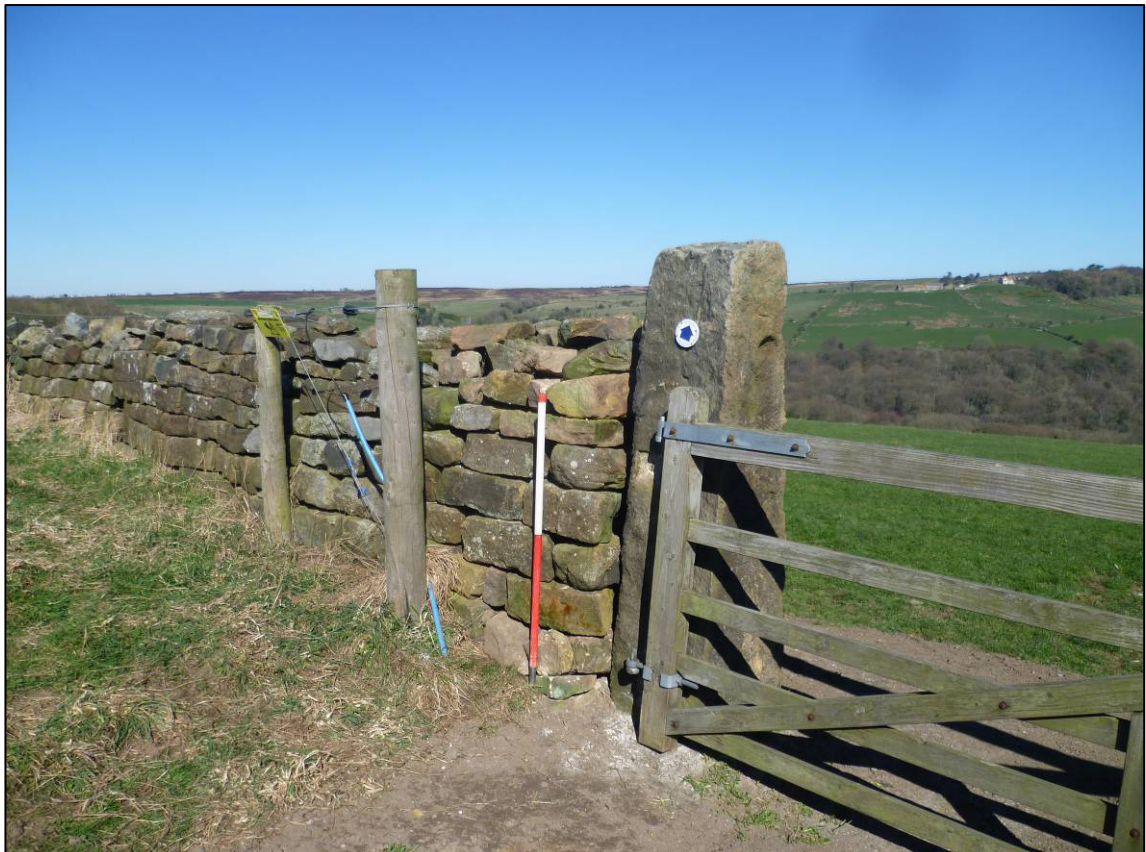
Plate 15: Repositioned western gateway, rebuilt wall end and re-hung gate, looking NW (photo 2/346).
